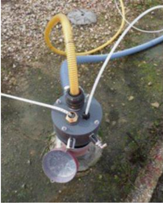
Image 5: Example showing similar temporary pipe arrangements that will be connected to each injection well during injection trials (approximately 21 well locations for up to 12 weeks)
