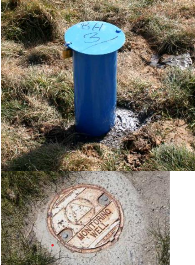
Image 2a and 2b: Indicative images of finished boreholes (top hat cover and flush cover)
