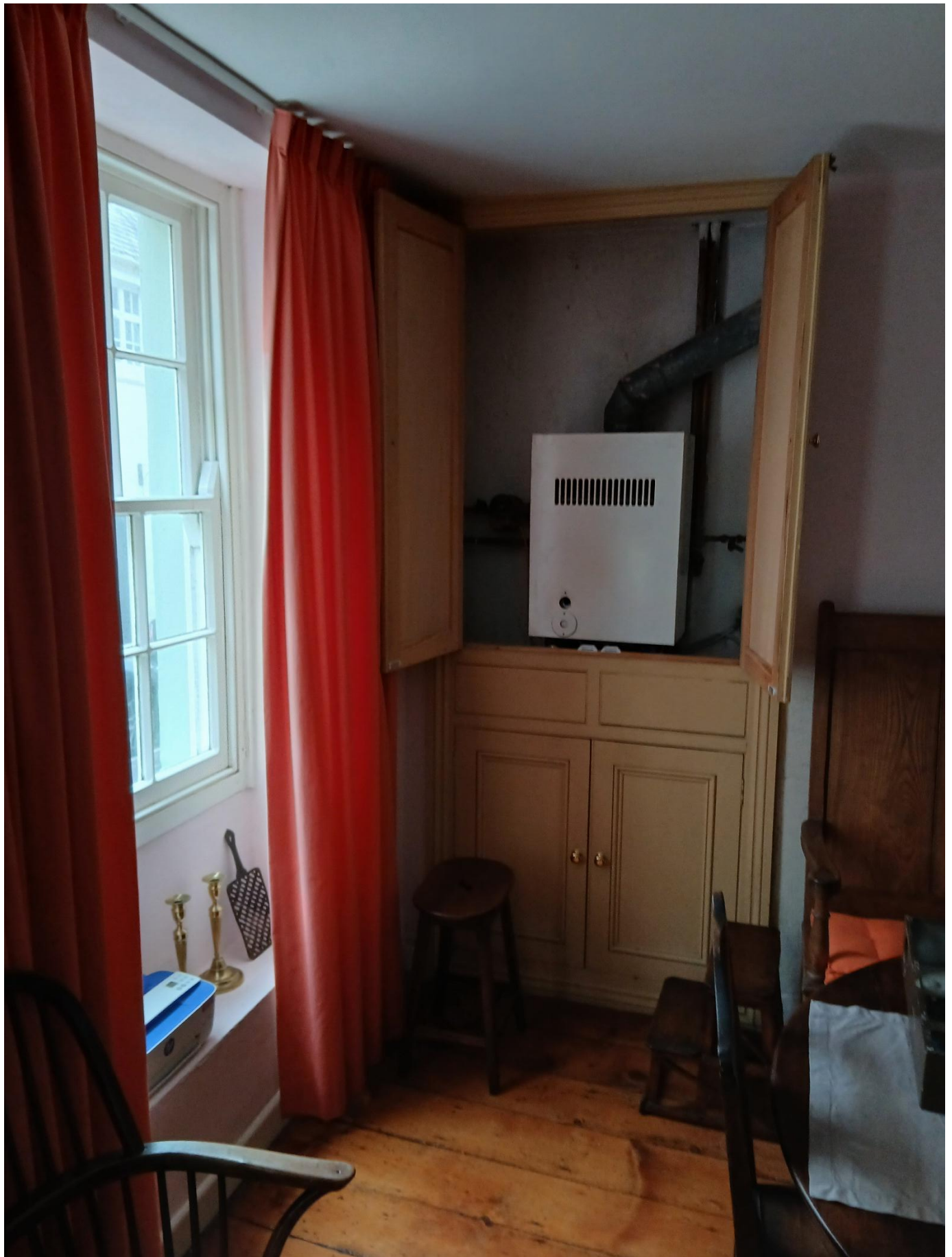
Current boiler location
