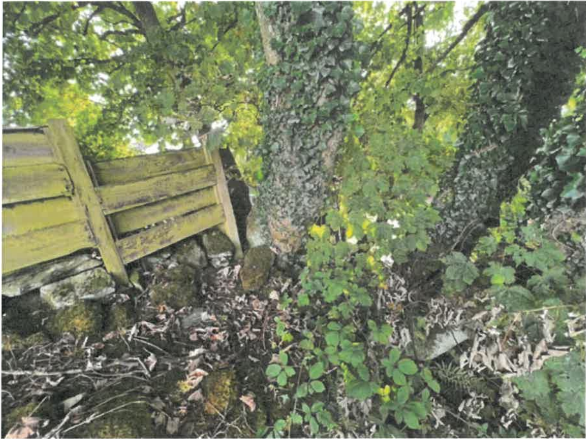
Tree from adjacent property growing through wall.
