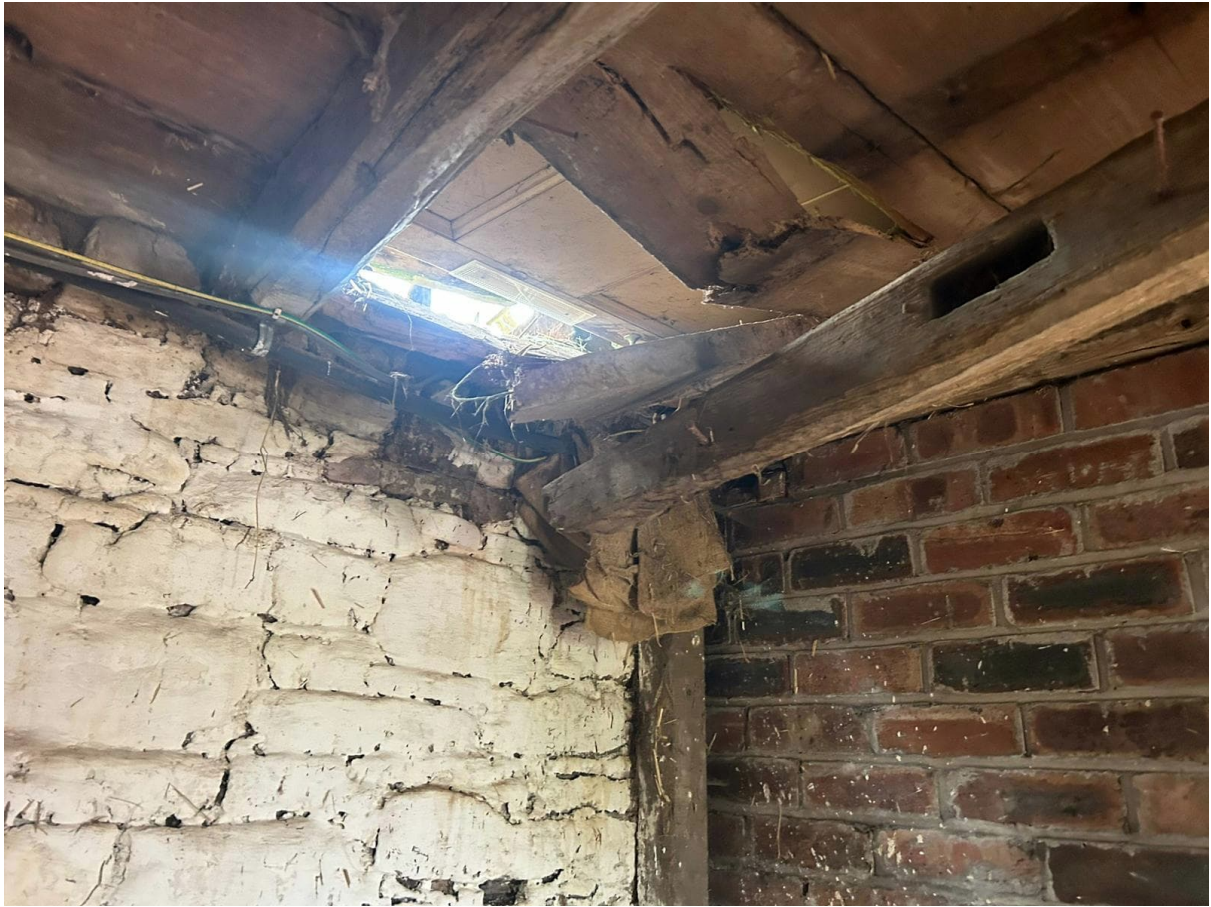
Fig 3 Photograph from underside of first floor showing collapsed section over store room.
