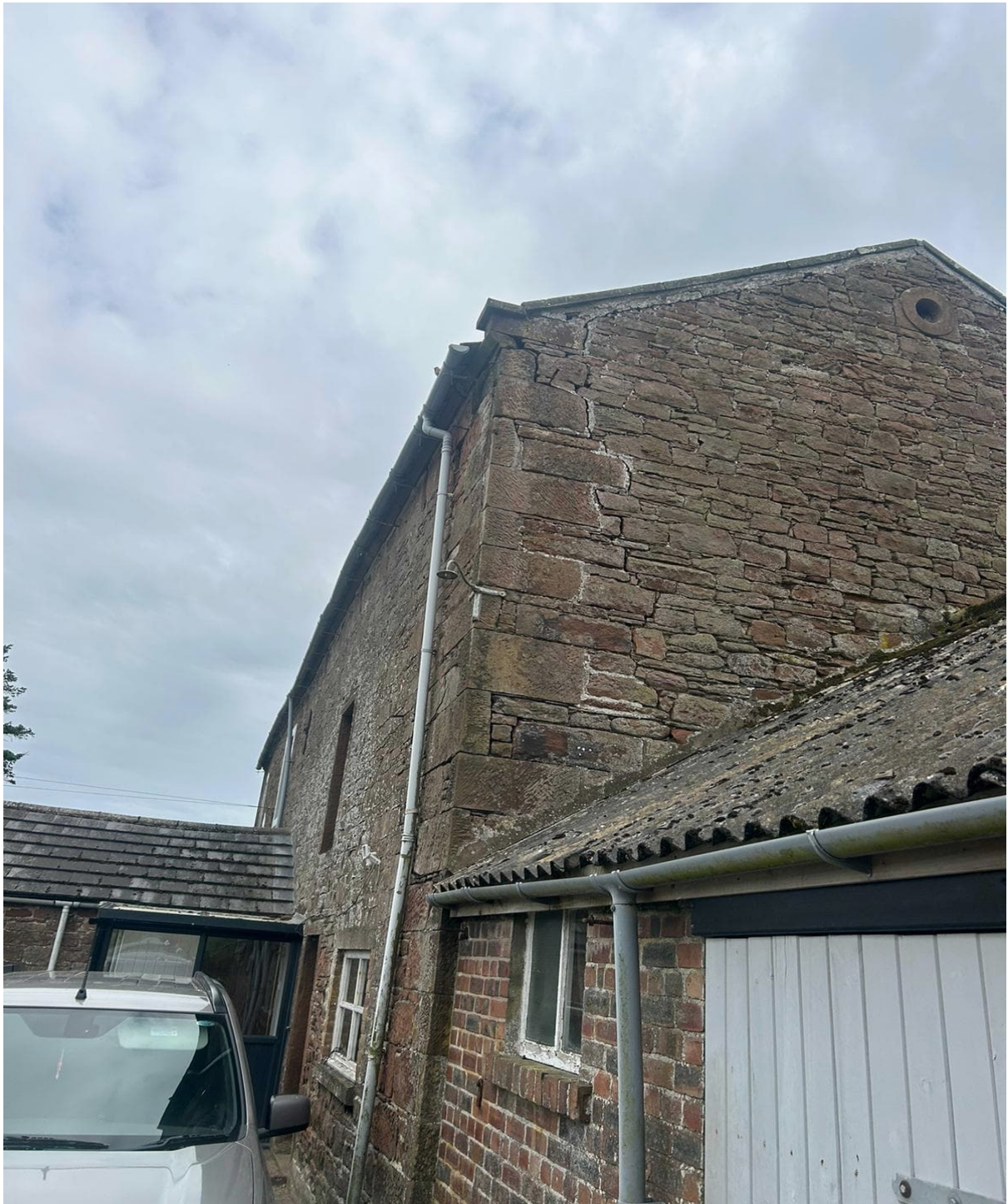
Fig 5 Photograph of vertical cracking to front side of gable end wall
