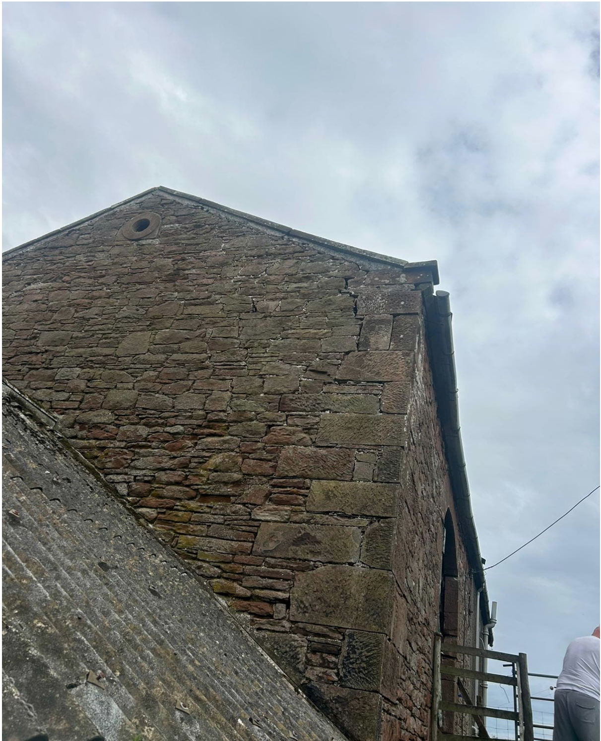
Fig 6 Photograph of vertical cracking to rear side of gable end wall
