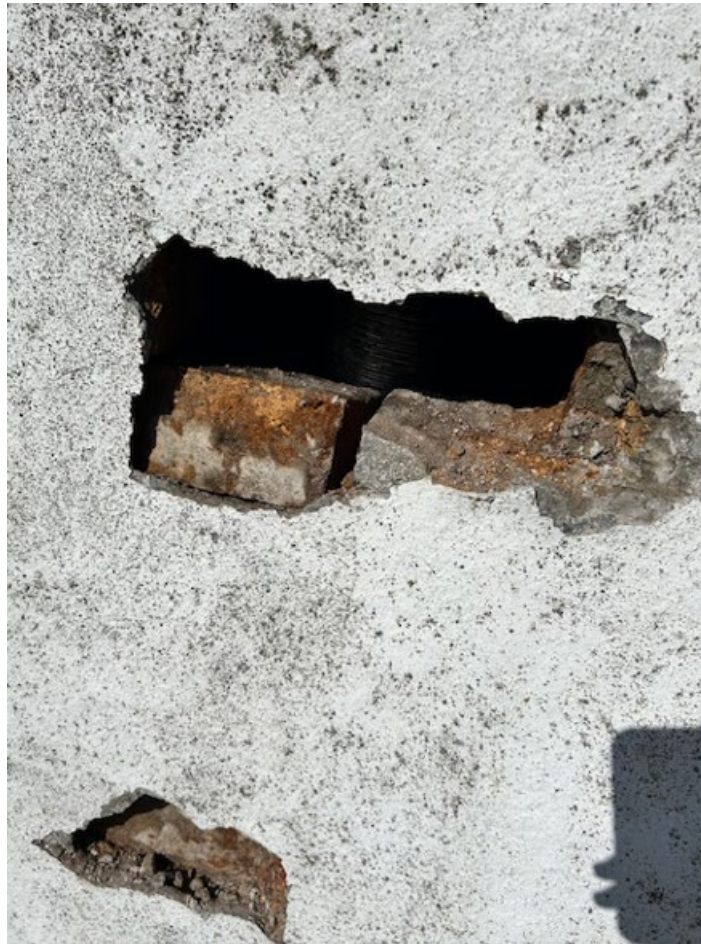
PHOTO 03 LOOSE MASONRY MID WAY DOWN STACK
