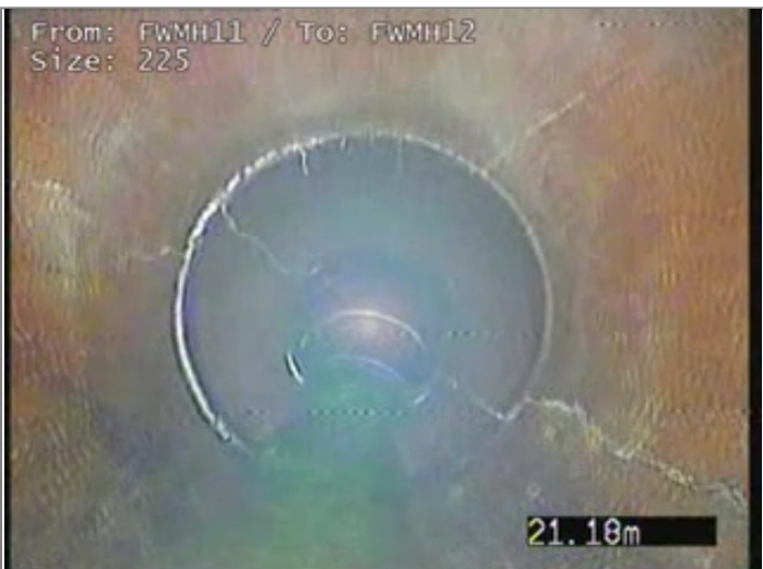
Fracture longitudinal at 4 o'clock
