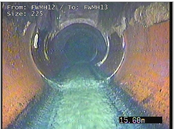
Finish node type, manhole, reference FWMH13
