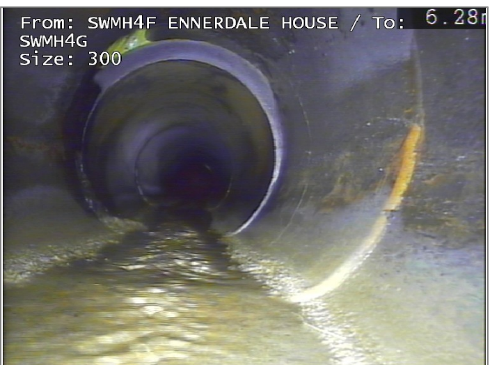
Broken pipe from 10 to 1 o'clock, at joint
