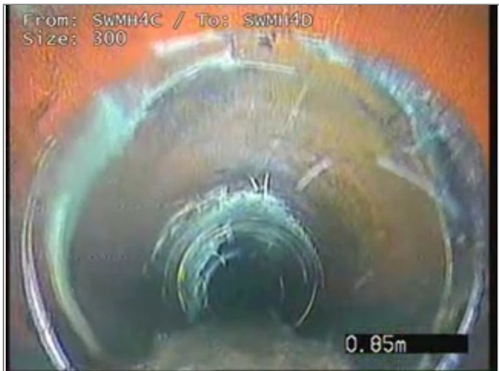
Fracture circumferential from 12 to 6 o'clock at joint
