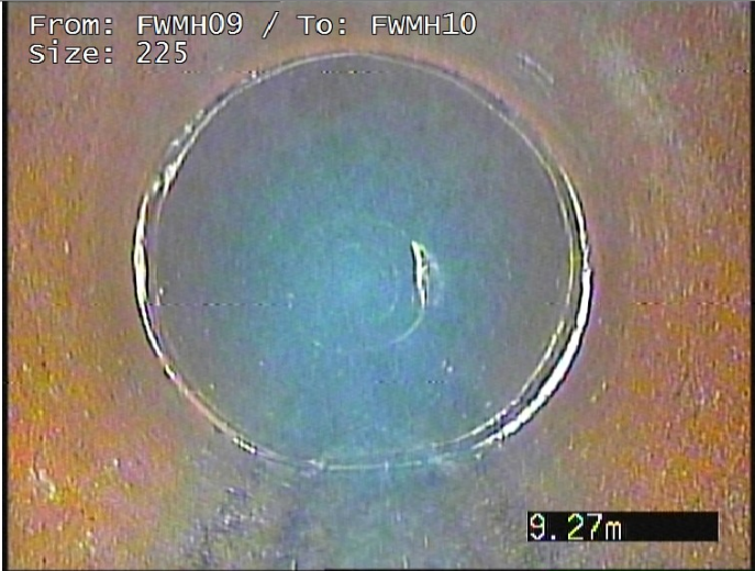
Fracture multiple from 12 to 12 o'clock, Finished
