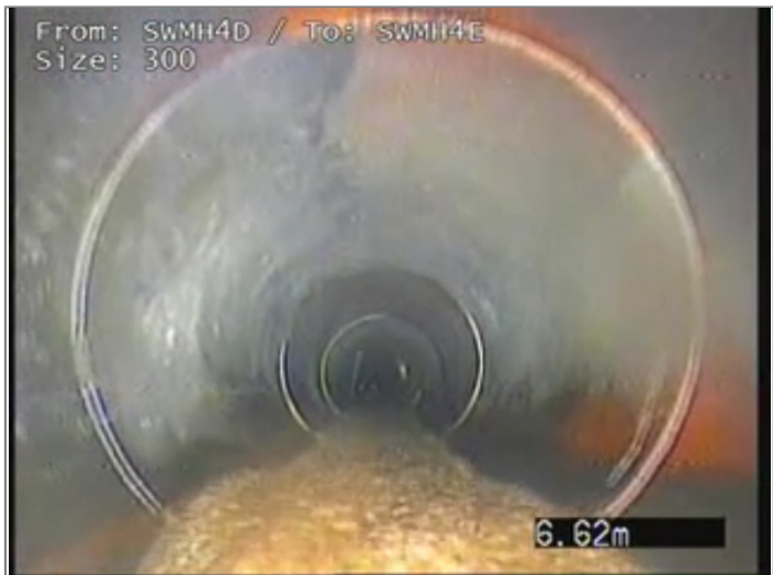
Crack circumferential from 2 to 5 o'clock at joint
