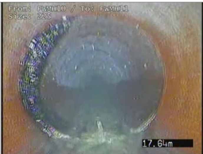
Attached deposits, encrustation from 6 to 11 o'clock 5% cross-sectional area loss at joint
