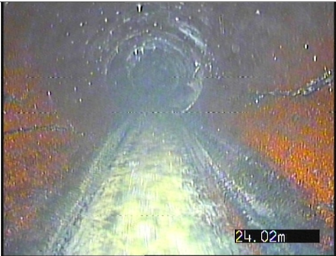
Start node type, manhole, reference FWMH12
