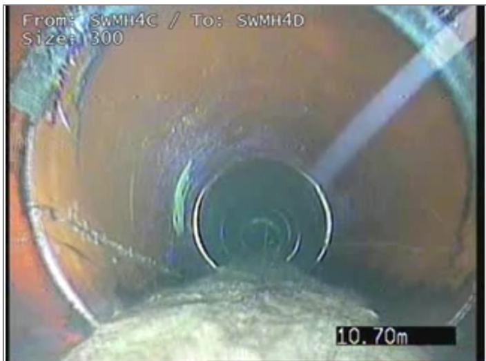
Fracture longitudinal at 8 o'clock
