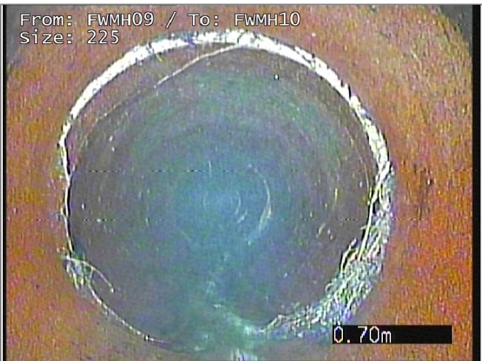
Fracture circumferential from 10 to 12 o'clock
