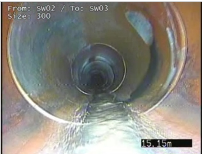
Crack circumferential from 1 to 3 o'clock at joint
