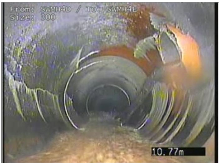
Connection defective, connecting pipe is blocked at 3 o'clock, diameter 150mm, intrusion 10% - Remark: ROOTS NOTED IN CONNECTION
