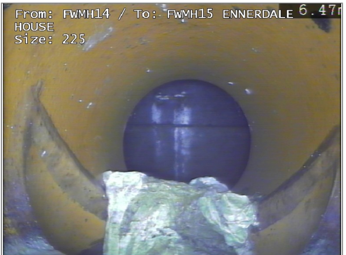
Finish node type, manhole, reference FWMH15
