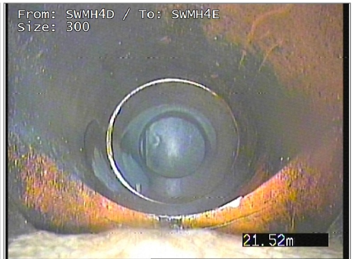
Finish node type, manhole, reference SWMH4E
