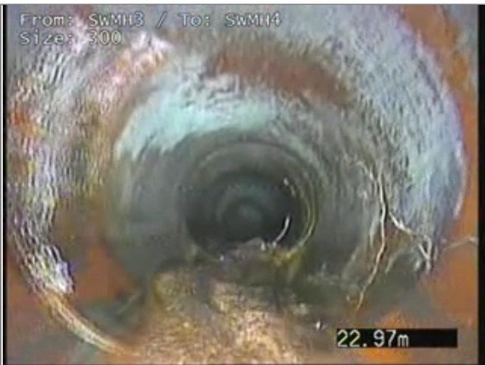
Roots fine at joint
