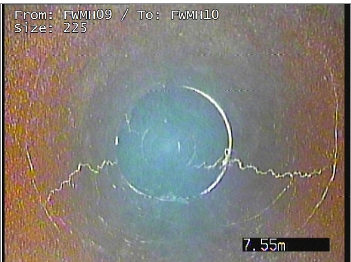
Fracture multiple from 12 to 12 o'clock, Start
