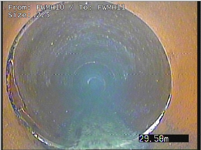
Fracture circumferential from 7 to 10 o'clock
