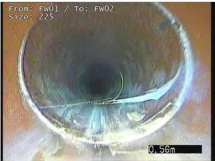
Crack circumferential from 4 to 7 o'clock at joint
