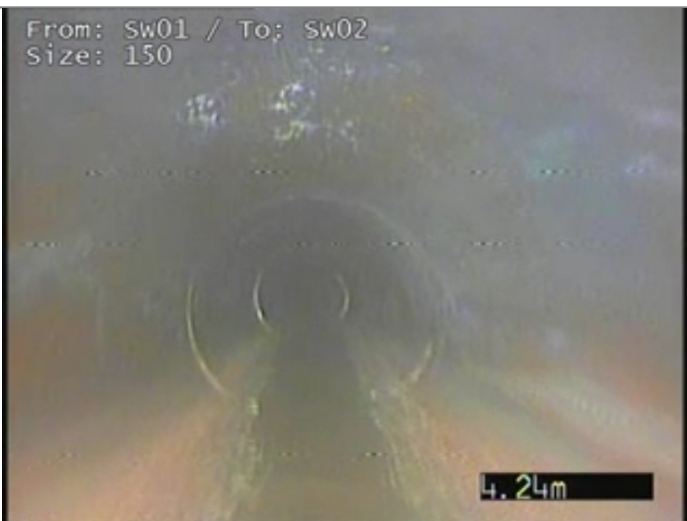
Attached deposits, encrustation from 10 to 5 o'clock 5% cross-sectional area loss, Finished
