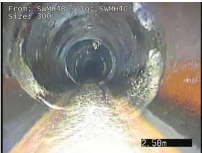
Attached deposits, encrustation from 1 to 9 o'clock 5% cross-sectional area loss at joint
