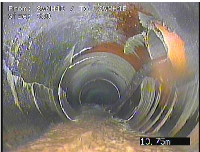
Fracture multiple from 12 to 12 o'clock
