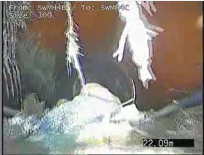
Other obstacles, other from 4 to 8 o'clock 40% cross-sectional area loss - Remark: DEBRIS OR SIMILAR RESTRICTING FLOW.
