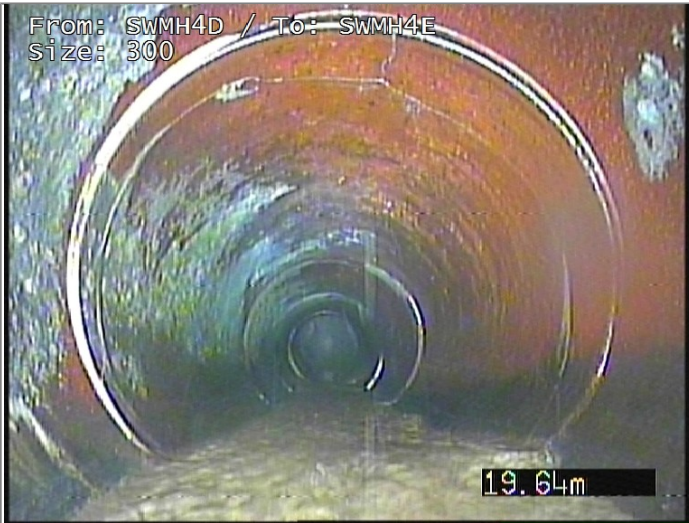
Fracture multiple from 12 to 12 o'clock
