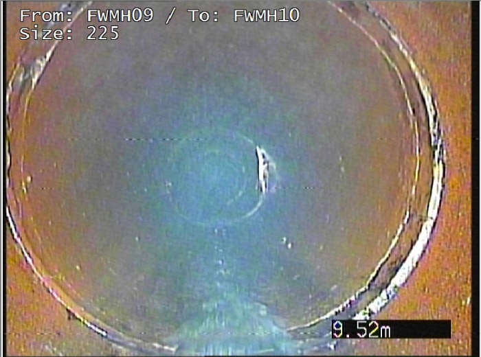
Fracture circumferential from 12 to 12 o'clock
