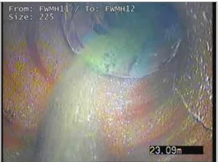
Fracture longitudinal at 4 o'clock
