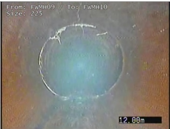
Fracture longitudinal at 12 o'clock
