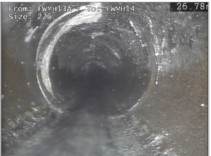
Attached deposits, encrustation from 9 to 12 o'clock 5% cross-sectional area loss, at joint
