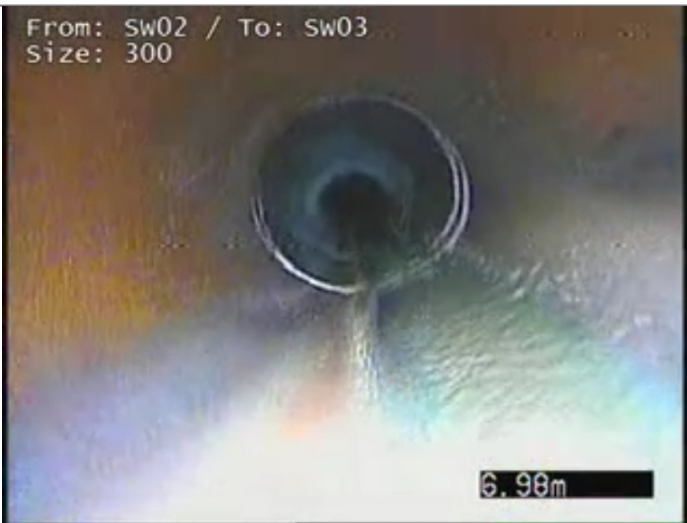
Attached deposits, encrustation from 3 to 6 o'clock 25% cross-sectional area loss, Finished
