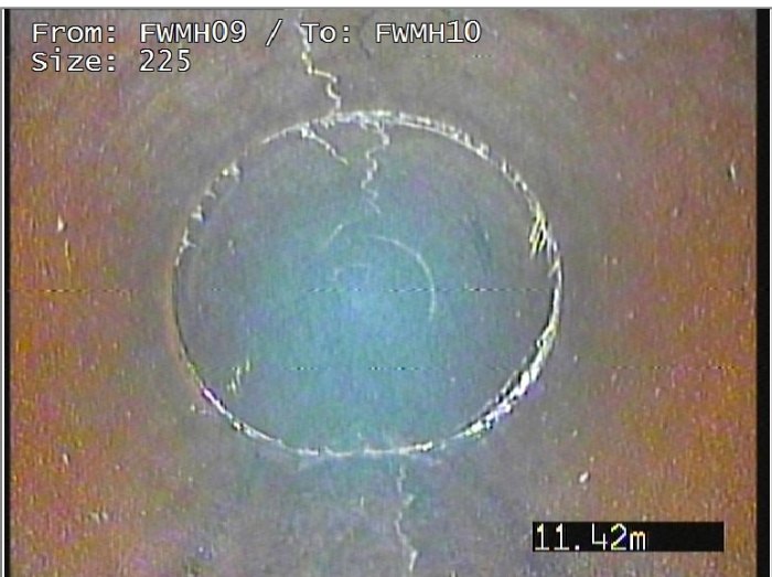
Fracture multiple from 12 to 12 o'clock, Start
