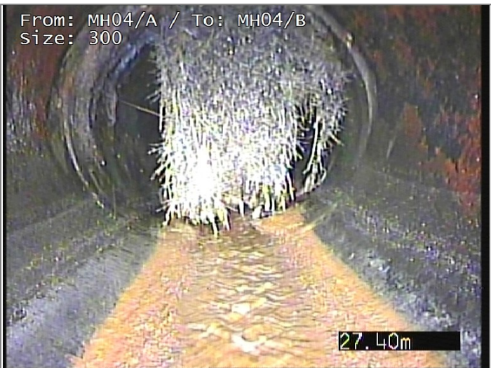
Roots mass 75% cross-sectional area loss
