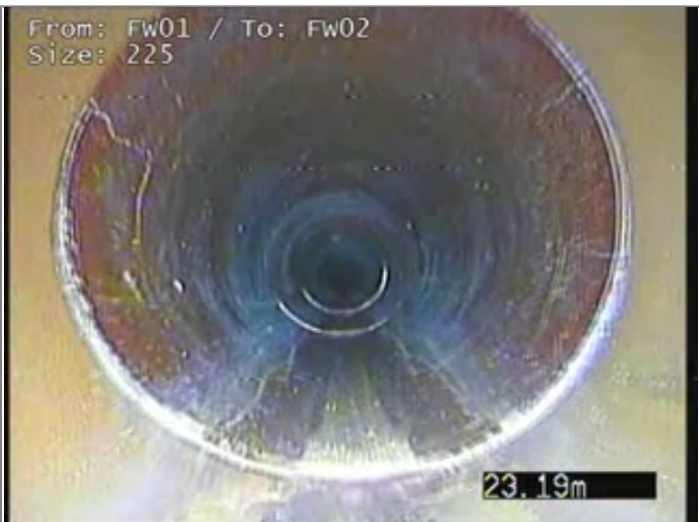
Crack radiates from 9 o'clock
