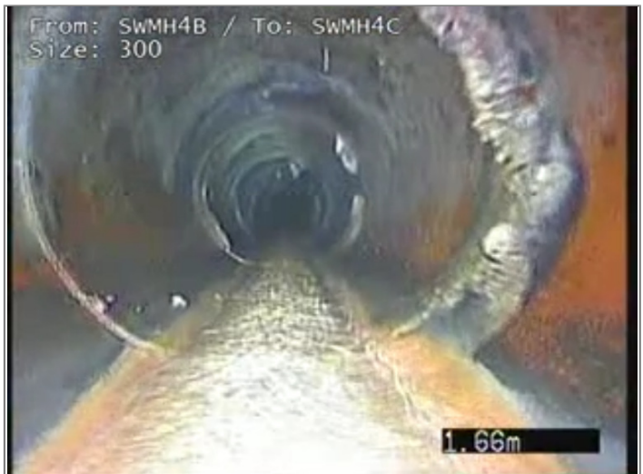
Attached deposits, encrustation from 12 to 6 o'clock 10% cross-sectional area loss at joint
