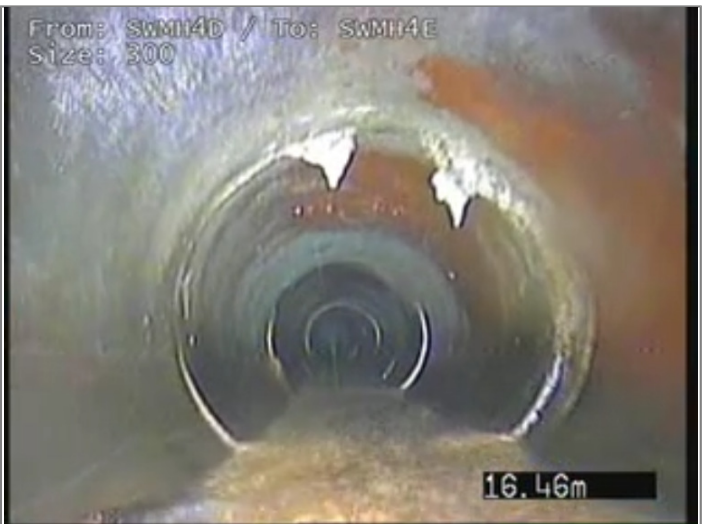
Roots fine at joint
