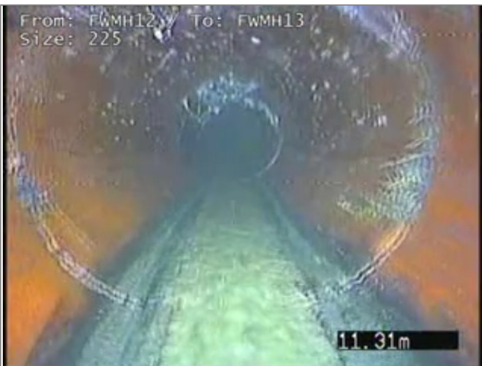
Roots fine at joint
