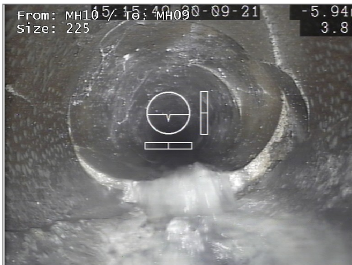
Broken pipe from 12 to 11 o'clock
