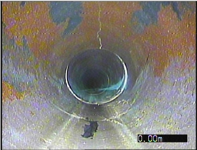
Start node type, manhole, reference FW01
