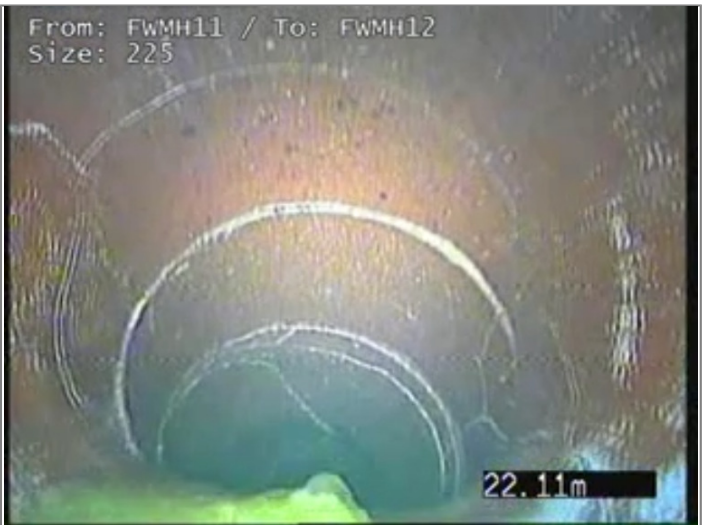
Fracture circumferential from 7 to 5 o'clock
