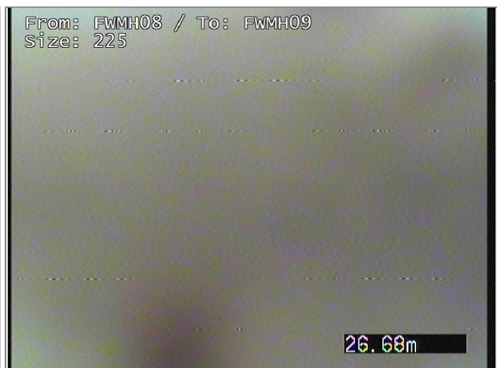
Survey abandoned - Remark: LINE REQUIRES TANKER HPWJ
