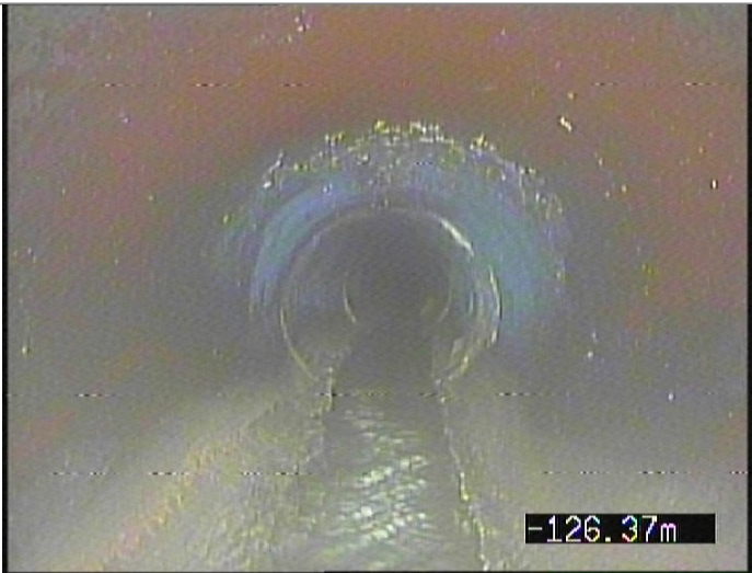
Start node type, manhole, reference SW01
