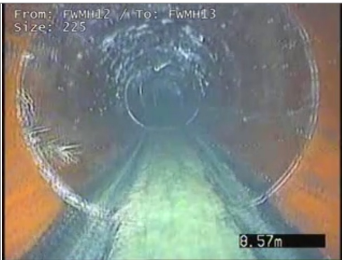
Roots fine at joint
