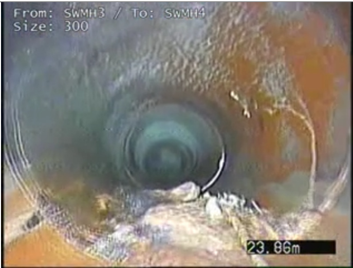
Crack circumferential from 8 to 10 o'clock at joint
