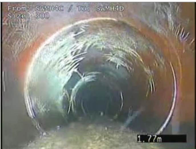
Roots fine at joint
