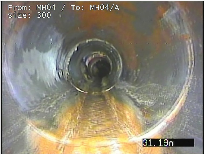
Fracture multiple from 12 to 12 o'clock, Finished
