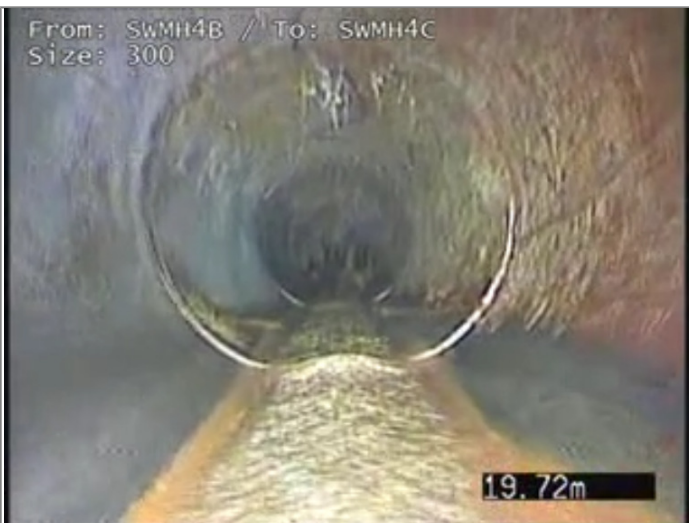
Roots fine at joint
