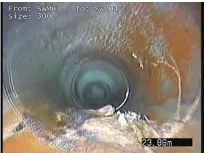
Fracture circumferential from 3 to 6 o'clock at joint
