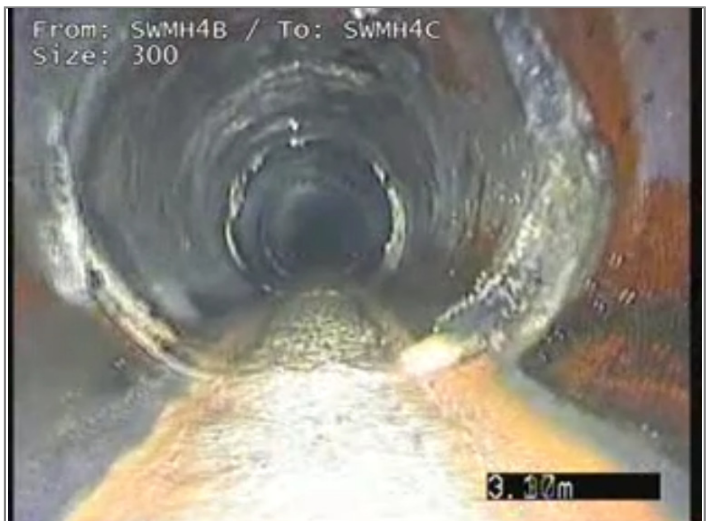
Attached deposits, encrustation from 1 to 6 o'clock 5% cross-sectional area loss at joint
