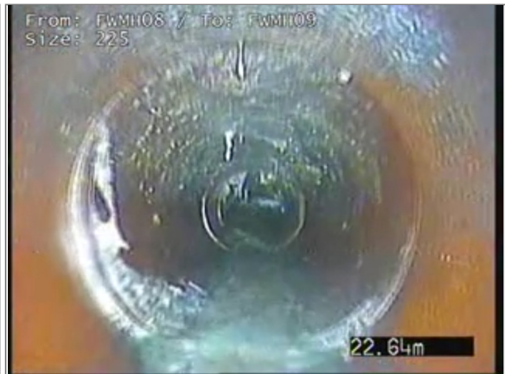
Roots fine at joint
