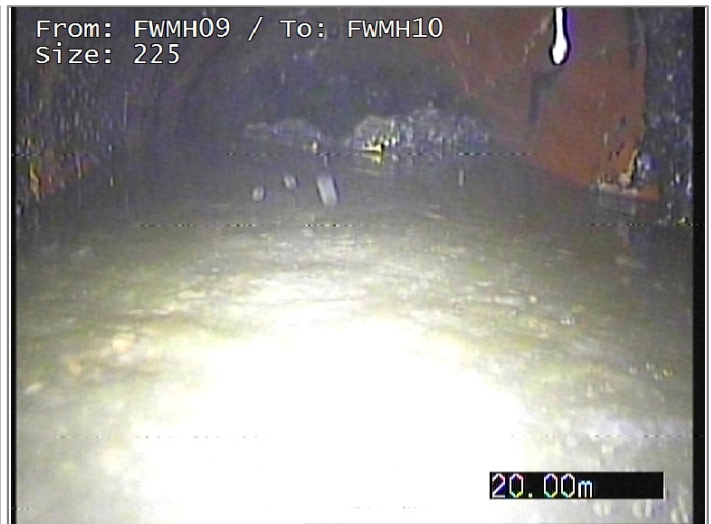
Survey abandoned - Remark: UNABLE TO CONTINUE WITH ROOT CUT AND CCTV REPAIRS WILL NEED TO BE MADE TO LINE
