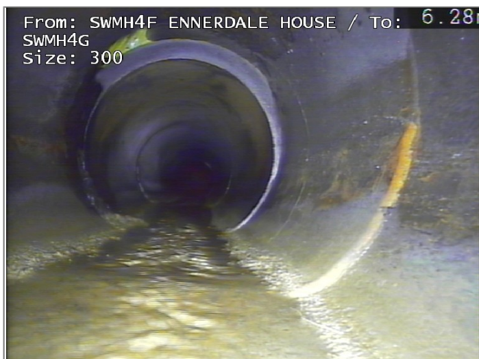
Fracture circumferential from 12 to 6 o'clock
