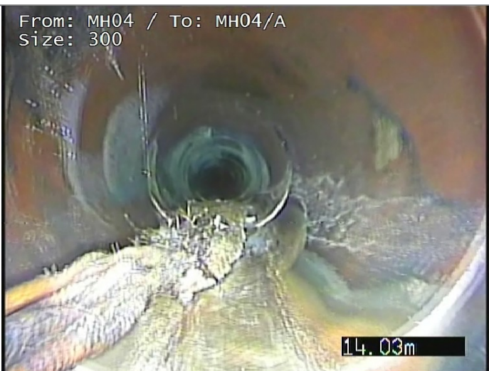
Attached deposits, encrustation at 7 o'clock 5% cross-sectional area loss, Finished
