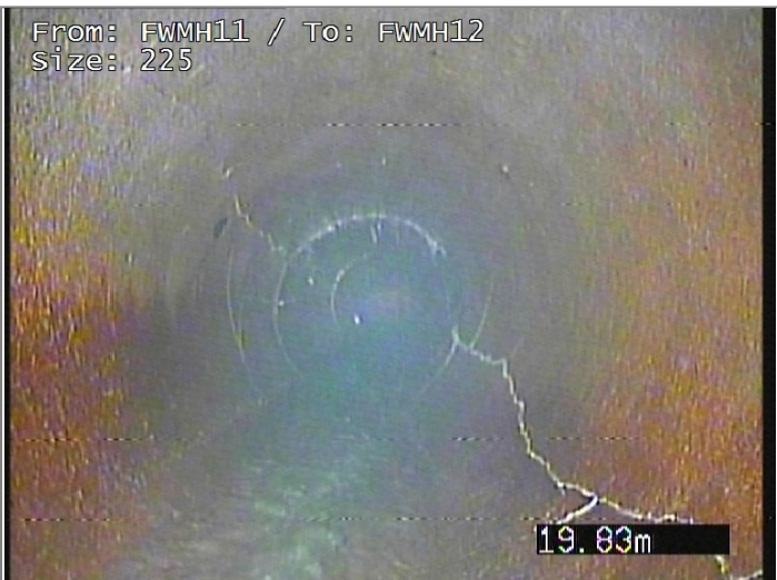
Fracture multiple from 12 to 12 o'clock, Start
