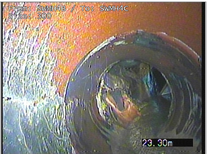
Survey abandoned - Remark: UNABLE TO PASS DEFECT
