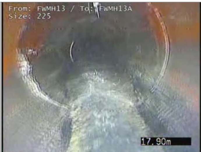
Attached deposits, encrustation at 9 o'clock 5% cross-sectional area loss at joint
