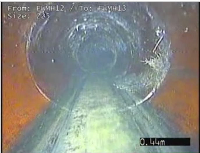
Roots fine at joint
