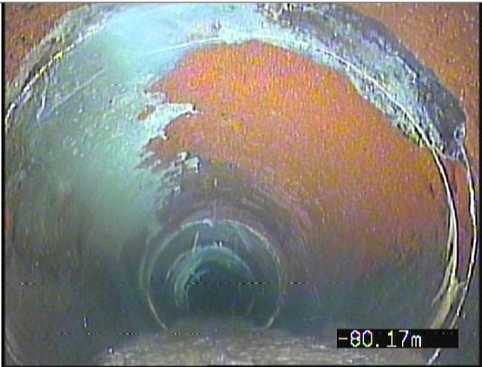
Start node type, manhole, reference SWMH4C
