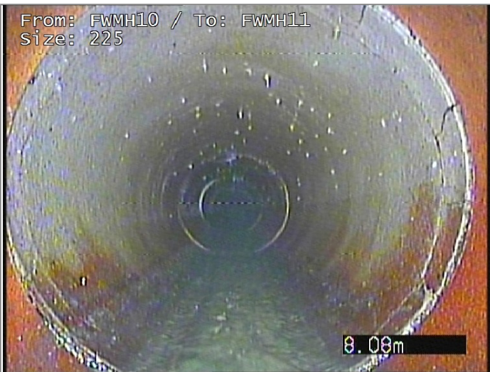
Fracture multiple from 12 to 6 o'clock
