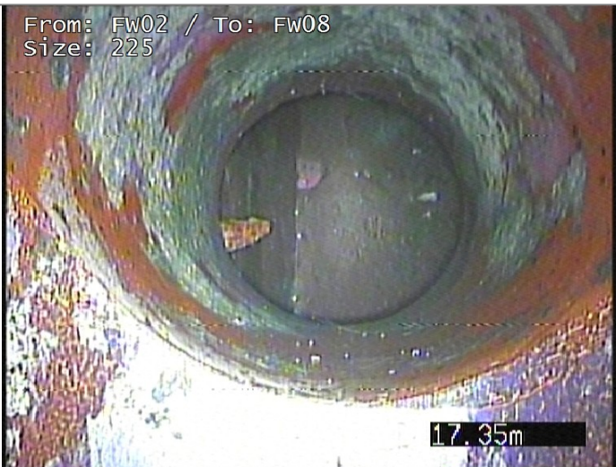
Finish node type, manhole, reference FW08
