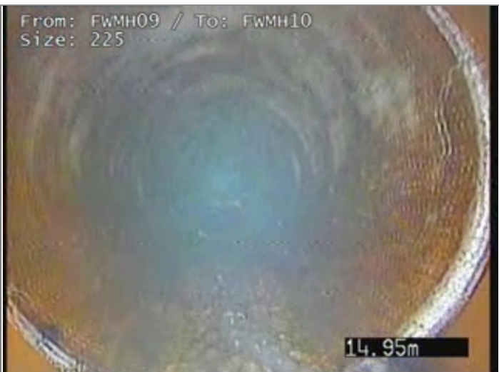
Crack circumferential from 2 to 3 o'clock at joint
