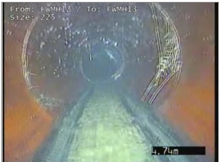
Roots fine at joint
