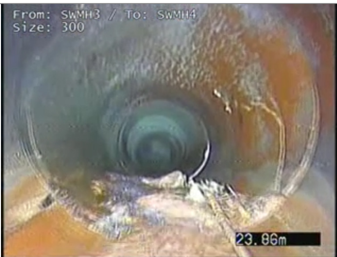
Roots mass 25% cross-sectional area loss at joint
