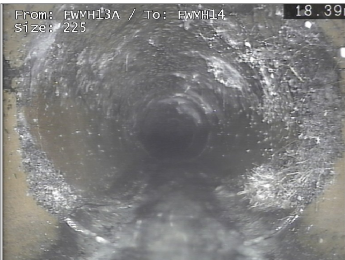
Roots mass 25% cross-sectional area loss
