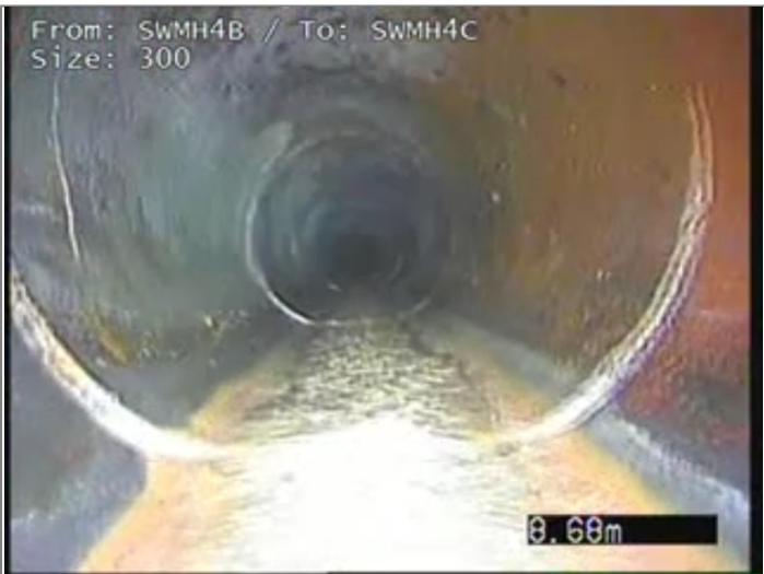
Crack circumferential from 9 to 11 o'clock
