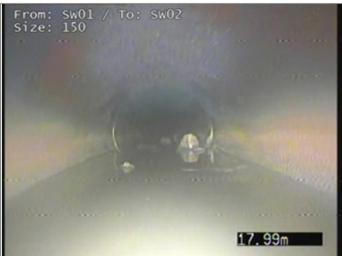
Settled deposits coarse 50% cross-sectional area loss, Start
