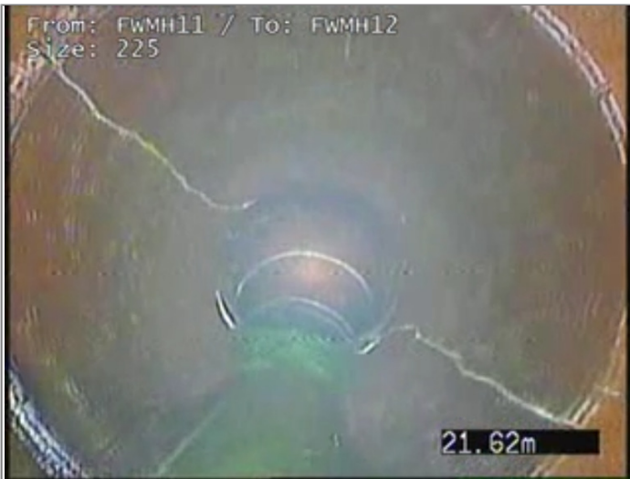
Fracture longitudinal at 10 o'clock
