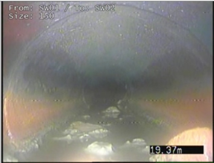
Settled deposits coarse 50% cross-sectional area loss, Finished
