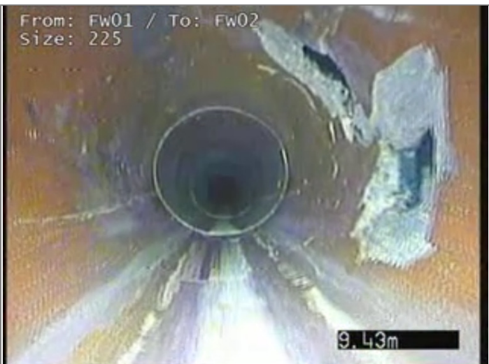
Hole in drain/sewer from 2 to 4 o'clock
