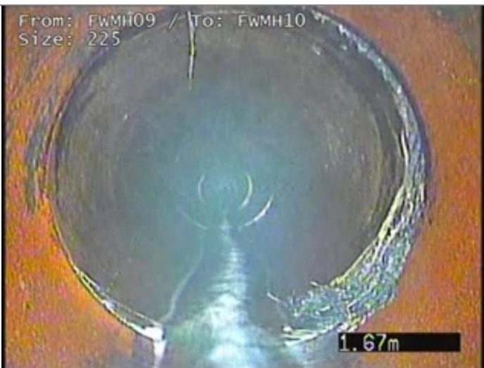
Crack circumferential from 3 to 8 o'clock at joint
