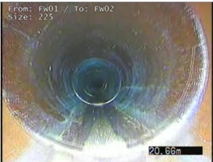
Crack circumferential from 3 to 6 o'clock at joint
