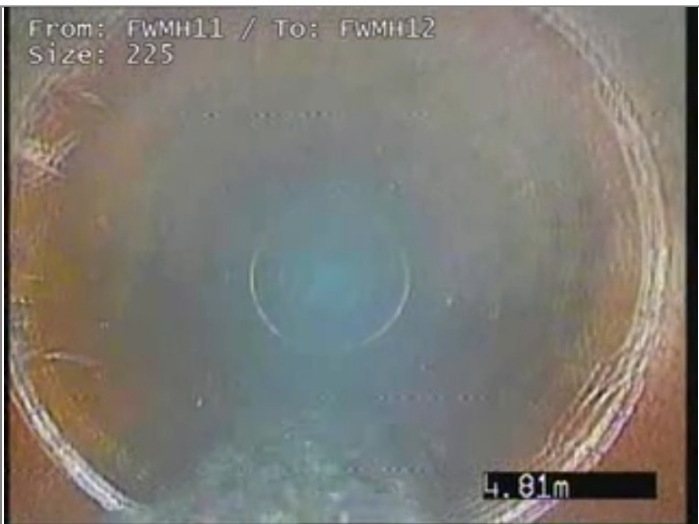
Crack circumferential from 4 to 5 o'clock at joint
