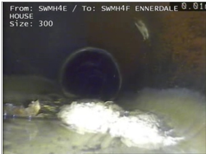
Attached deposits, encrustation from 5 to 6 o'clock 10% cross-sectional area loss, Start
