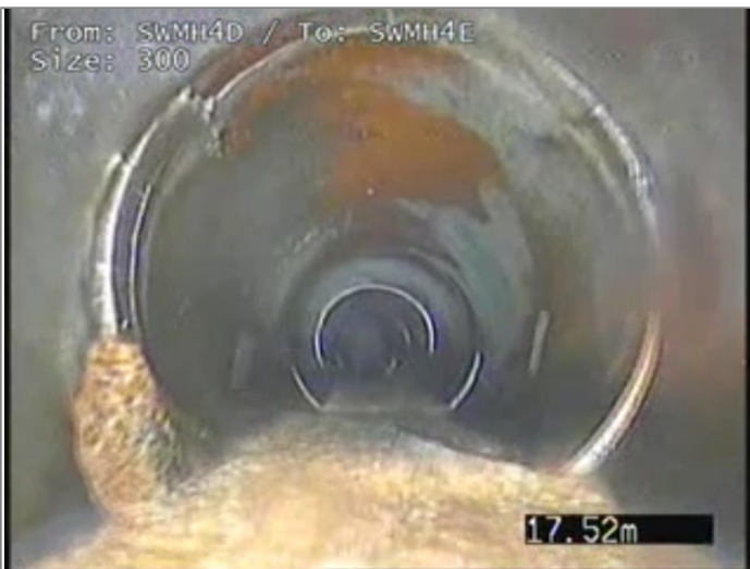
Attached deposits, encrustation from 6 to 9 o'clock 5% cross-sectional area loss at joint
