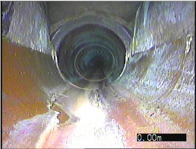
Start node type, manhole, reference FW02
