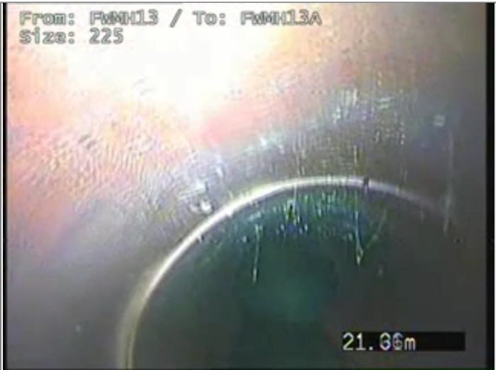
Loss of vision, camera under water, Finished
