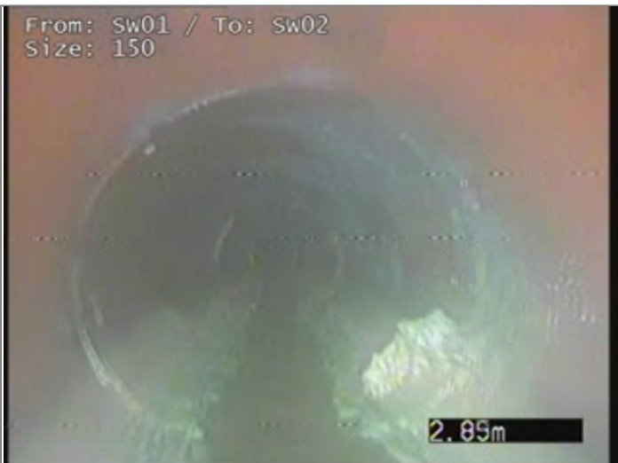
Attached deposits, encrustation at 5 o'clock 5% cross-sectional area loss at joint
