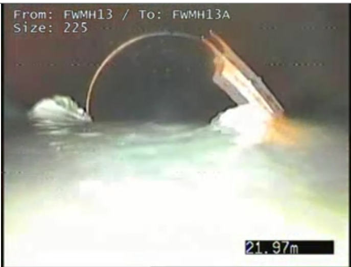
Other obstacles, other from 3 to 9 o'clock 50% cross-sectional area loss - Remark: UNKNOWN OBSTRUCTION RESTRICTING FLOW.
