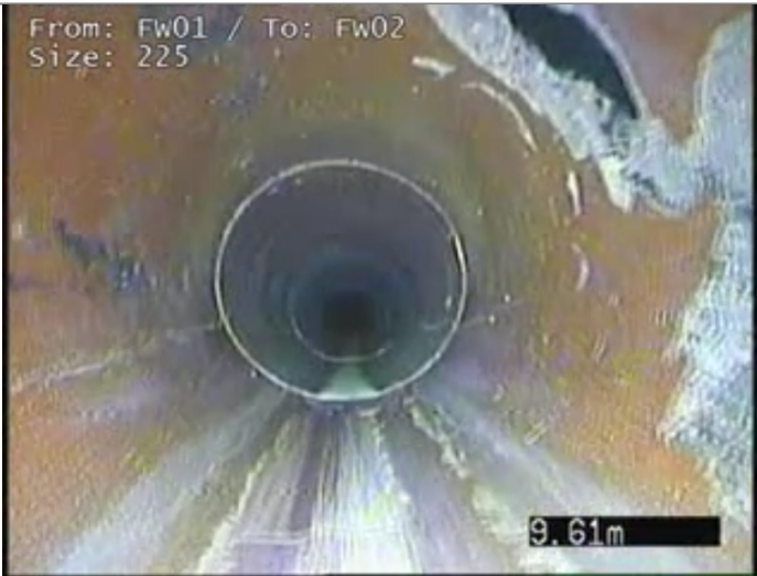
Hole in drain/sewer from 12 to 3 o'clock
