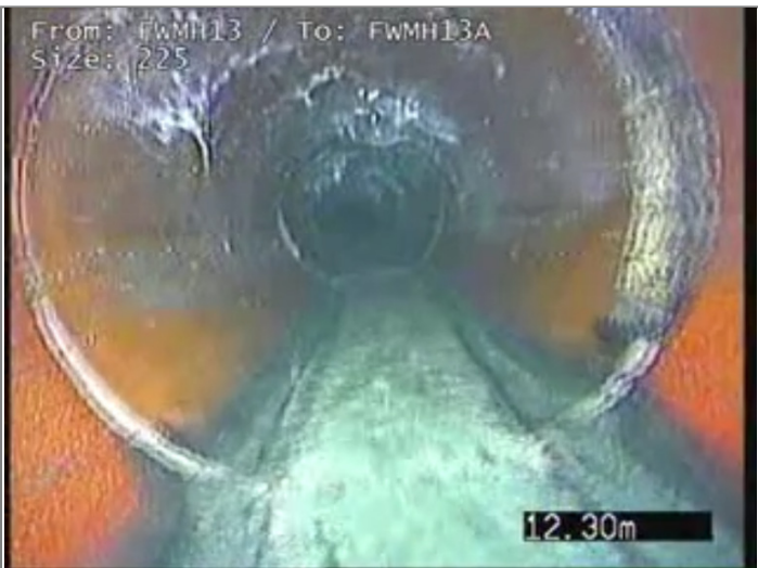
Attached deposits, encrustation from 12 to 4 o'clock 5% cross-sectional area loss at joint
