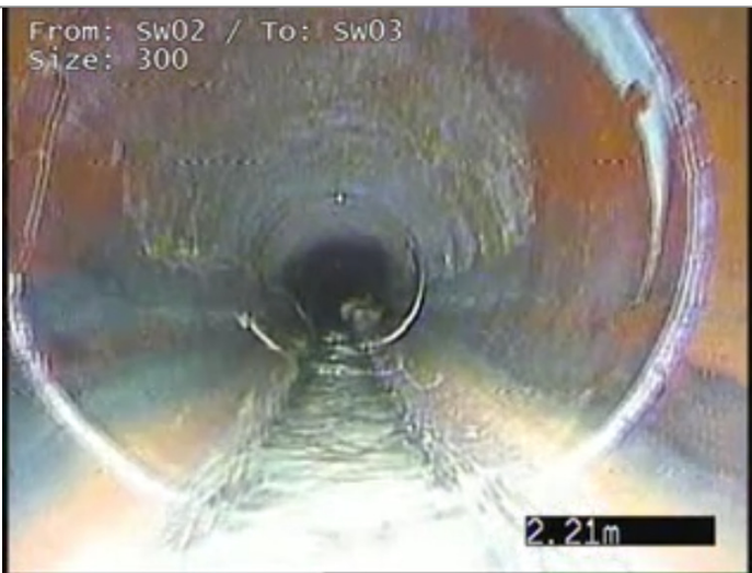
Crack circumferential from 9 to 11 o'clock at joint
