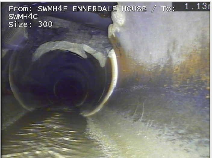
Hole in drain/sewer from 10 to 2 o'clock
