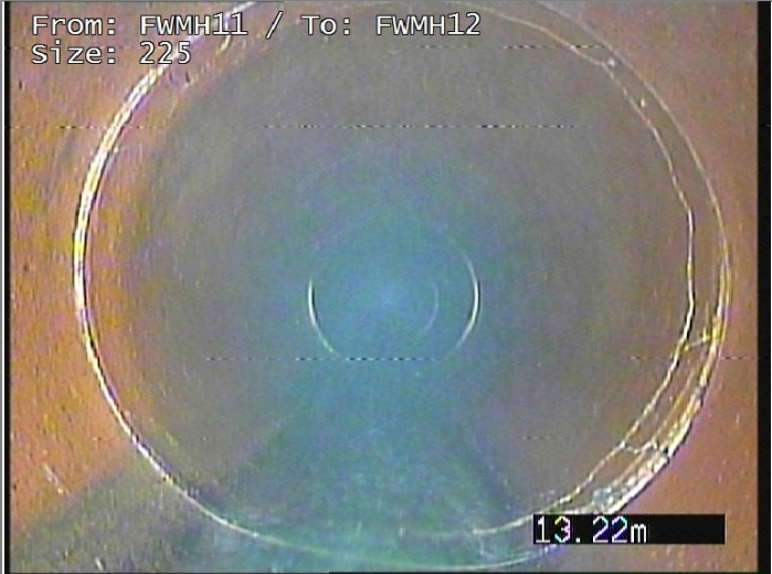
Fracture circumferential from 12 to 6 o'clock
