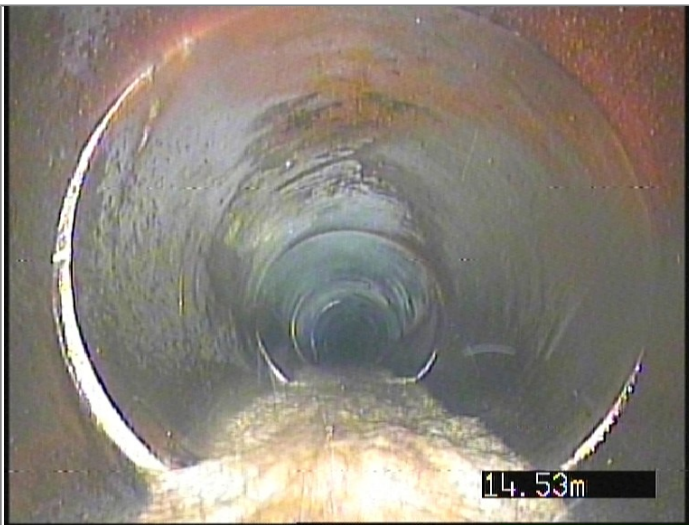
Start node type, manhole, reference SWMH4D
