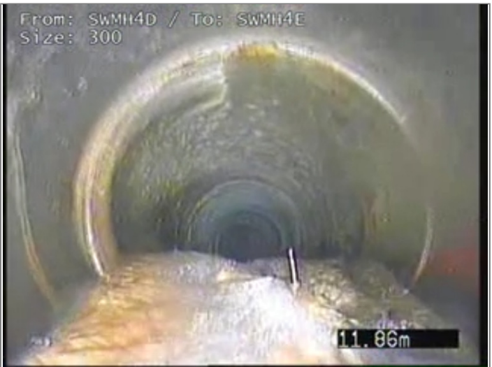
Fracture circumferential from 7 to 10 o'clock
