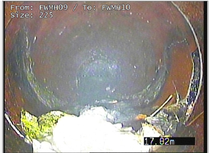
Broken pipe from 2 to 8 o'clock
