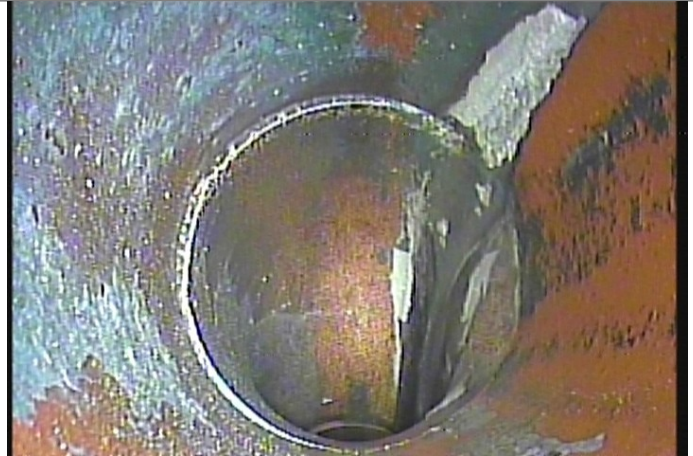
Access problems: MH06 U/S MH05 LIMITED ACCESS FOR CCTV
