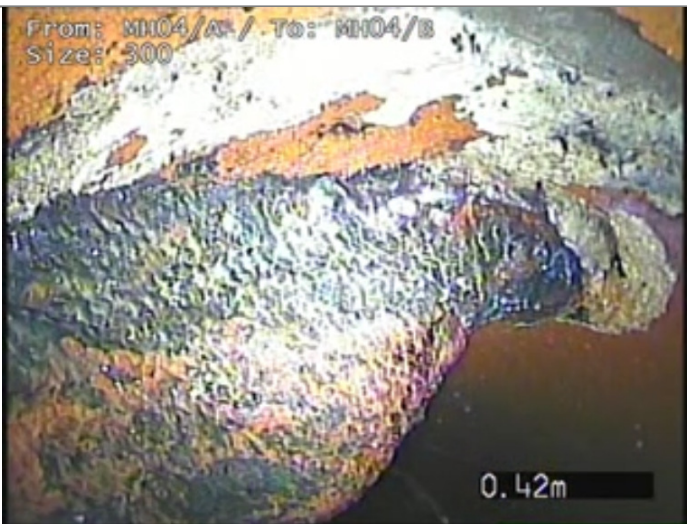
Attached deposits, encrustation from 6 to 12 o'clock 25% cross-sectional area loss
