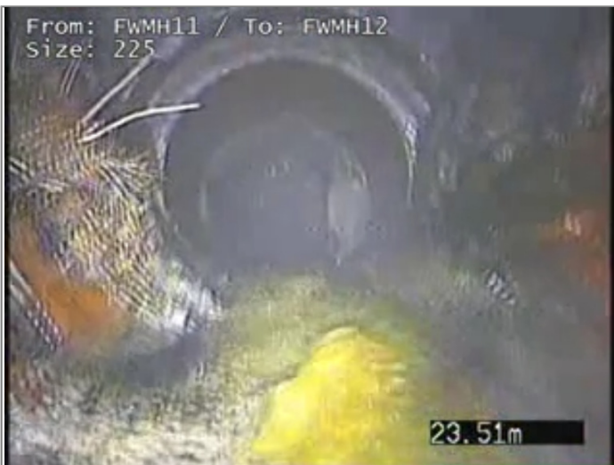
Roots mass 10% cross-sectional area loss - Remark: IN MANHOLE
