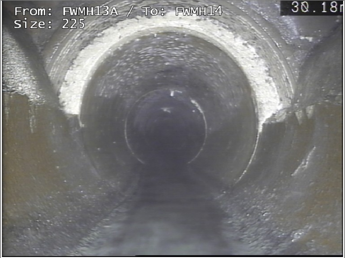
Finish node type, manhole, reference FWMH14
