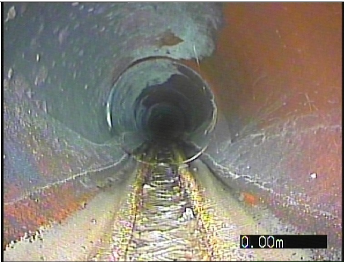
Start node type, manhole, reference SWMH04
