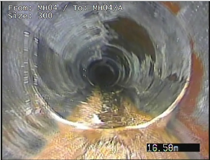
Roots mass 20% cross-sectional area loss, Finished
