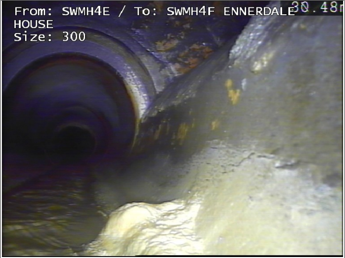
Finish node type, manhole, reference SWMH4F ENNERDALE HOUSE
