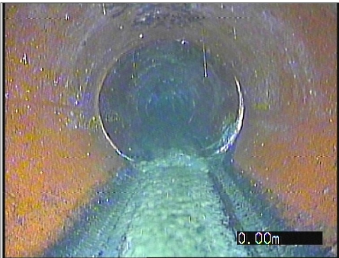
Start node type, manhole, reference FWMH13
