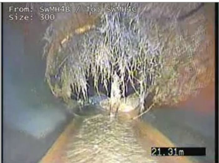
Roots mass 50% cross-sectional area loss at joint
