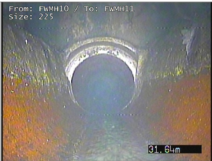
Finish node type, manhole, reference FWMH11
