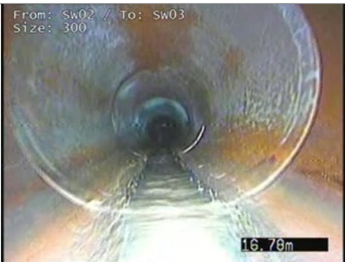
Crack circumferential from 1 to 4 o'clock at joint
