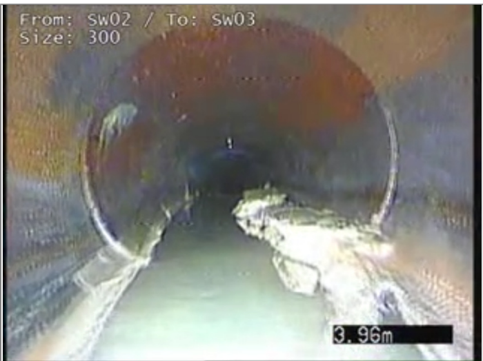
Attached deposits, encrustation from 4 to 6 o'clock 10% cross-sectional area loss, Start
