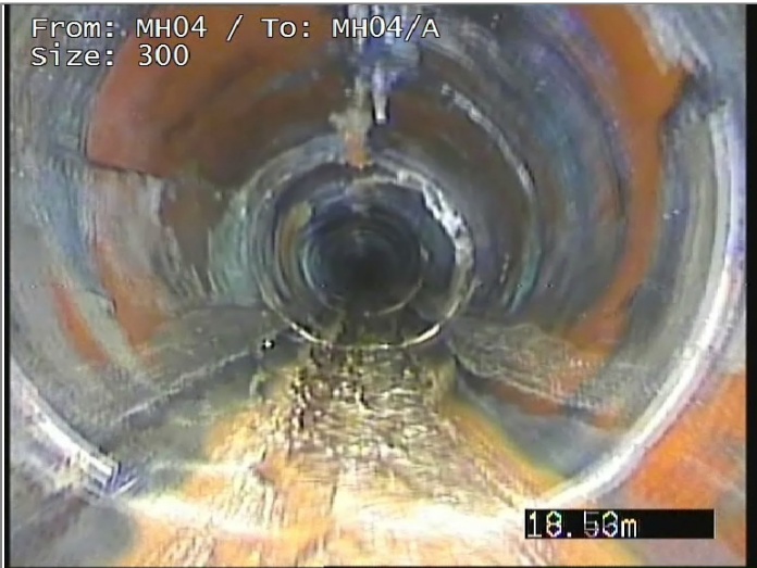
Fracture multiple from 12 to 12 o'clock, Start
