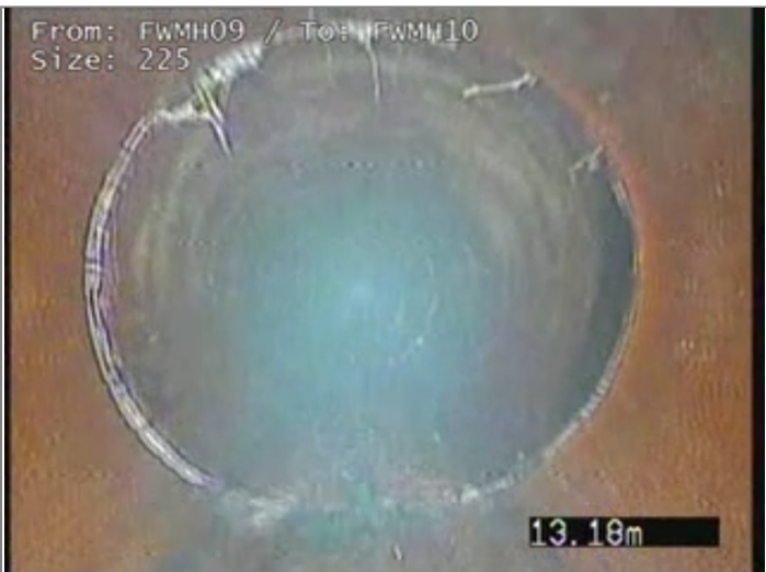
Roots fine at joint - Remark: FINE ROOTS REMAIN POST ROOT CUT.
