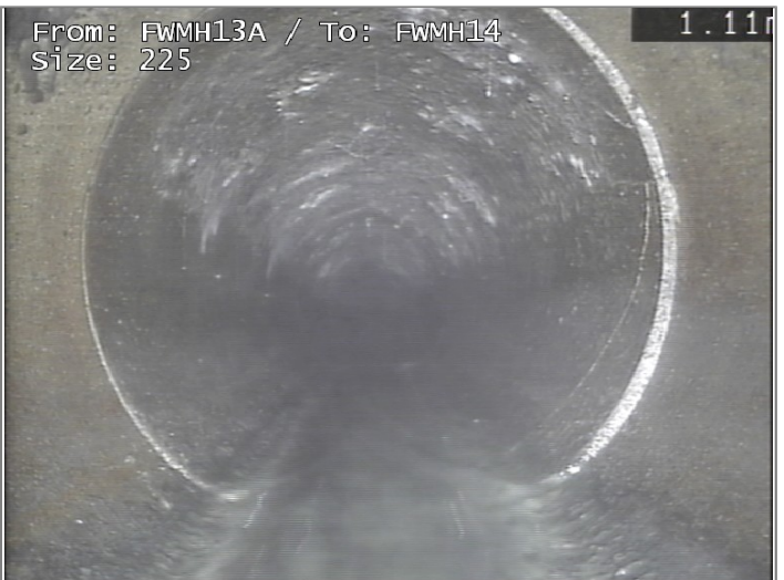
Crack circumferential from 2 to 6 o'clock, at joint
