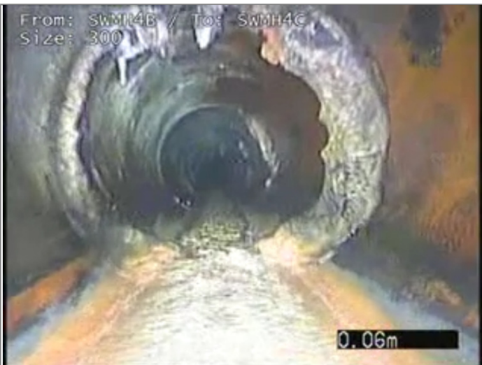
Attached deposits, encrustation from 12 to 6 o'clock 20% cross-sectional area loss at joint
