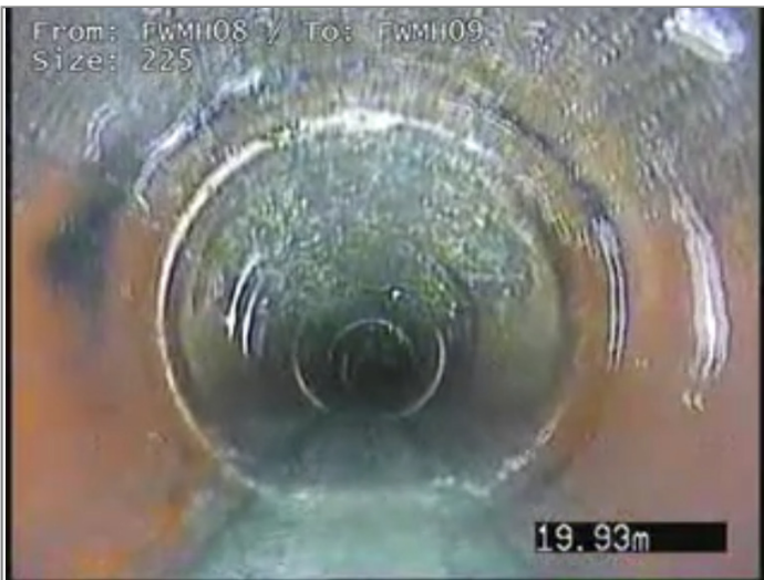
Fracture circumferential from 2 to 4 o'clock
