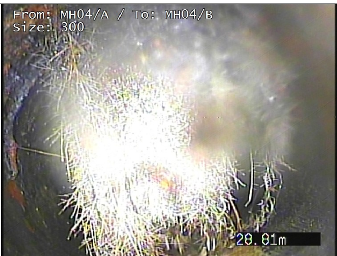
Survey abandoned - Remark: UNABLE TO PASS ROOT MASS
