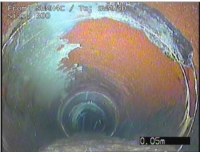
Fracture multiple from 12 to 12 o'clock
