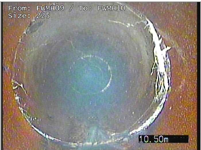
Fracture multiple from 12 to 12 o'clock
