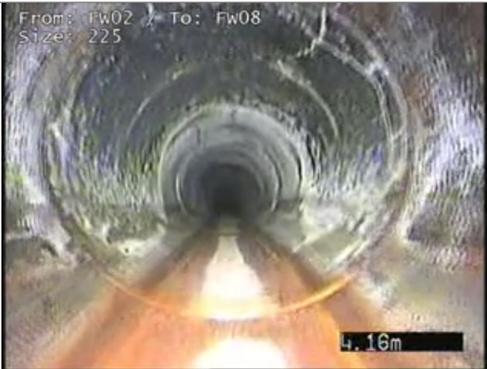
Fracture circumferential from 12 to 3 o'clock at joint
