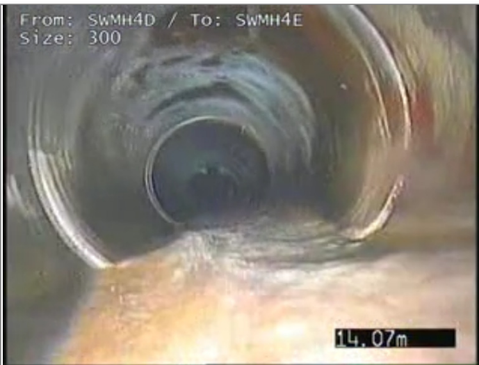
Fracture circumferential from 2 to 5 o'clock at joint
