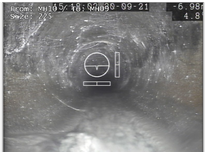
Survey abandoned - Remark: UNABLE TO PASS DEFECT
