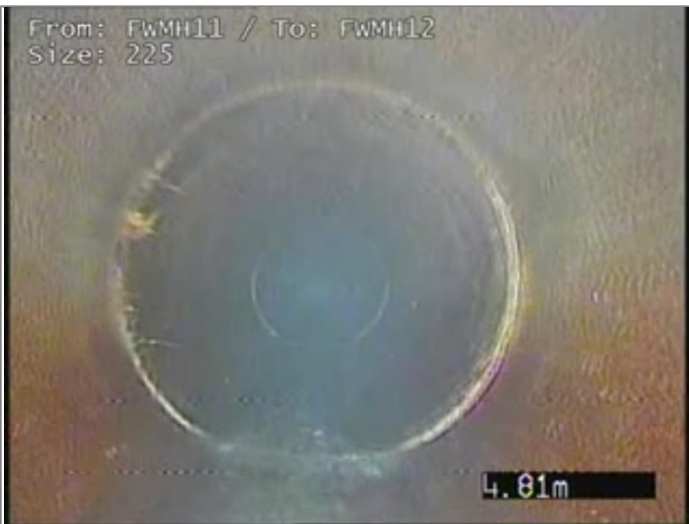
Roots fine at joint
