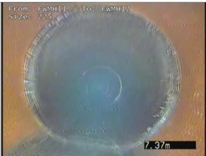
Roots fine at joint
