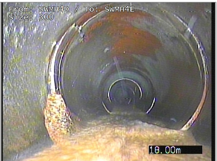
Fracture multiple from 12 to 12 o'clock
