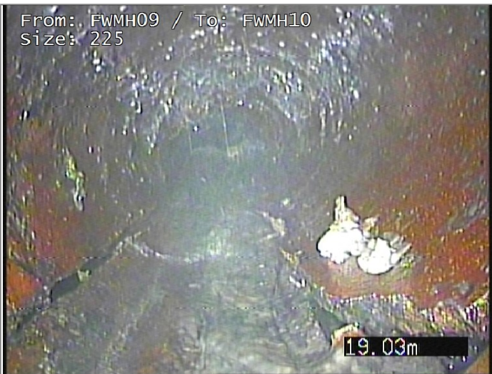
Broken pipe from 3 to 9 o'clock
