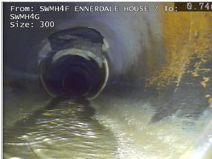
Crack circumferential from 1 to 5 o'clock, at joint
