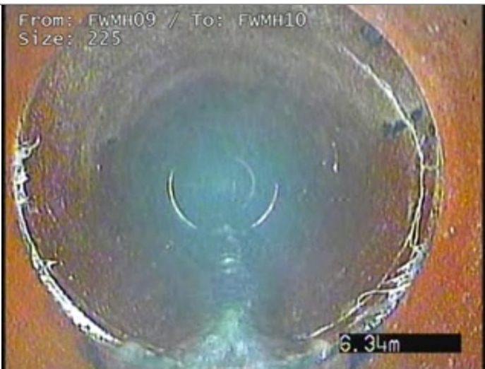
Roots fine at joint - Remark: FINE ROOTS REMAIN POST ROOT CUTTING
