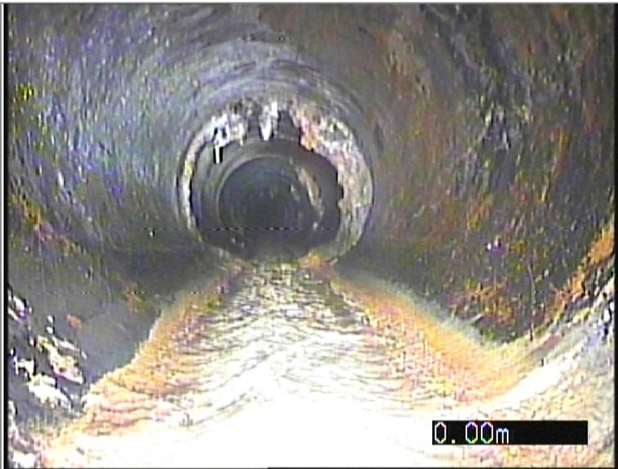
Start node type, manhole, reference SWMH4B
