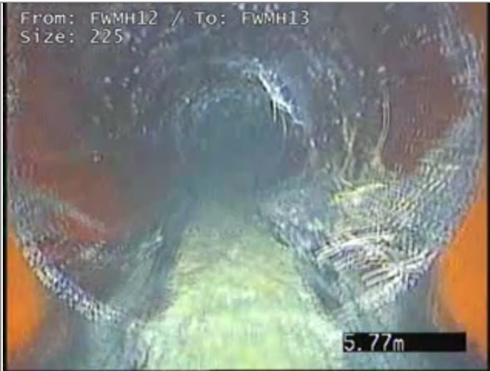
Roots mass 5% cross-sectional area loss at joint
