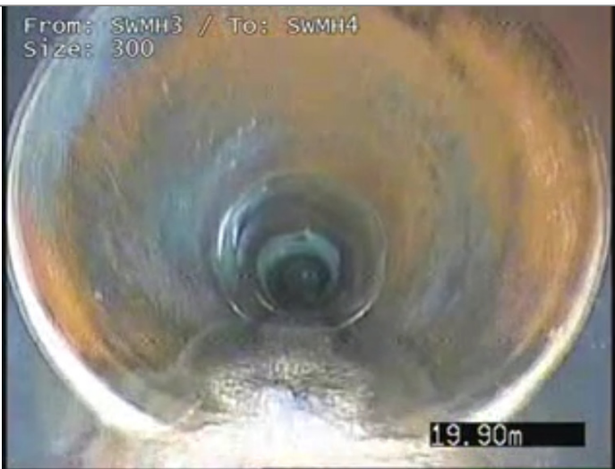
Crack circumferential from 2 to 5 o'clock at joint
