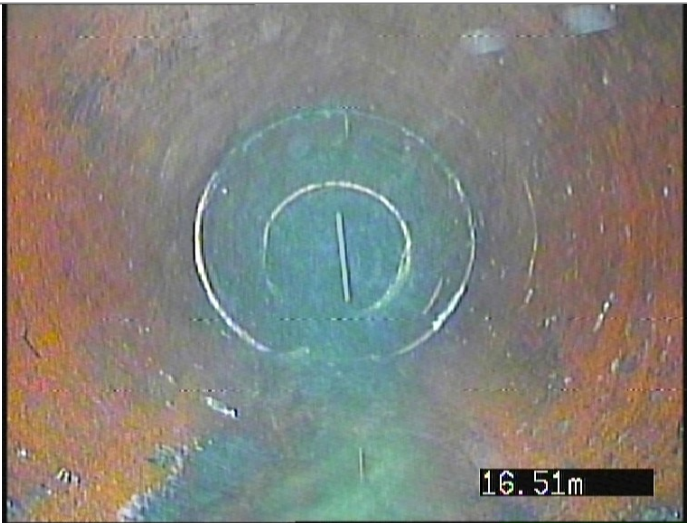
Start node type, manhole, reference FWMH09
