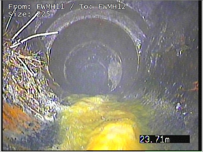
Finish node type, manhole, reference FWMH12
