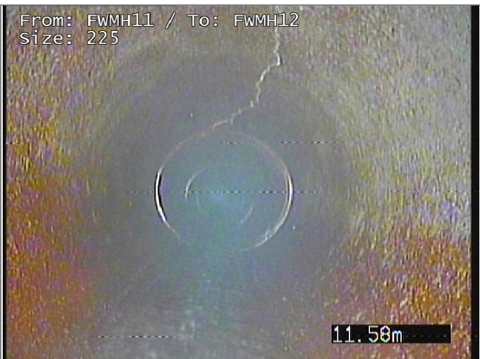
Fracture longitudinal at 12 o'clock
