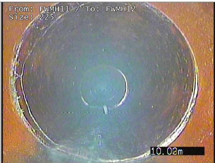
Fracture circumferential from 6 to 12 o'clock
