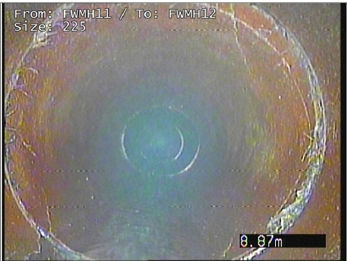
Fracture circumferential from 12 to 3 o'clock
