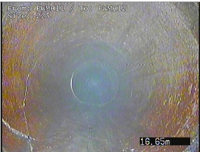
Fracture multiple from 6 to 12 o'clock
