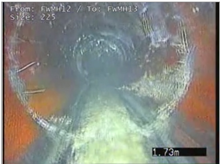
Roots fine at joint
