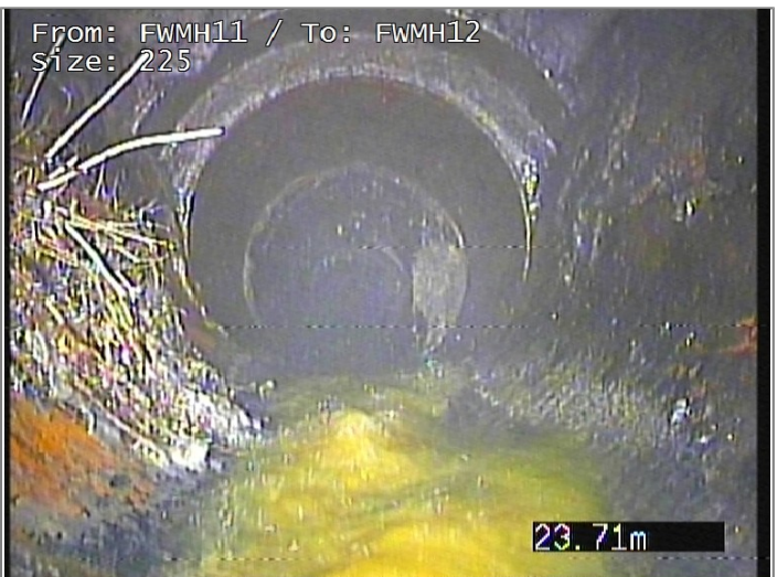
Fracture multiple from 12 to 12 o'clock, Finished
