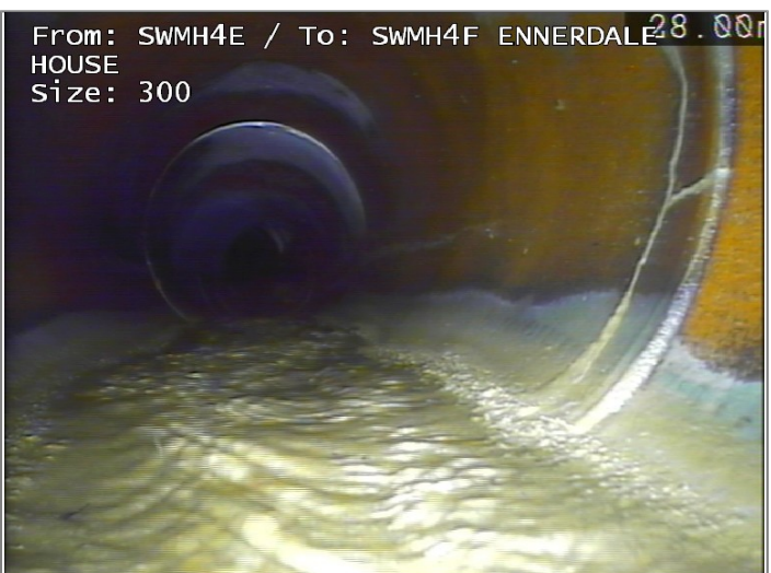
Fracture circumferential from 1 to 6 o'clock, at joint
