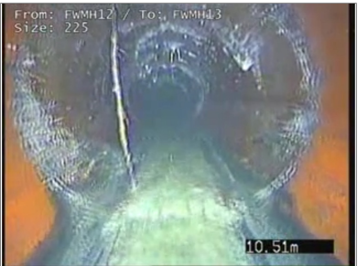
Roots mass 5% cross-sectional area loss at joint
