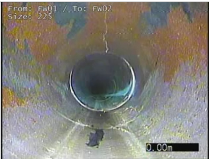
Crack longitudinal at 12 o'clock
