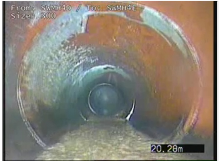
Crack circumferential from 12 to 2 o'clock at joint
