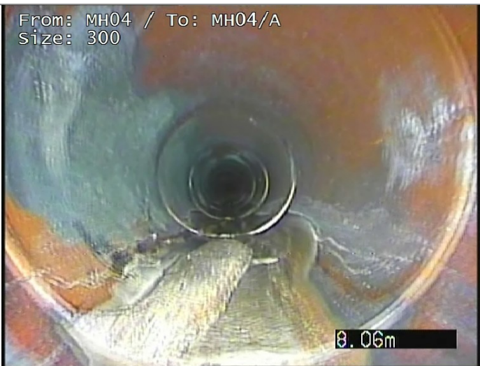
Attached deposits, encrustation at 7 o'clock 5% cross-sectional area loss
