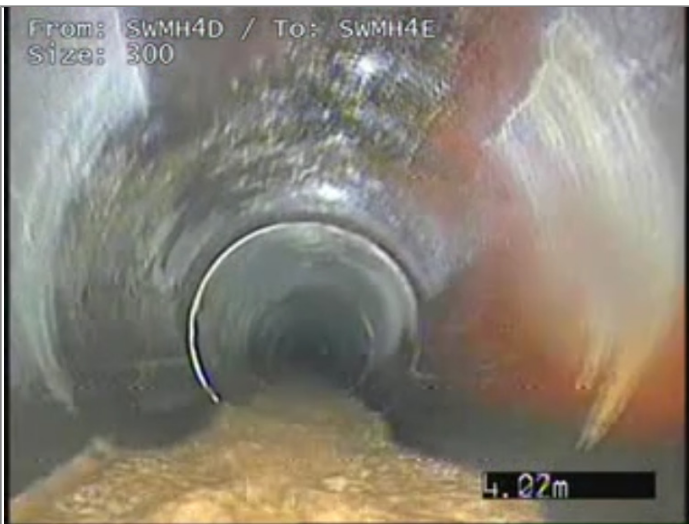
Fracture longitudinal at 2 o'clock
