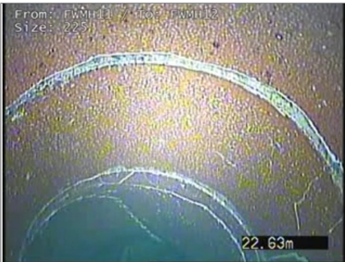
Line of drain/sewer deviates down BENDS DOWN TO THE NEXT MANHOLE.
