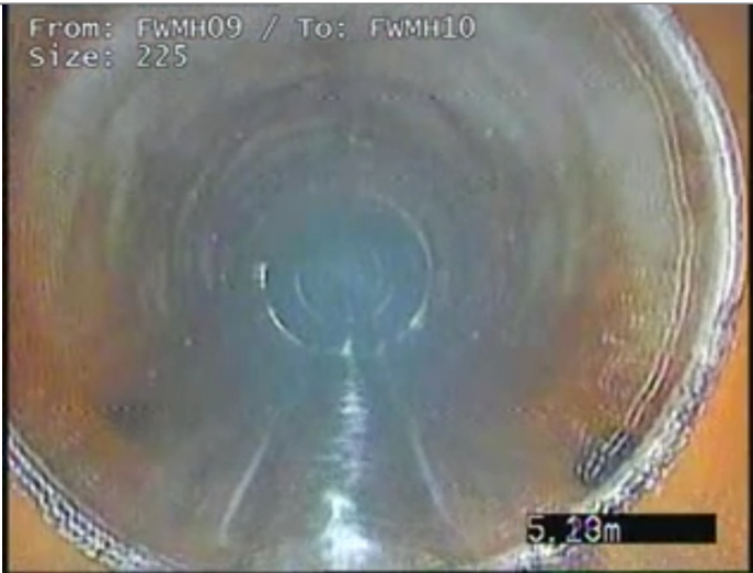
Crack circumferential from 1 to 5 o'clock at joint
