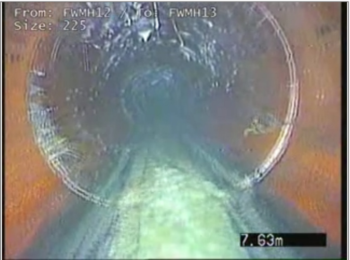
Roots fine at joint
