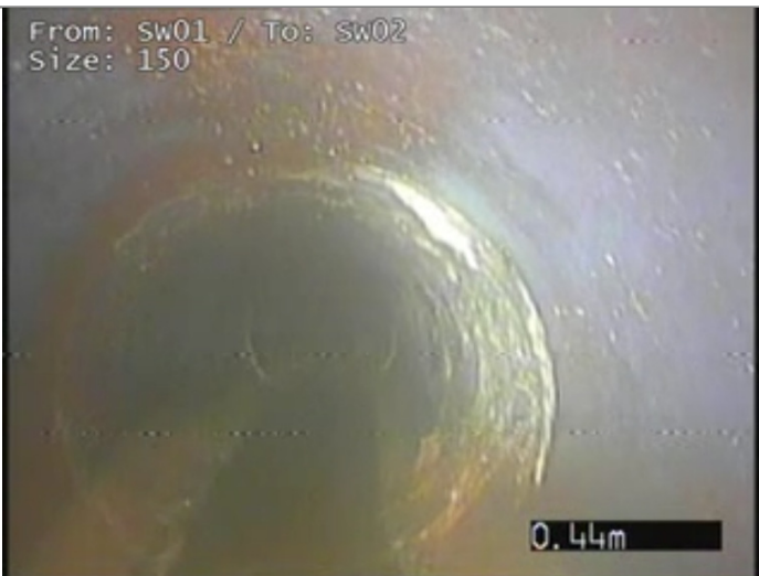
Attached deposits, encrustation from 10 to 5 o'clock 5% cross-sectional area loss, Start
