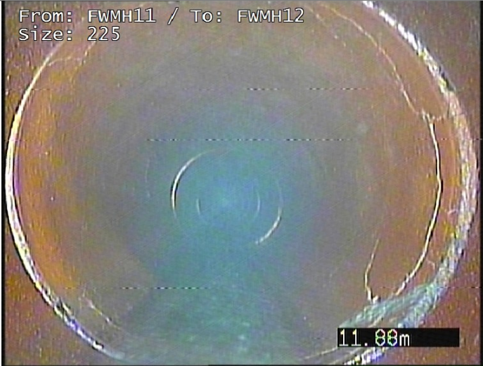
Fracture multiple from 12 to 12 o'clock
