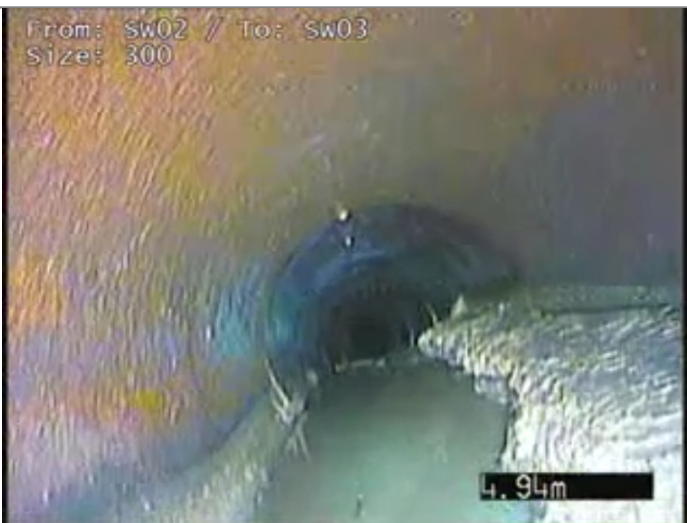
Attached deposits, encrustation from 4 to 6 o'clock 10% cross-sectional area loss, Finished
