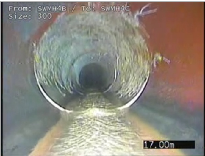
Roots fine at joint
