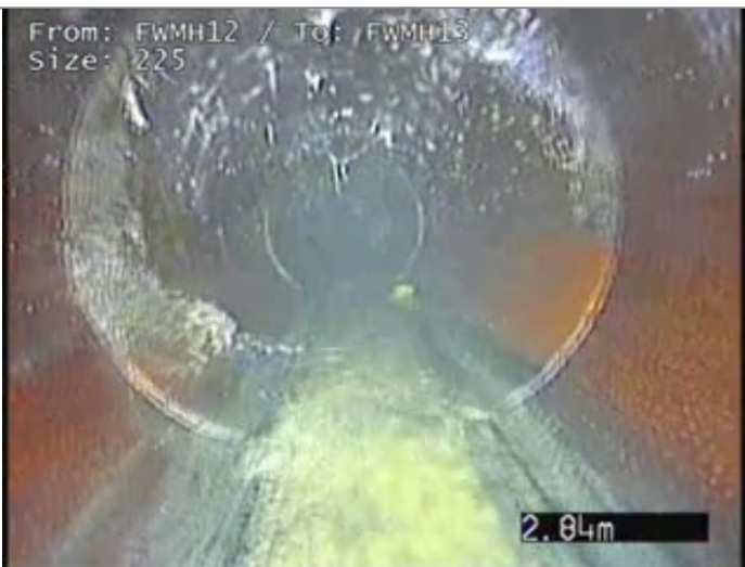
Roots mass 5% cross-sectional area loss at joint
