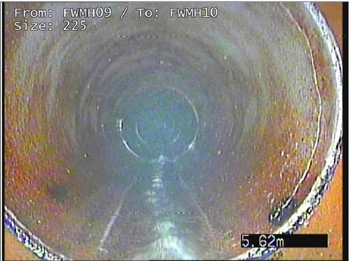
Fracture circumferential from 12 to 5 o'clock
