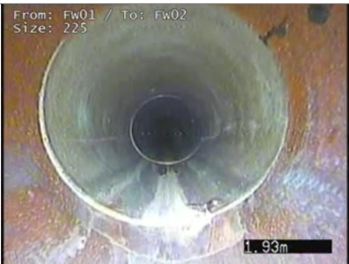
Crack circumferential from 5 to 7 o'clock at joint
