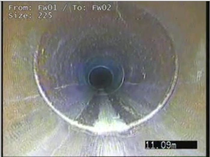
Crack longitudinal at 12 o'clock
