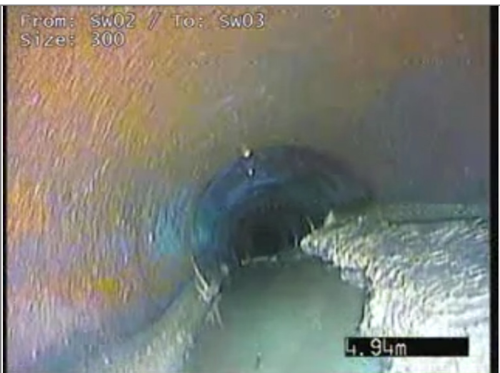
Attached deposits, encrustation from 3 to 6 o'clock 25% cross-sectional area loss, Start
