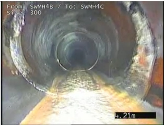
Attached deposits, encrustation from 1 to 6 o'clock 5% cross-sectional area loss at joint
