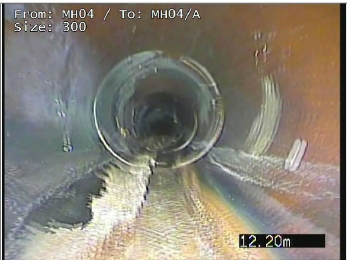
Attached deposits, encrustation at 7 o'clock 5% cross-sectional area loss, Start
