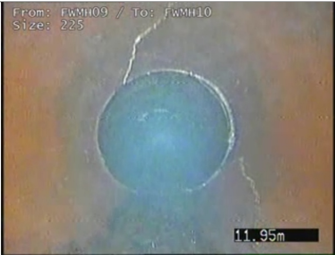
Fracture longitudinal at 4 o'clock
