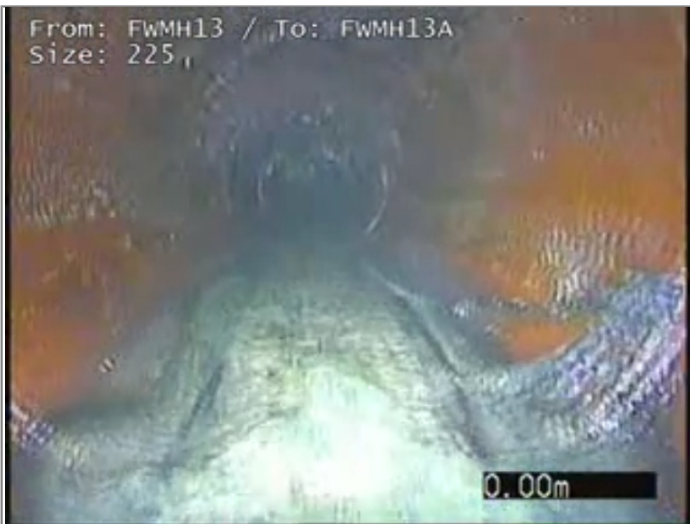
Roots fine at joint
