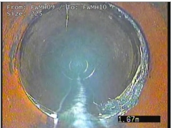
Roots fine at joint - Remark: ROOT REMAINING POST ROOT CUTTING.
