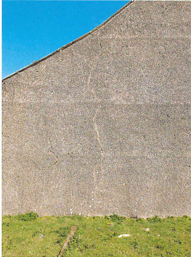
PHOTO 03 VIEW ON CRACKING TO LEFT HAND ELEVATION
