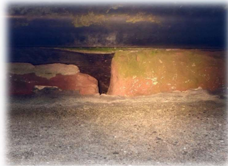
Plate 6: Gap at wallhead/tabling.
