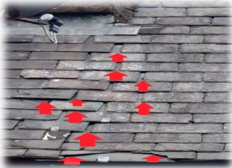
Plate 5: Slipped slates close to chimney and adjoining property.
