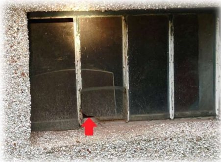
Plate 7: Crack and gap at top of window (E. aspect).
