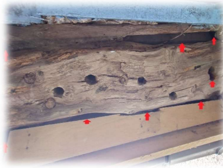
Plate 11: Gap under door lintel.
