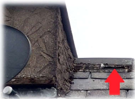
Plate 3: Gap under ridge (W. aspect).
