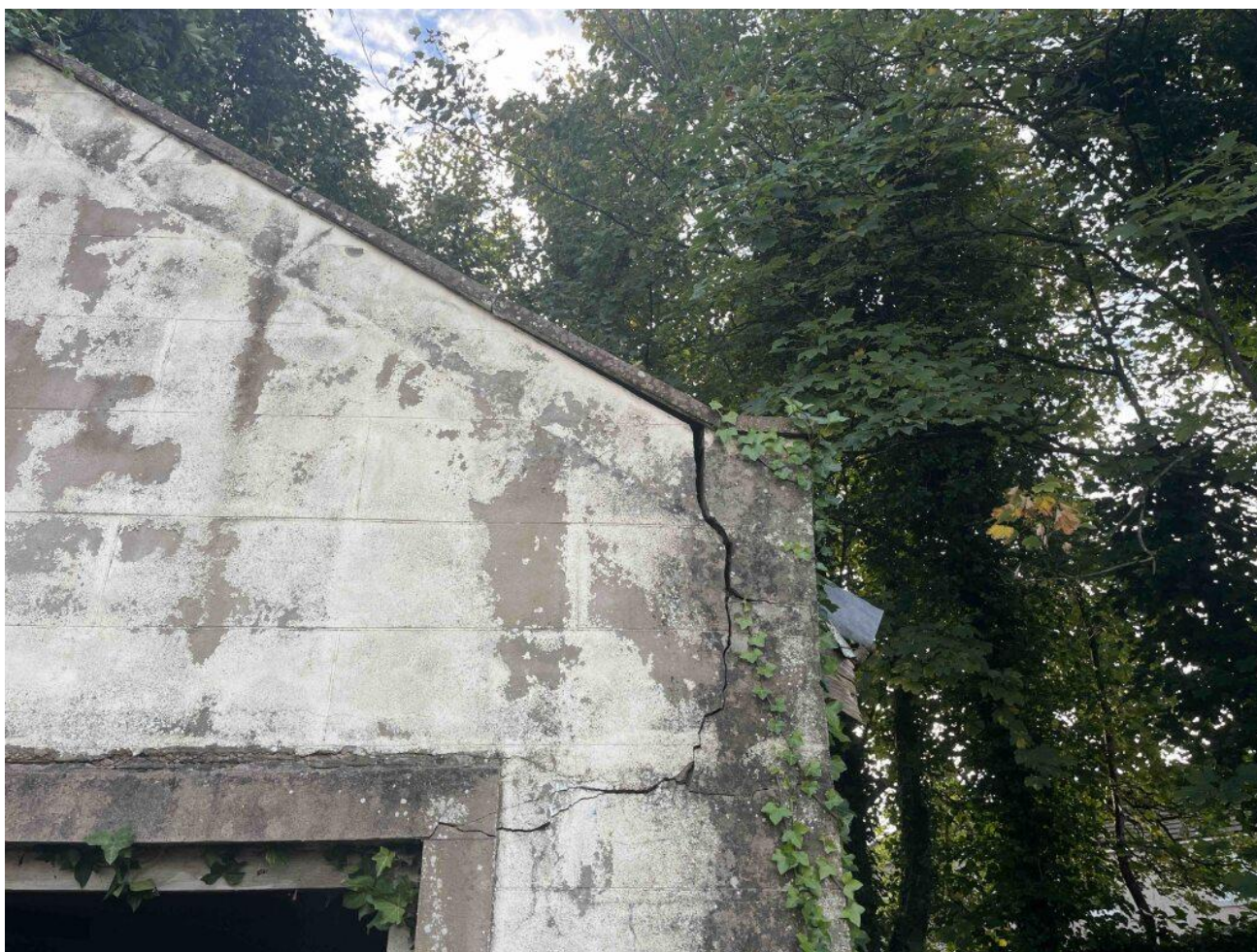
Image 9 – Crack on front aspect
