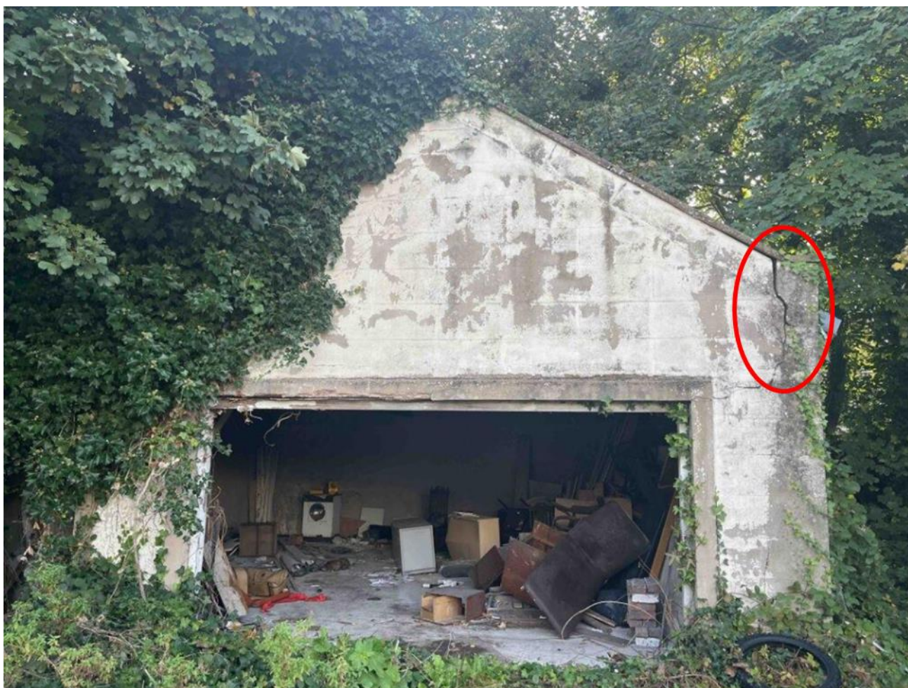
Image 4 – Front aspect of building with external damage circled
