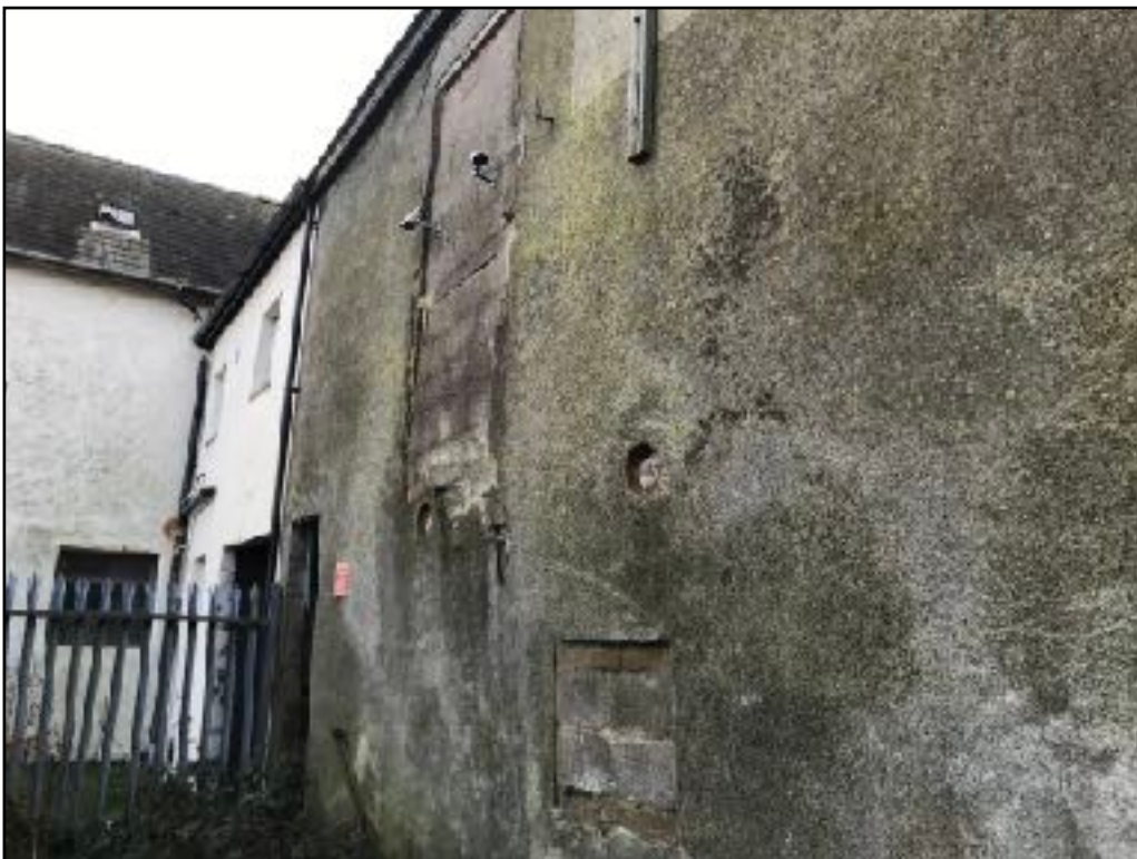
Figure 5: Showing the dilapidated barn which adjoins a neighbouring property on Hensingham Court in the north east corner of the site. This building offers 'low' bat roost potential and requires a dedicated bat survey.
