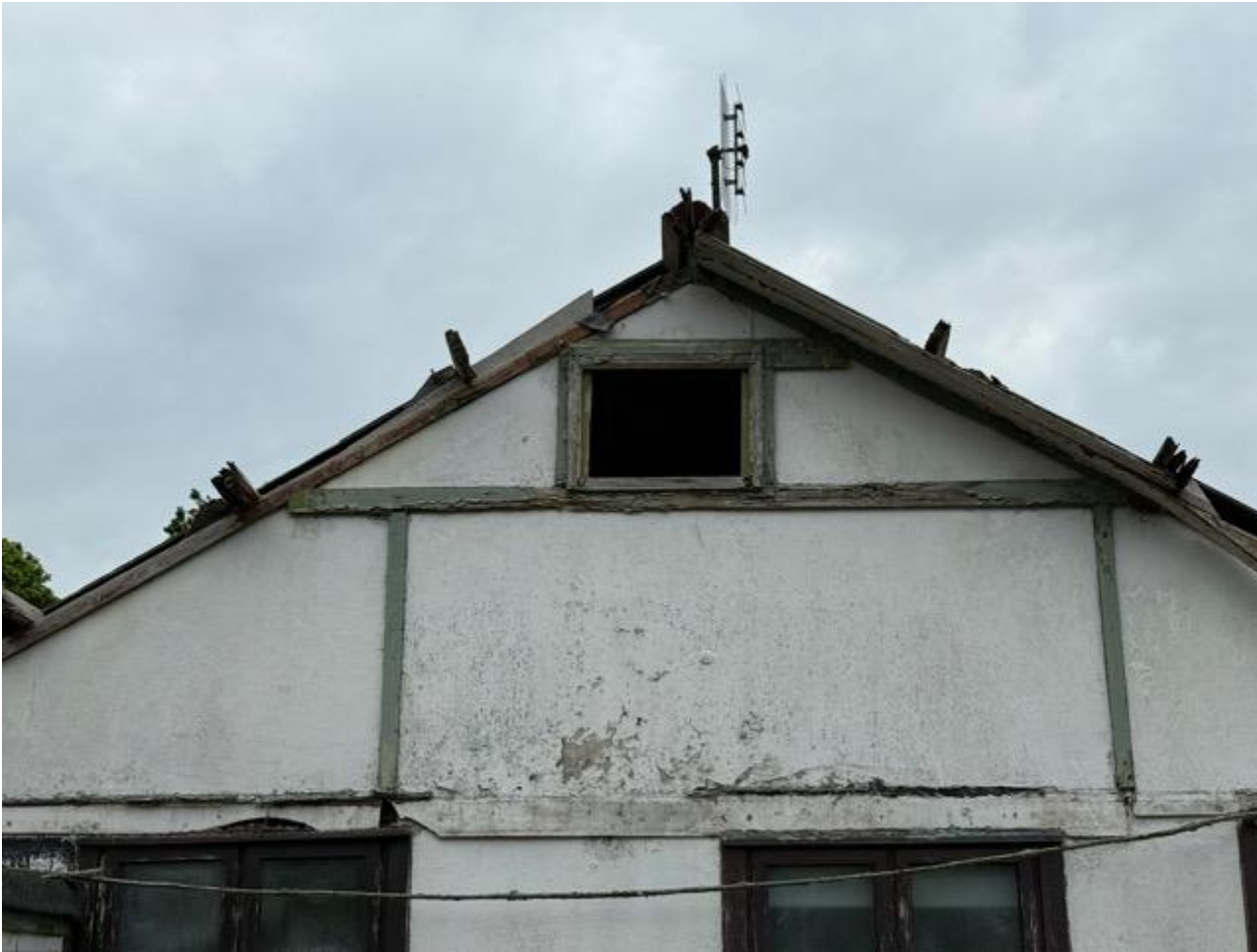
Photo 4: Opening present to roof void present on western elevation of B1.
