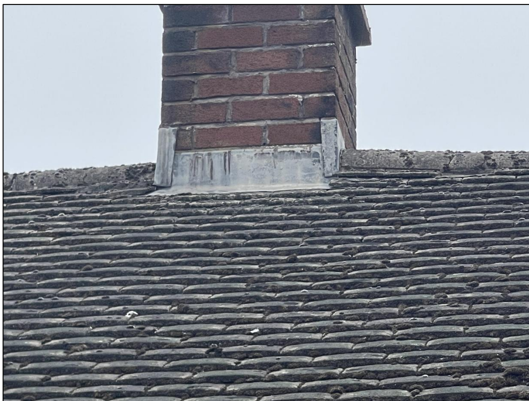
Plate 6 – Minor lifted tiles of B1 around chimney
