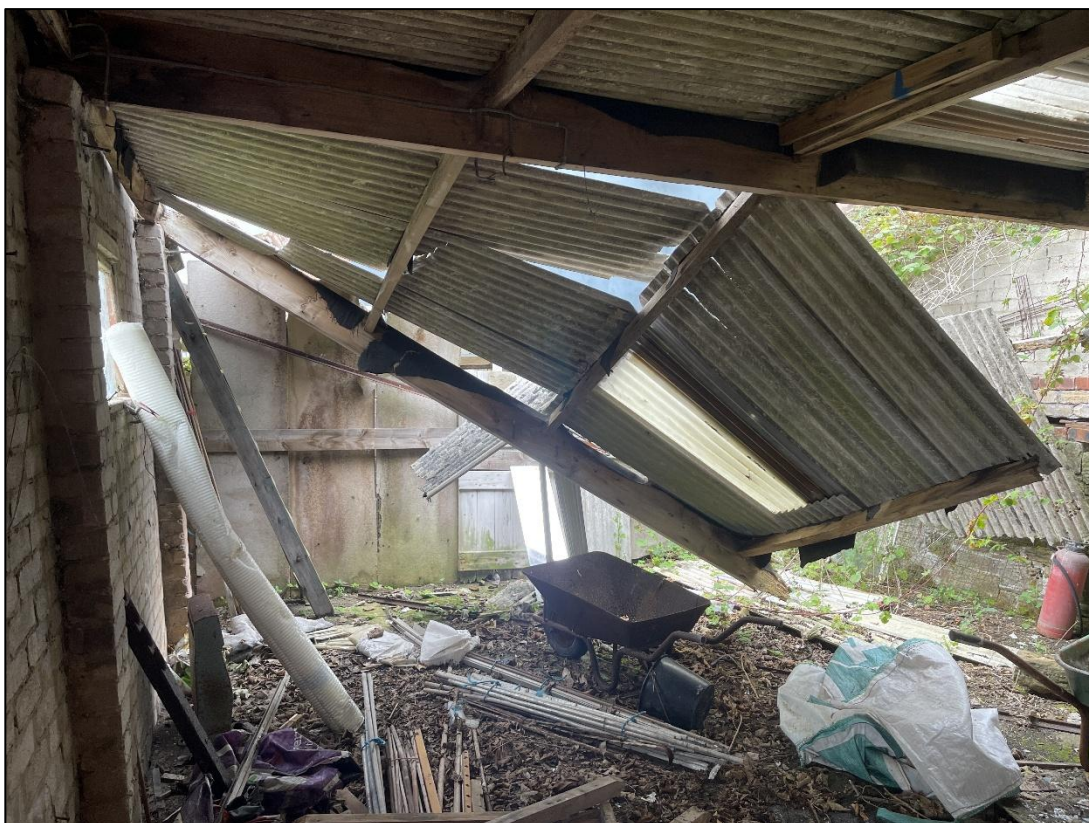
Plate 10 – Interior of B2, note collapsed roof
