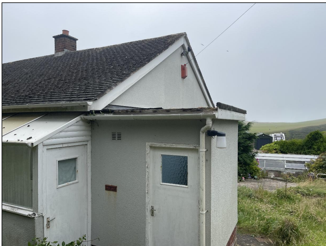
Plate 3 – Degradation to northern extension of B1
