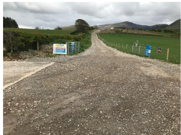
Hard standing and track looking easterly. Track means stock and machinery can safely be moved without having to use road.
