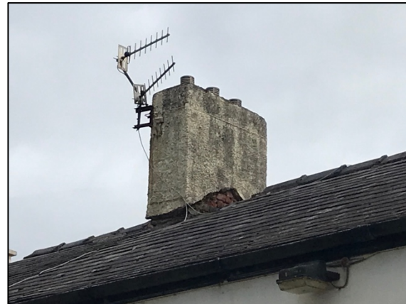
10. Detail of chimney to the gable end of 10 North Street with exposed brickwork indicating that the roof profile has been lowered.
