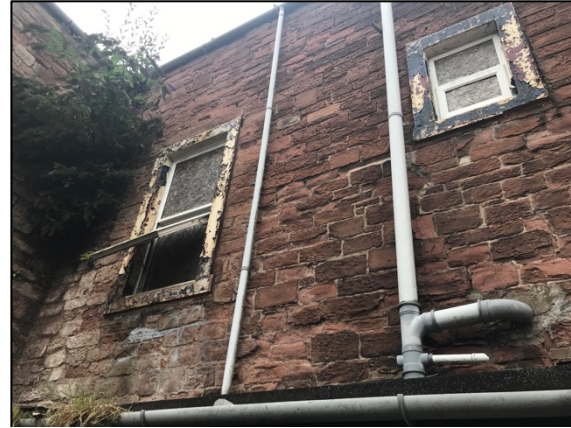
8. Detail of painted stone window surrounds, a typical vernacular building detail in the former county of Cumberland.
