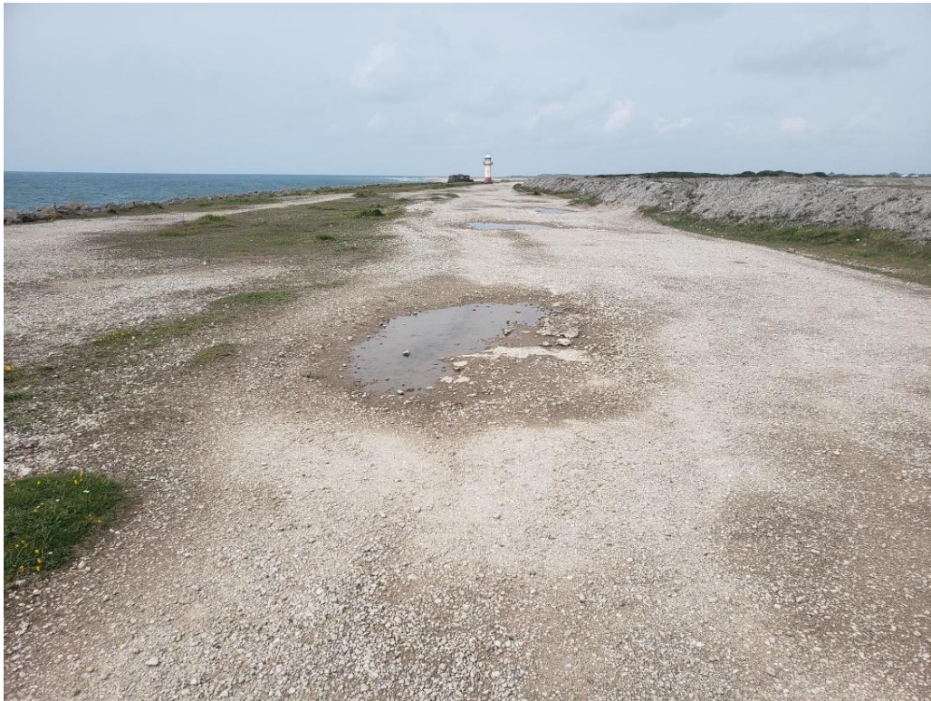
Plate 4.1 The BOAT along the sea wall. The darker areas show vegetated habitats of importance which will be protected during the works.
