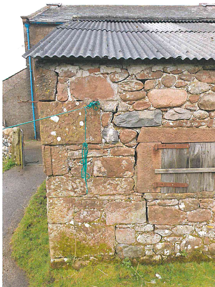
PHOTOGRAPH 02 VIEW ON CRACK TO REAR CORNER
