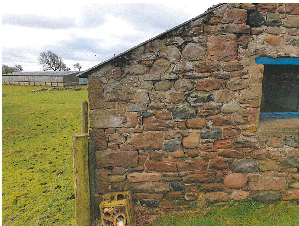
PHOTOGRAPH 01 VIEW ON LEFT AND GABLE CRACKING
