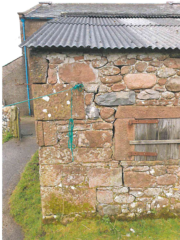
PHOTOGRAPH 02 VIEW ON CRACK TO REAR CORNER
