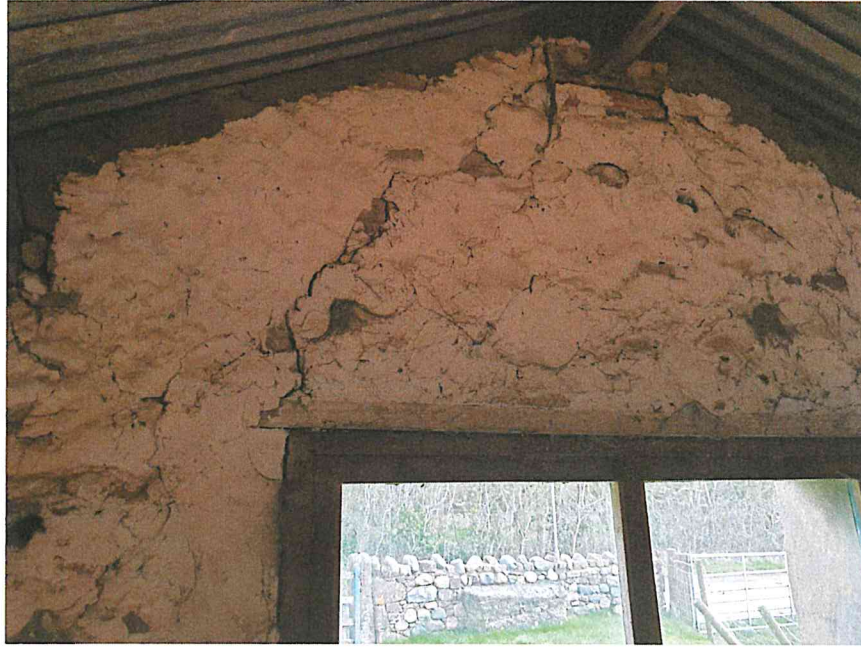
PHOTOGRAPH 03 VIEW ON GABLE LINTEL & CRACKING
