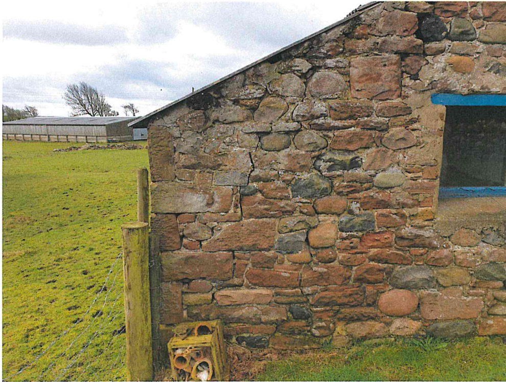
PHOTOGRAPH 01 VIEW ON LEFT AND GABLE CRACKING
