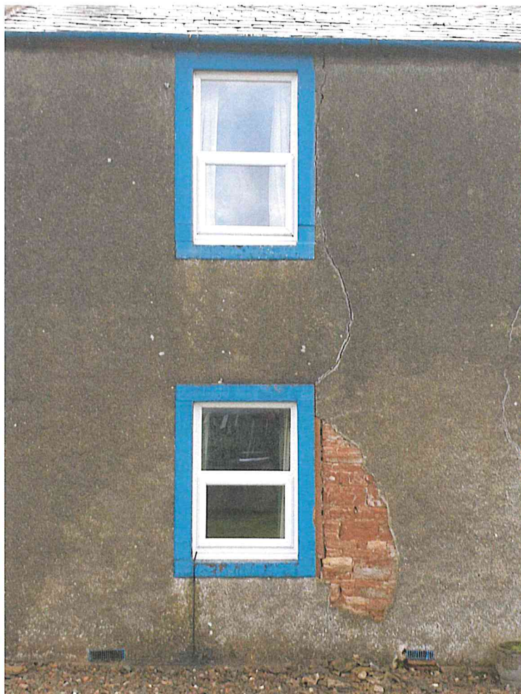
PHOTOGRAPH 02 VIEW ON CRACK TO FRONT ELEVATION
