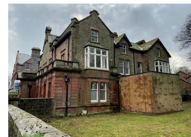
FIG 09 Elevations of existing building showing dilapidation.
