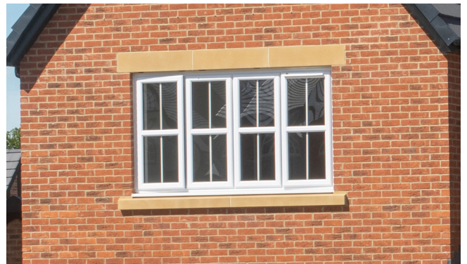
Buff cast concrete heads & cills
