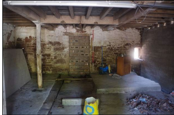
Figure 24. Defunct Bay 2, Room 2
