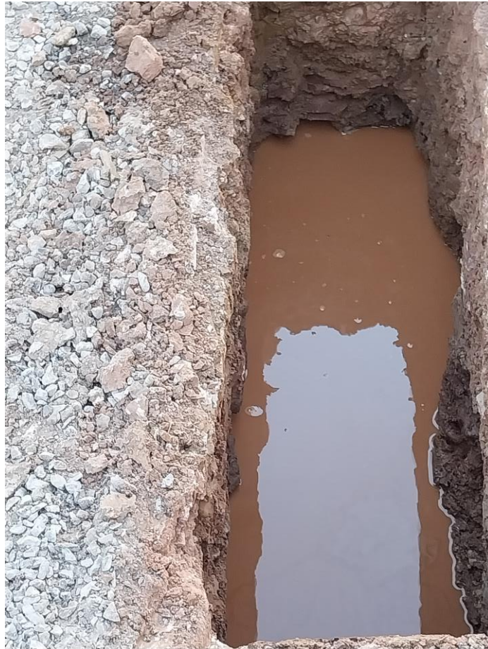
PHOTO 02 PIT WITH 0.8M DEPTH OF WATER
