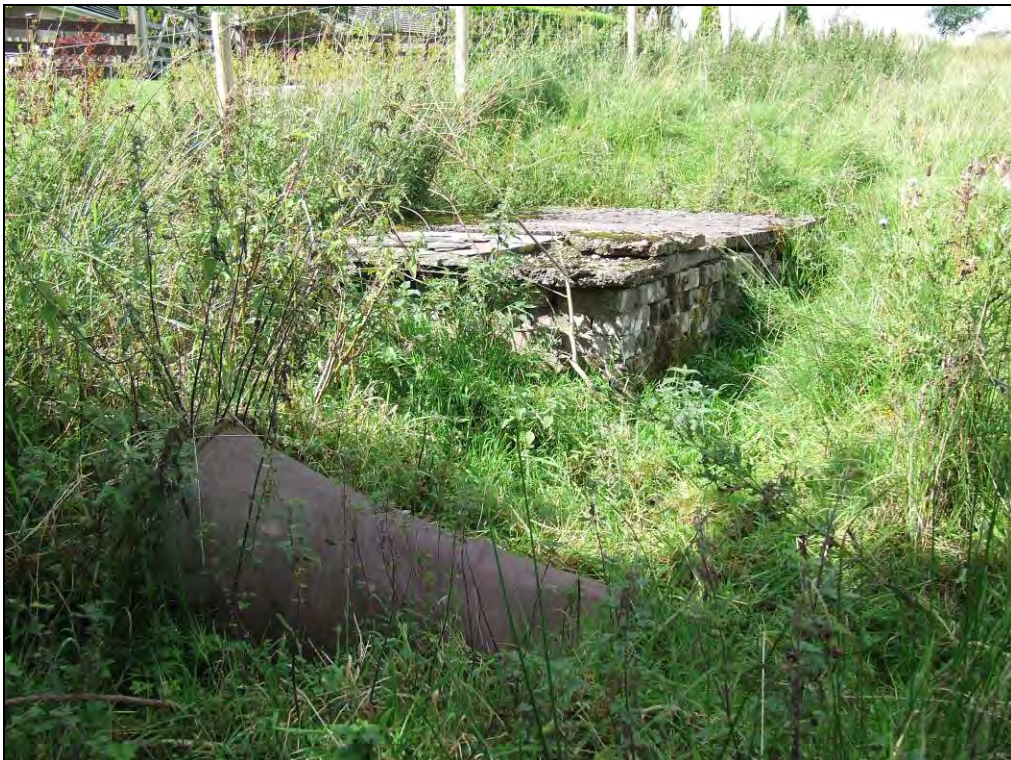
Photo 22: Site Interior – Old partially buried rusted metal drum located in the south western corner of the site near the brick tank shown on photo 21
