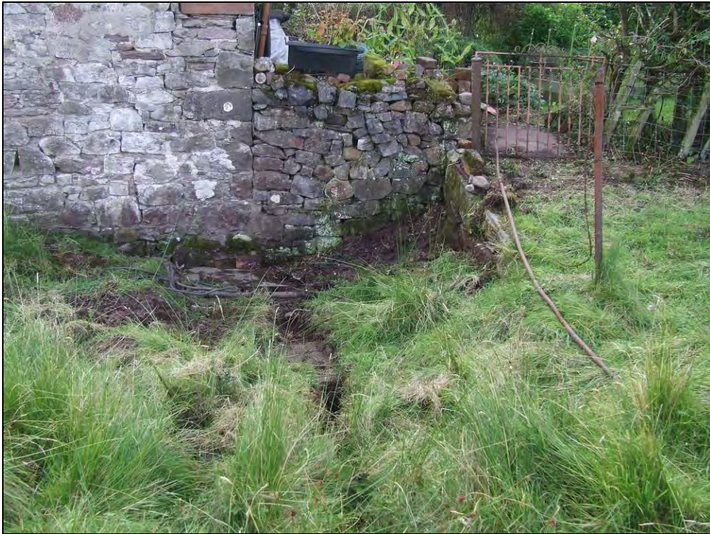
Photo 19: Site Interior – Small issue of water shown on photo 18, showing path of stream flowing south towards edge of outbuilding on southern site boundary, but disappearing beneath stone slab (centre)
