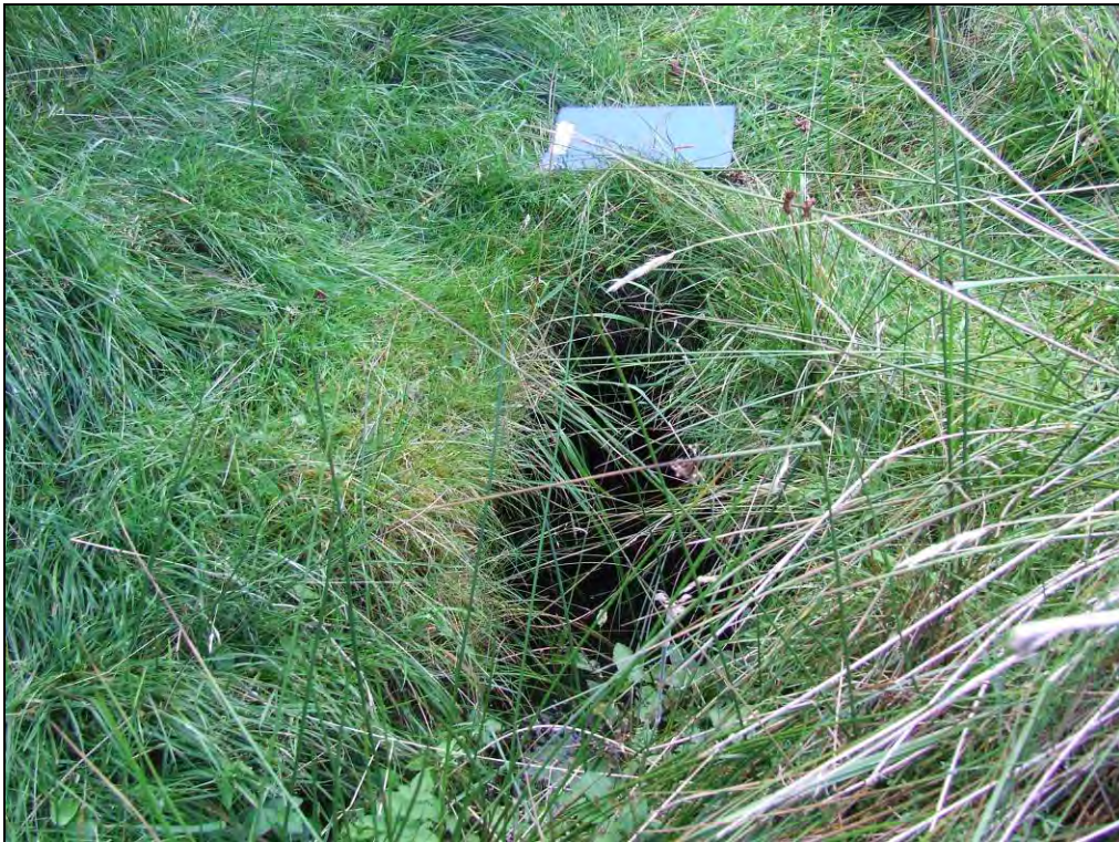
Photo 14: Site Interior – Small issue of water from the low lying area of land and near the eastern site boundary. The stream is believed to flow into the culvert extending beneath Kirkland Road
