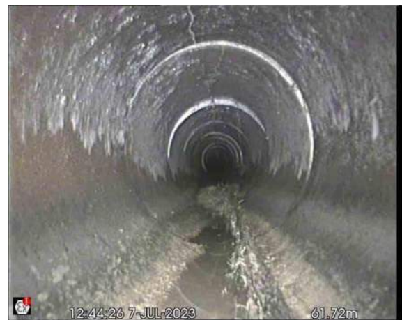
S1X_0da77cd8-fcb1-4675-a079-829a03bf0231_20230712_153819_414.jpg, 00:04:43, 61.72 m Crack, longitudinal at 11 o'clock
