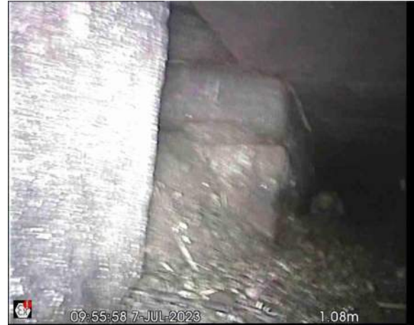
Culvert 1X_1094904e-3591-43dd-b28d-2fe7ede5a29a_20230712_15 3001_075.jpg, 00:00:16, 1.08 m General photograph taken at this point, connecting culvert from the left ???
