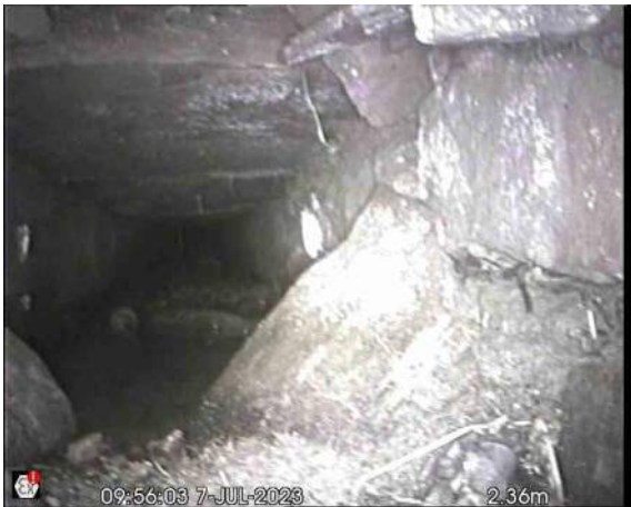
Culvert 1X_86003402-d99d-4b76-9c86-e92dd74b784f_20230712_152 825_223.jpg, 00:00:21, 2.36 m Other obstacles, other object in invert from 03 o'clock to 07 o'clock, 30% cross-sectional area loss, displaced stone
