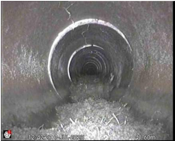
S1X_e2f99fed-5821-4776-9c9e-a2e1b8bafd3b_20230712_153748_131.jpg, 00:02:43, 41.60 m Crack, longitudinal at 01 o'clock, start
