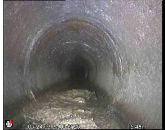
UpstreamX_16a7884a-b1a9-40ba-a95e-05f619c9b81d_20230712_152100_901.jpg, 00:01:14, 15.48 m Settled deposits, fine, 20% cross-sectional area loss
