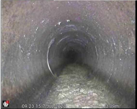
UpstreamX_1f9e9eba-3129-4080-a726-869b478841a0_20230712_152033_962.jpg, 00:00:27, 0.00 m Settled deposits, fine, 10% cross-sectional area loss, start
