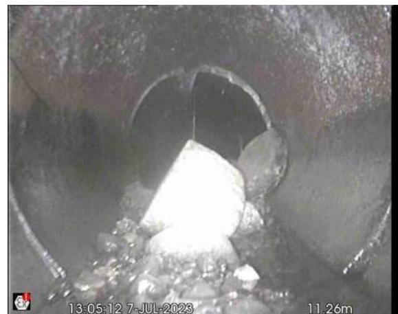
S1aX_ef45af67-820c-429f-b1af-b6abd90ddd0a_20230712_154306_174.jpg, 00:00:46, 11.26 m Other obstacles, other object in invert from 03 o'clock to 09 o'clock, 50% cross-sectional area loss, brick
