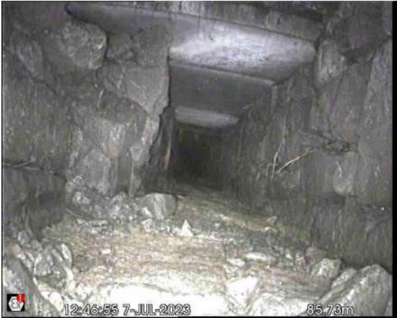
S1X_467947fe-245f-42d2-9d27-58a3b9efde16_20230712_15 4112_037.jpg, 00:07:12, 85.73 m Pipe size changes, new size(s), 350mm high, 380mm wide, changes to stone culvert
