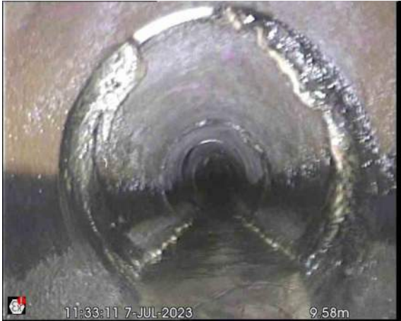
S3X_f0026768-a756-481a-9617-00cbd74a359b_20230712_155246_863.jpg, 00:00:48, 9.58 m Attached deposits, encrustation at joint from 12 o'clock to 12 o'clock, 10% cross-sectional area loss, Through out length of pipe
