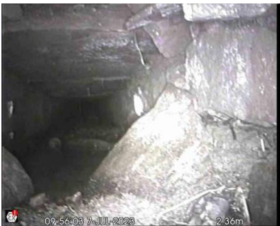
Culvert 1X_86003402-d99d-4b76-9c86-e92dd74b784f_20230712_152 825_223.jpg, 00:00:21, 2.36 m Other obstacles, other object in invert from 03 o'clock to 07 o'clock, 30% cross-sectional area loss, displaced stone
