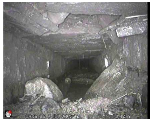
Culvert 1X_18759280-8c50-49a7-812e-a6b0ab322bbd_20230712_15 2834_768.jpg, 00:00:21, 2.36 m Other obstacles, other object in invert from 03 o'clock to 07 o'clock, 30% cross-sectional area loss, displaced stone
