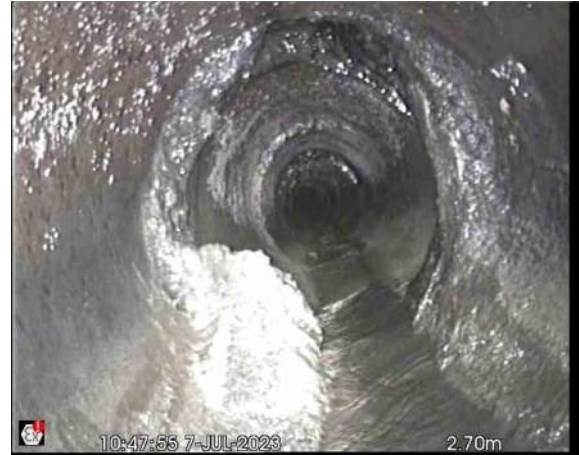
S1aX_85baacd2-e3dc-47e1-ad39-c863b252ea2d_20230712_154515_279.jpg, 00:00:53, 2.70 m Attached deposits, encrustation at joint from 12 o'clock to 12 o'clock, 20% cross-sectional area loss
