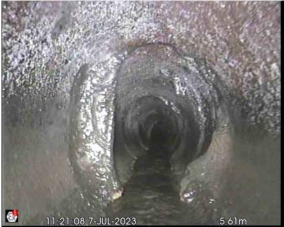
S2X_d35bcb8c-475d-49be-a2de-f415b27af1f6_20230712_154751_477.jpg, 00:00:32, 0.00 m Attached deposits, encrustation at joint from 12 o'clock to 12 o'clock, 25% cross-sectional area loss, throughout pipe
