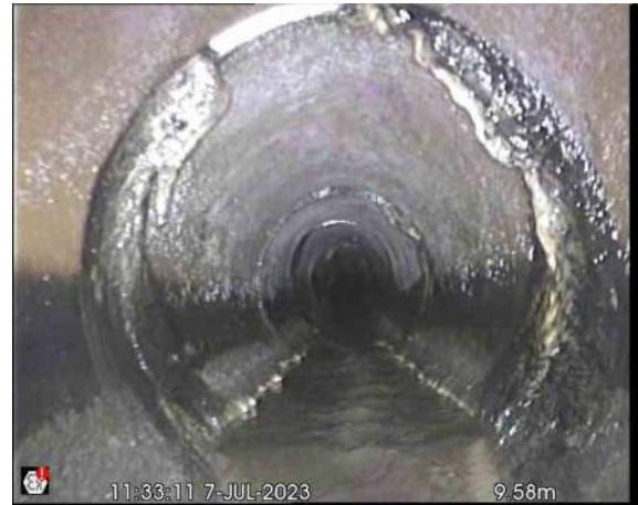
S3X_78760974-7af3-4e6e-be33-efc7330ed7c5_20230712_155451_998.jpg, 00:00:48, 9.58 m Infiltration, dripping at joint at 12 o'clock, through out pipe
