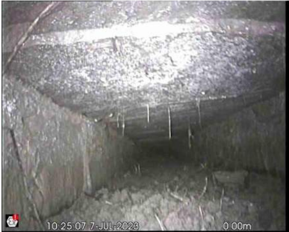
Culvert 2X_c420a4d8-6f79-4c9a-8500-59d2b430bae7_20230712_153 117_352.jpg, 00:00:07, 0.10 m Settled deposits, coarse, 15% cross-sectional area loss
