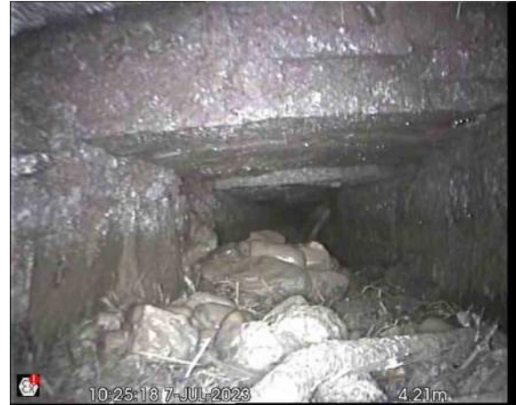
Culvert 2X_3d796954-06bb-49e0-85b5-42e8f7daafe1_20230712_153 133_483.jpg, 00:00:19, 4.21 m Settled deposits, coarse, 60% cross-sectional area loss
