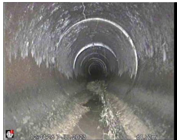
S1X_0da77cd8-fcb1-4675-a079-829a03bf0231_20230712_153819_414.jpg, 00:04:43, 61.72 m Crack, longitudinal at 11 o'clock
