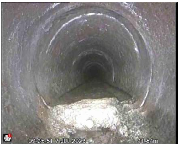
UpstreamX_d0f13ee9-871a-4629-ba44-8d6ef983a3a5_20230712_152448_915.jpg, 00:03:03, 41.64 m Other obstacles, other object in invert from 04 o'clock to 08 o'clock, 25% cross-sectional area loss
