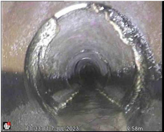
S3X_f0026768-a756-481a-9617-00cbd74a359b_20230712_155246_863.jpg, 00:00:48, 9.58 m Attached deposits, encrustation at joint from 12 o'clock to 12 o'clock, 10% cross-sectional area loss, Through out length of pipe
