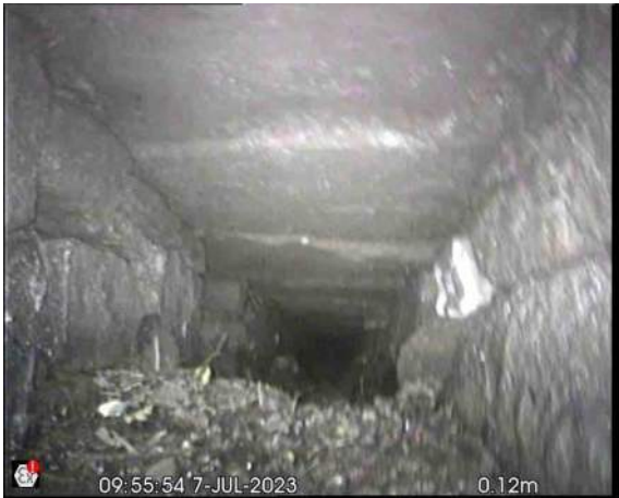
Culvert 1X_d6dfd373-dab2-499d-98f8-233d747fb44b_20230712_152 754_219.jpg, 00:00:13, 0.12 m Settled deposits, fine, 25% cross-sectional area loss
