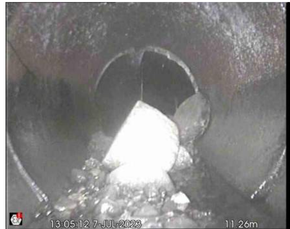
S1aX_ef45af67-820c-429f-b1af-b6abd90ddd0a_20230712_154306_174.jpg, 00:00:46, 11.26 m Other obstacles, other object in invert from 03 o'clock to 09 o'clock, 50% cross-sectional area loss, brick
