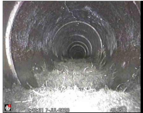
S1X_45acfc27-6d4f-4806-ab6a-398c2d1aa1b4_20230712_153627_751.jpg, 00:02:48, 43.05 m Roots, mass, 20% cross-sectional area loss
