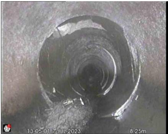
S1aX_454040a4-6254-4383-b57f-404792e38f38_20230712_154339_036.jpg, 00:00:37, 8.25 m Hole in drain or sewer from 11 o'clock to 01 o'clock
