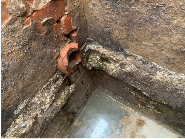
Fig 2, 3 and 4. Brick built, triple chamber septic tank.
