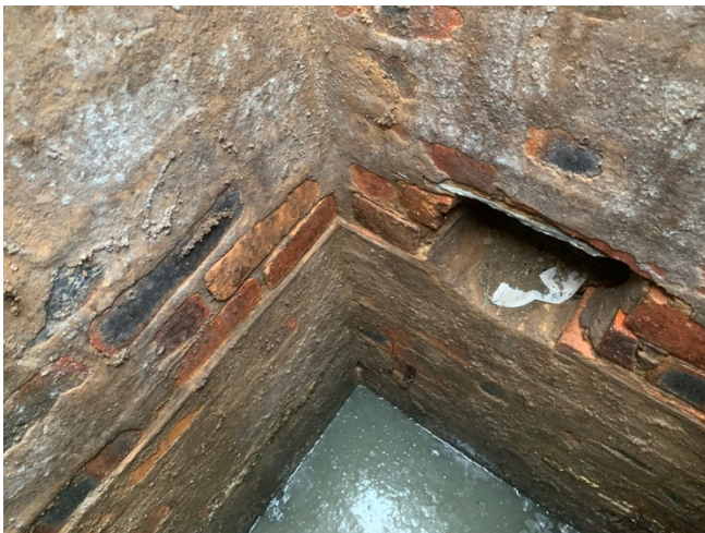
Fig 5. Liquid level below outlet pipe.
