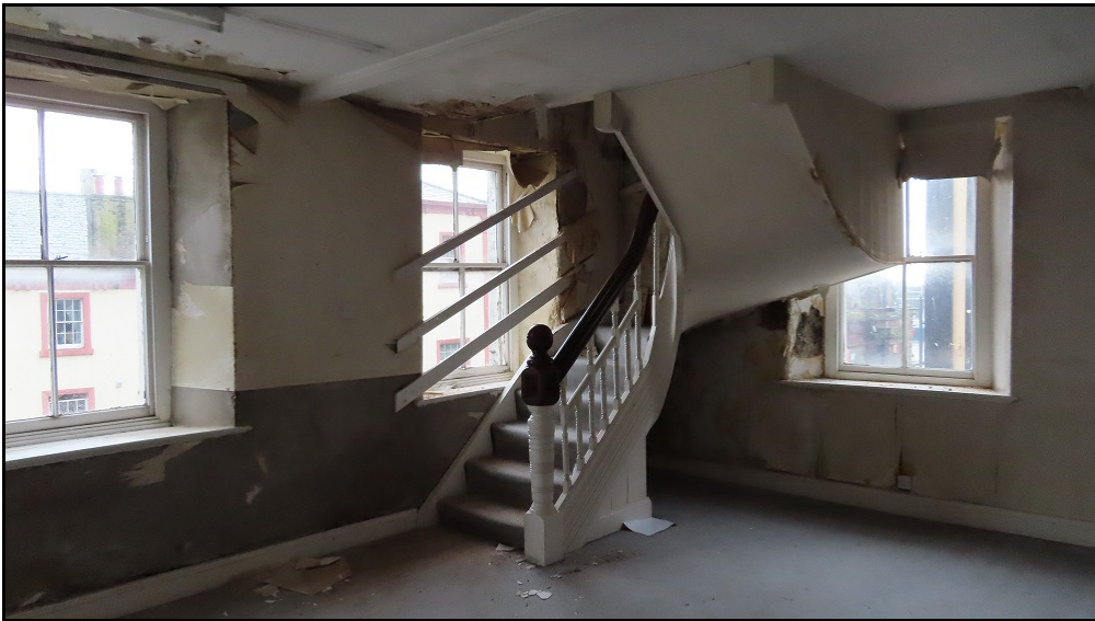
12. The surviving mid-Victorian staircase between first and second floors will be retained
