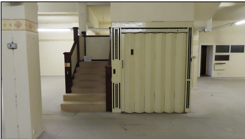
10. The gated lift and adjoining stair date from the early 1900's and will be retained
