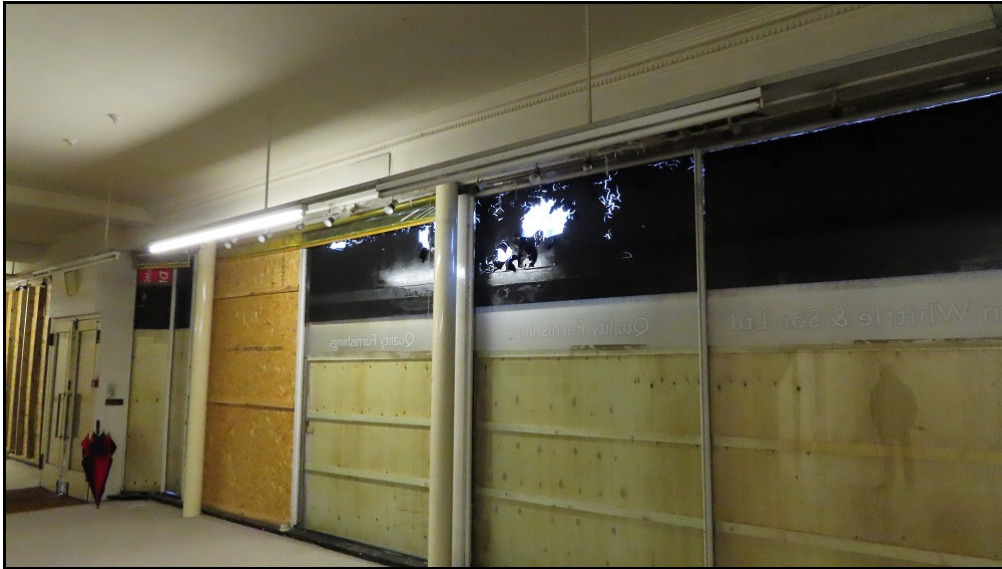
9. The steel columns that support the shop frontage date from the early 1900's and will be retained
