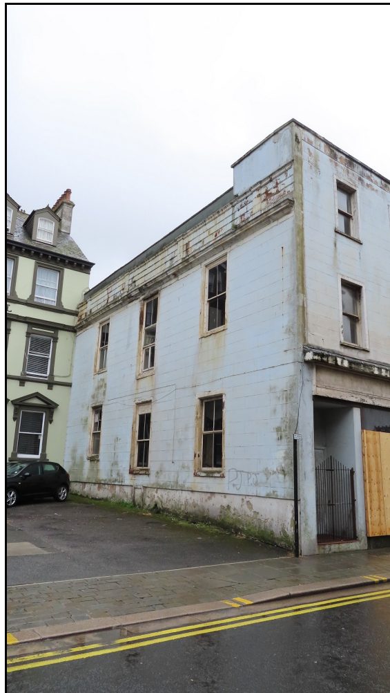
8. The view of the rear of the building from Tangiers Street with the Waverley Hotel adjoining
