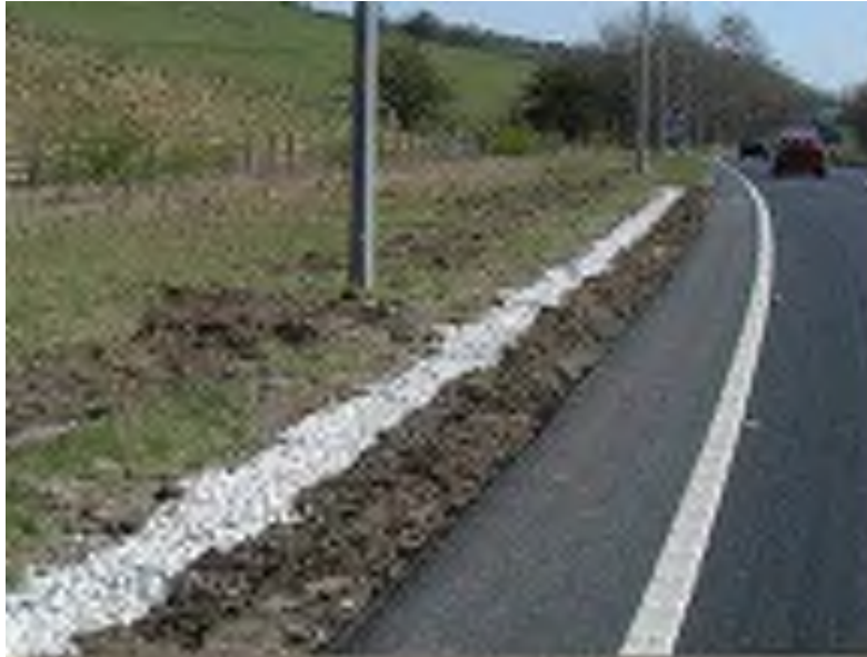
Photo showing edge of carriageway filter strip
