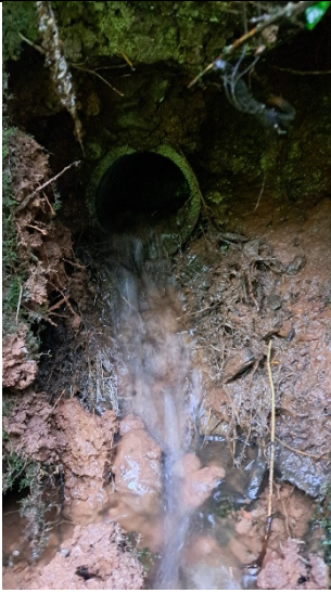
Pipe into cutting upslope of site (thought to connect to existing sewer)
