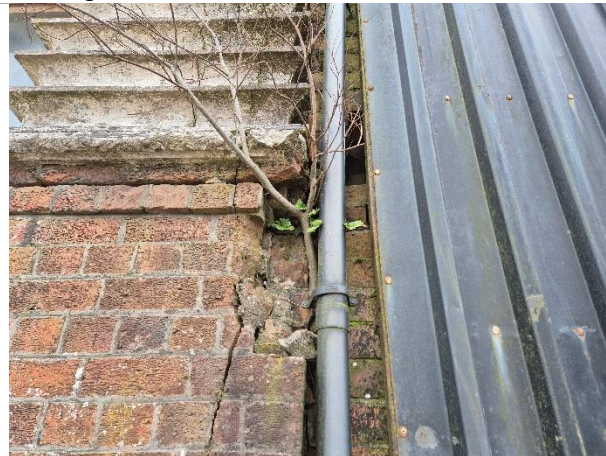
Photo 6: Gaps in external brickwork were inspected at height with an endoscope and torch; no bats or evidence of use by roosting bats. Gaps are damp owing to water ingress.
