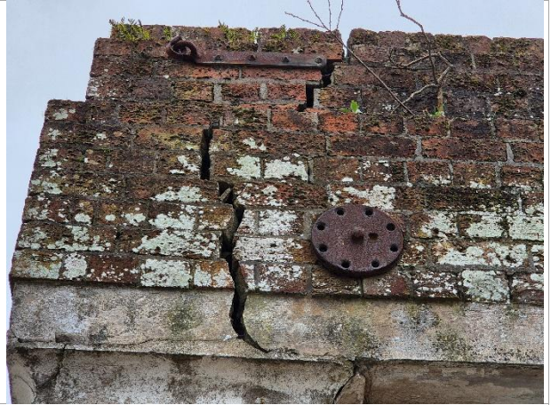
Photo 8: Gaps in external brickwork were inspected at height with an endoscope and torch; no bats or evidence of use by roosting bats. Gaps are damp owing to water ingress.
