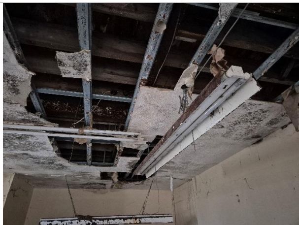
Photo 11: Ceiling beneath flat-roofed section; extensive areas of water ingress
