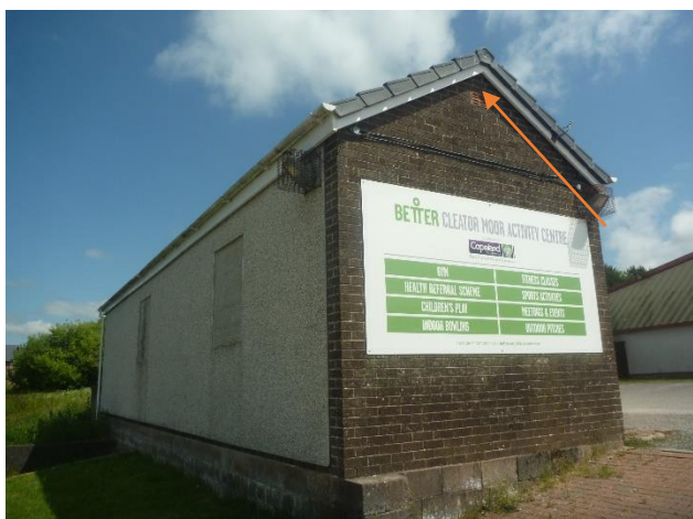
Photo 27: Building 2, south-western gable end, showing location where bat droppings were found internally (Roost 1)
