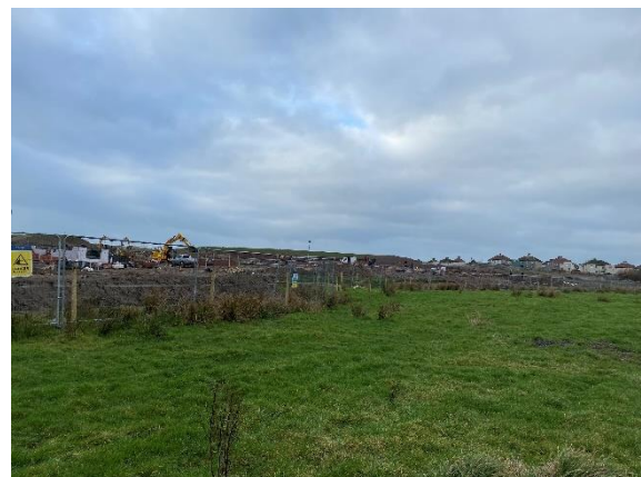
Photograph 17 – Area of construction site encroachment
