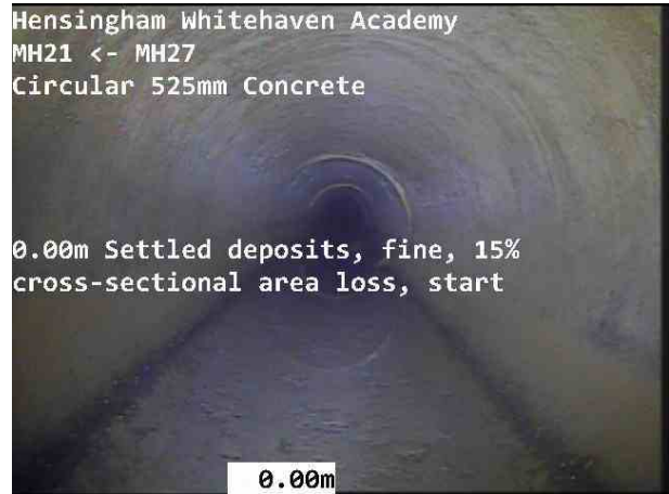
MH21X_0134eacd-9871-4a78-9401-57dceaa3e30f_20220622_153452_952.jpg, 00:00:06, 0.00 m Settled deposits, fine, 15% cross-sectional area loss, start
