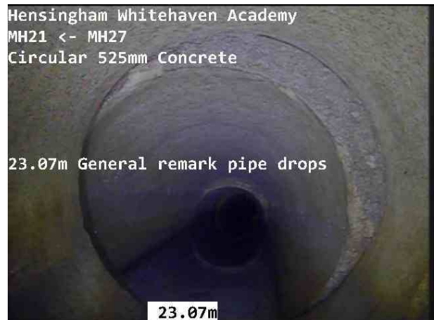
MH21X_7e59d3ce-88e2-4efb-8494-19a2d08cb071_20220622_153616_513.jpg, 00:03:18, 23.07 m General remark, pipe drops
