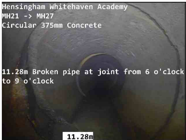
MH21X_1ef3ecfa-3af1-44f4-ad44-7e9d1b8603e4_20220622_153716_635.jpg, 00:01:11, 11.28 m Broken pipe at joint from 6 o'clock to 9 o'clock
