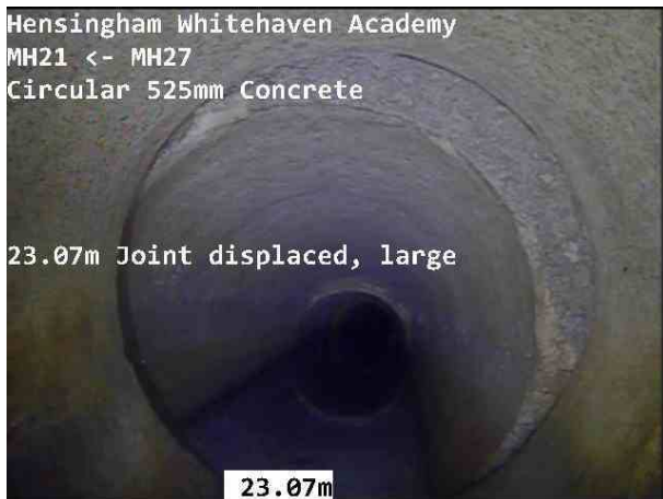
MH21X_57a3cae3-a014-41c0-bd47-c7d6fe2c8a72_20220622_153612_461.jpg, 00:03:14, 23.07 m Joint displaced, large
