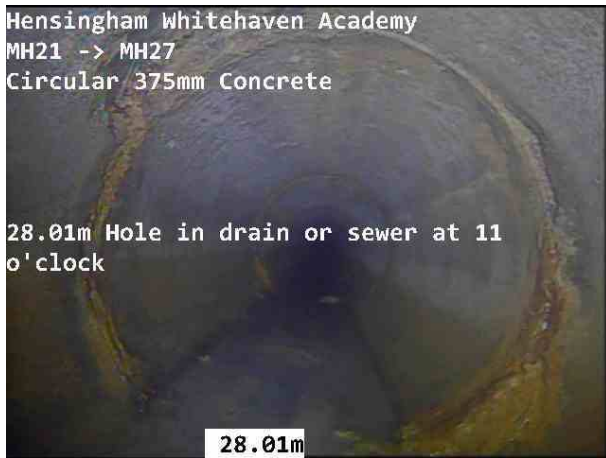
MH21X_93253561-1162-4ec8-9cdb-99992a037ac8_20220622_153731_878.jpg, 00:02:24, 28.01 m Hole in drain or sewer at 11 o'clock
