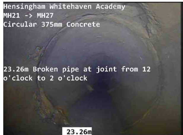
MH21X_bd9c0086-9608-4a43-b255-08ca5241b232_20220622_153724_203.jpg, 00:01:59, 23.26 m Broken pipe at joint from 12 o'clock to 2 o'clock
