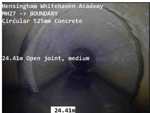
MH27X_7e87f2c5-7157-4a47-8fbf-ca90e7f55776_20220622_153645_124.jpg, 00:05:15, 24.41 m Open joint, medium
