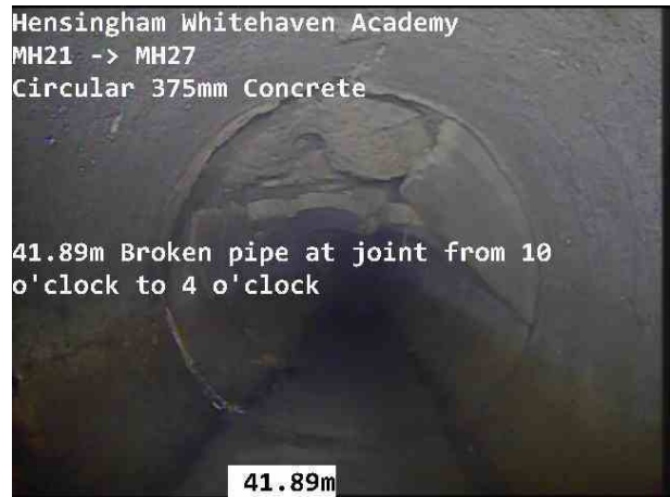
MH21X_06554e84-0b61-4b9d-8768-af657374f4f4_20220622_153739_665.jpg, 00:03:23, 41.89 m Broken pipe at joint from 10 o'clock to 4 o'clock
