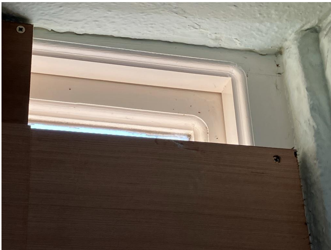
Close up photo of rear window - Internal view confirms this is a modern factory made window with routed curved edges confirming this. Window is temporary boarded due to vandalism
