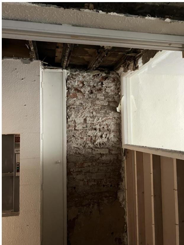
Rear half of front room in Apartment 2 ground floor, exposed brick aligns with chimney stack on first floor and basement.
