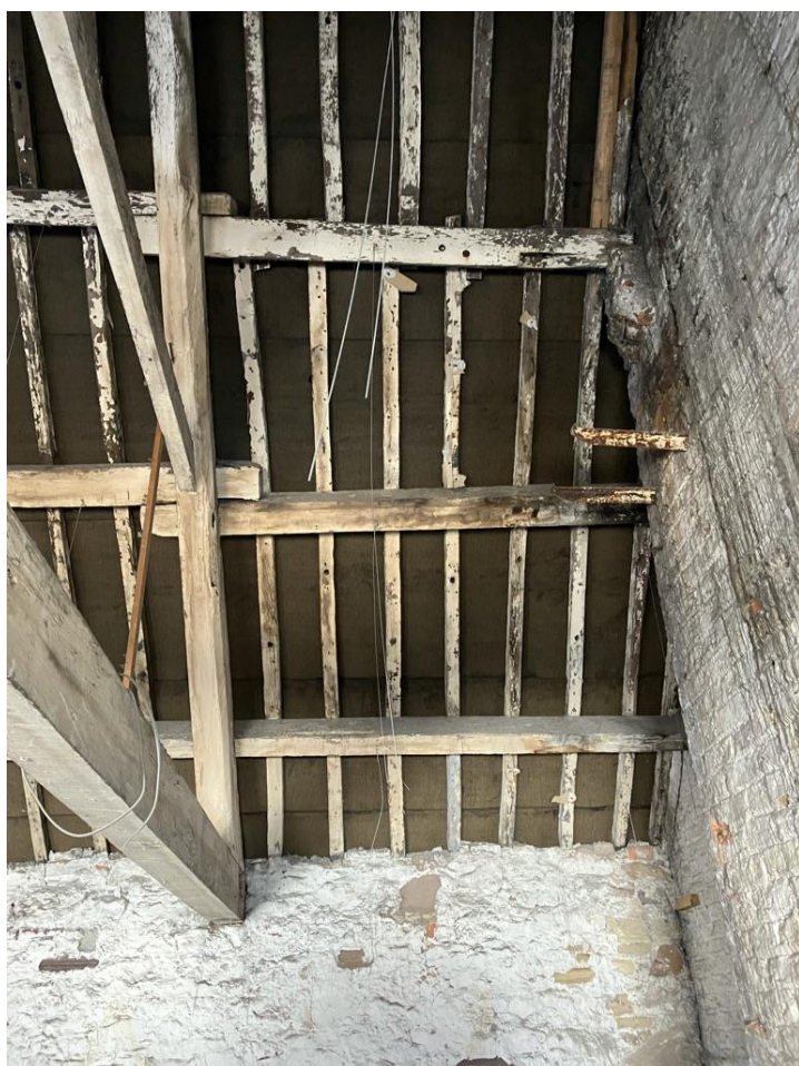
Location of attic stairs to right hand gable of existing roof structure.
