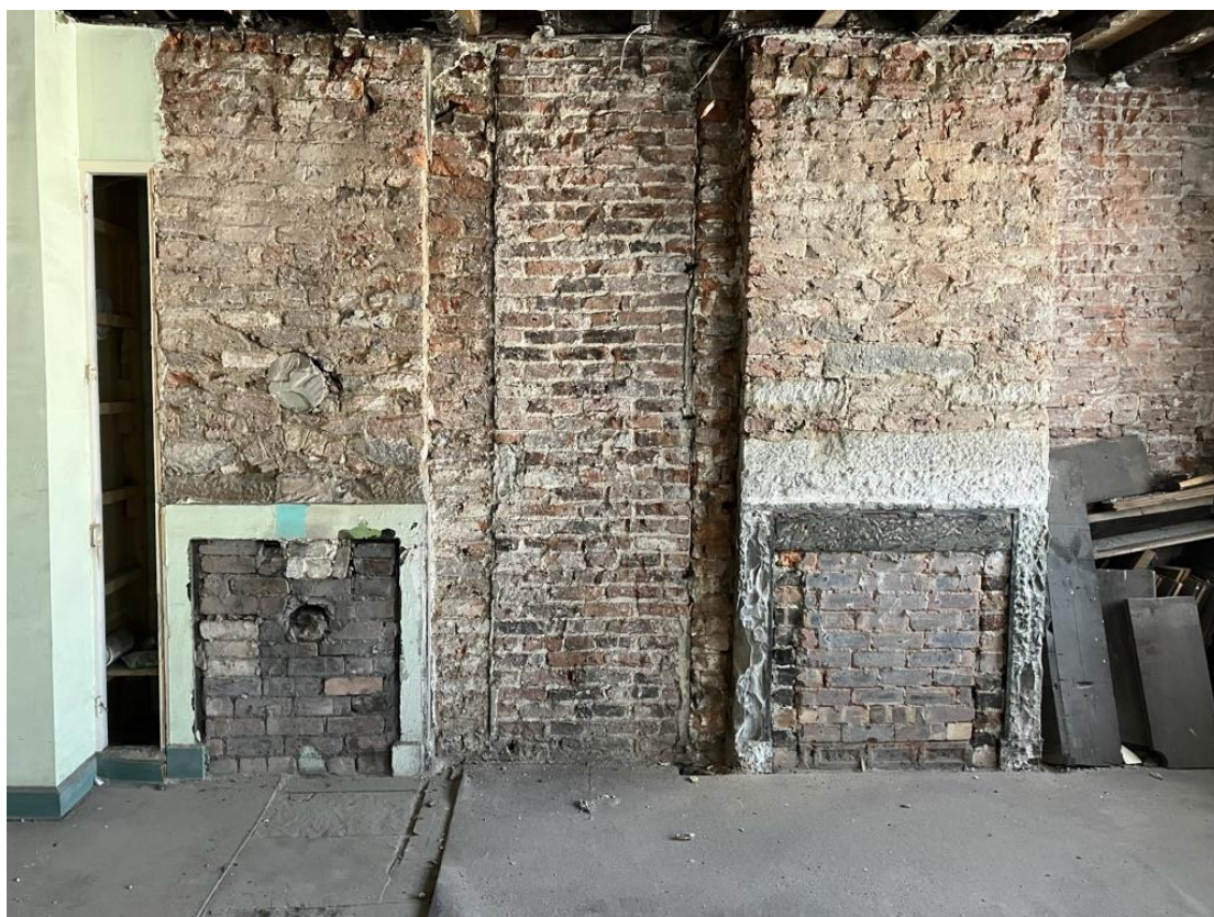
Chimney stack at first floor gable with central stack shown centrally between, and serves fireplace in ground floor of apartment 2.
