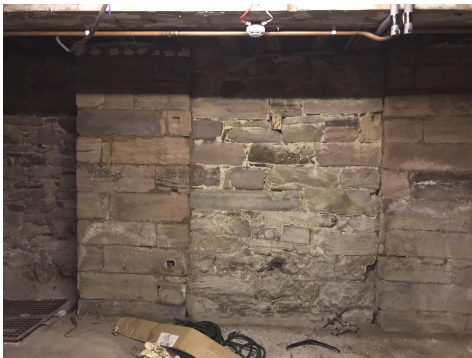
Basement gable wall viewing towards adjacent property – Basement stonework indicates the alignment of two chimney stacks within the building which rise through three floors. Central infill of stone is referenced on upper two floors.
