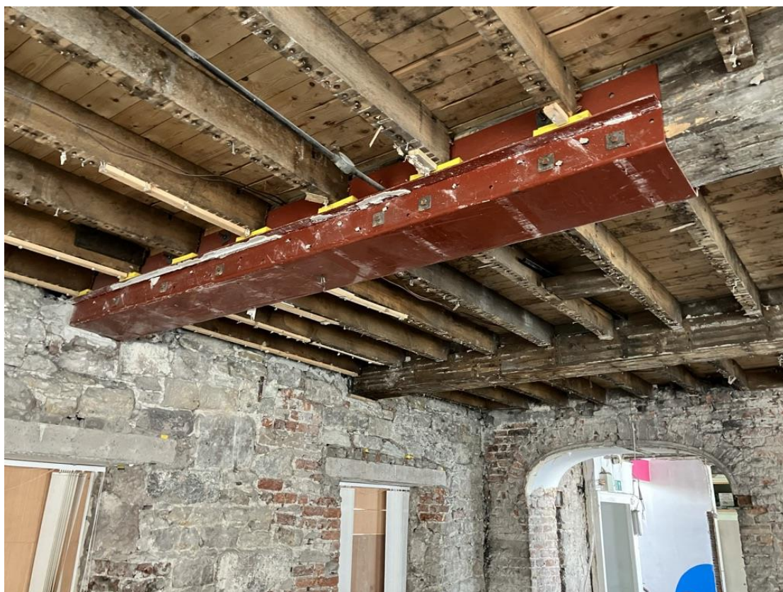
First floor ceilings with previously installed steel strengthening by previous building owner. This also indicates modern floor joists and floor boards installed within the last 50 years.
