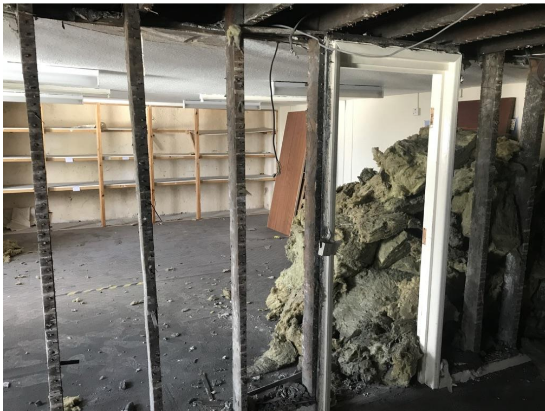
Thermal insulation removed from roof voids to allow inspection of the existing timbers
