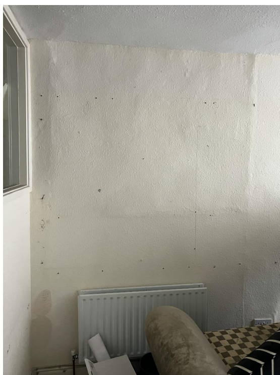
Apartment 2 – assumed former fireplace location sat centrally between two existing chimney stacks and remains unaltered. Profile of two distinct chimney stacks to left and right hand side visible in plaster profile. No works are proposed to this chimney stack with the except of inserting an air brick for ventilation.
