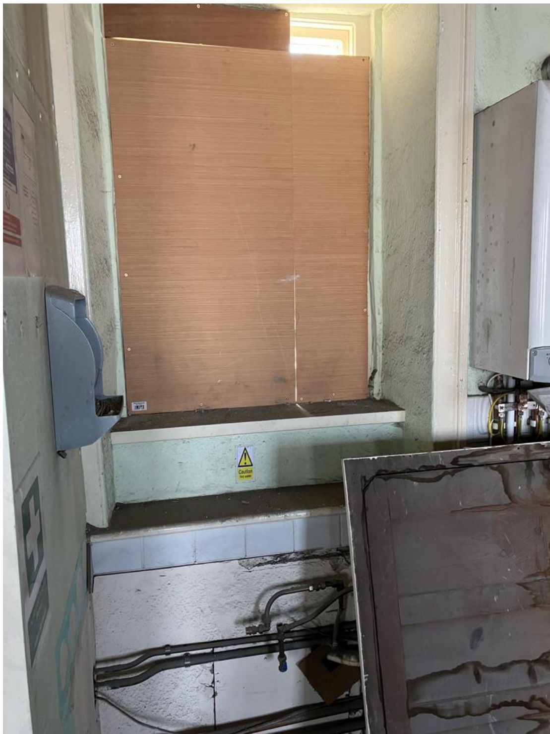
Internal view of window indicating a modern raised cill to allow kitchen to be installed. Wooden timber beads to plasterwork remain and architrave to window reveal
