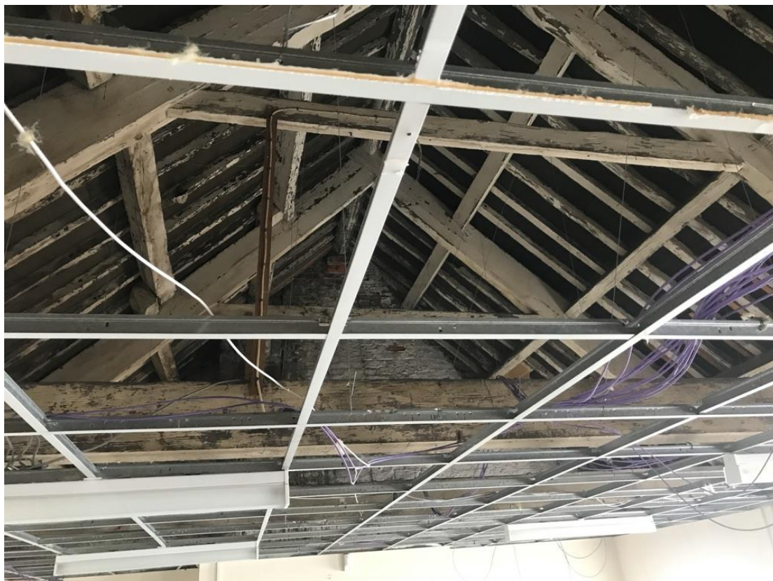
Sample photograph of second floor attic level which reflected the majority of floors where existing plastered or lath and plastered ceilings had all been previously removed and timbers all covered with thermal quilt insulation
