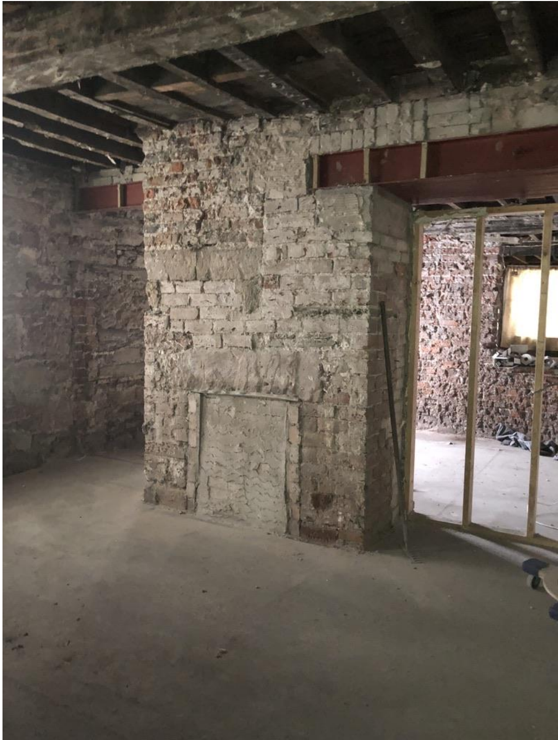
Modern steelwork and strengthening works to existing openings with new brickwork over.
