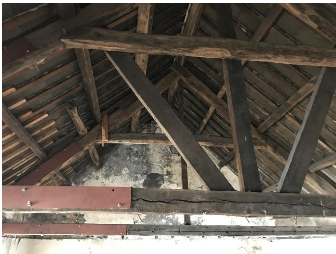
Previous steel strengthening works to roof trusses. Evidence of additional modern timber bracing also added to main trusses.
