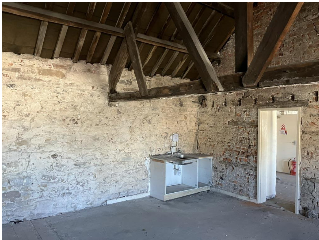
Location of attic stairs to left hand section of second floor – stairs fitted between truss and former 'party wall'
