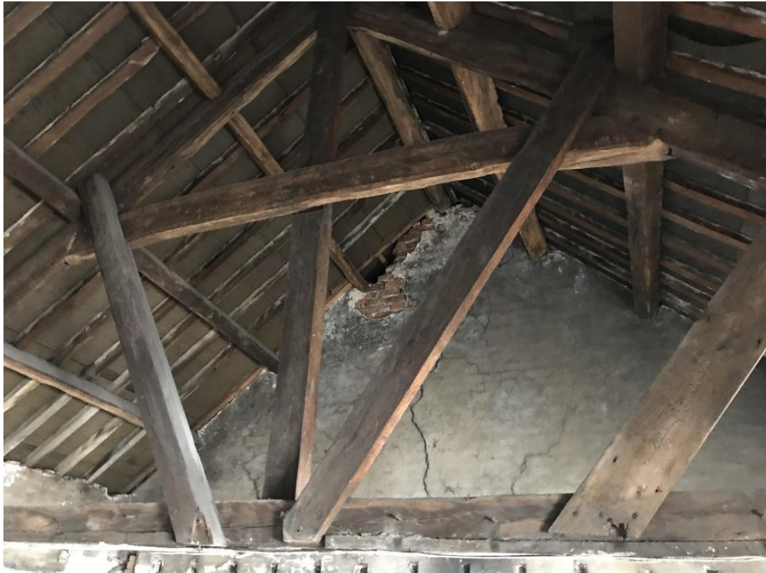
Original roof trusses within the second floor indicating additional strengthening and repairs
