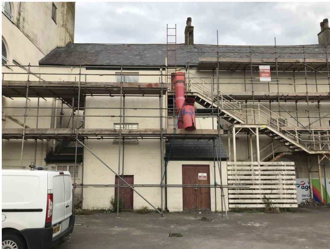
Rear elevation showing decayed steel staircase
