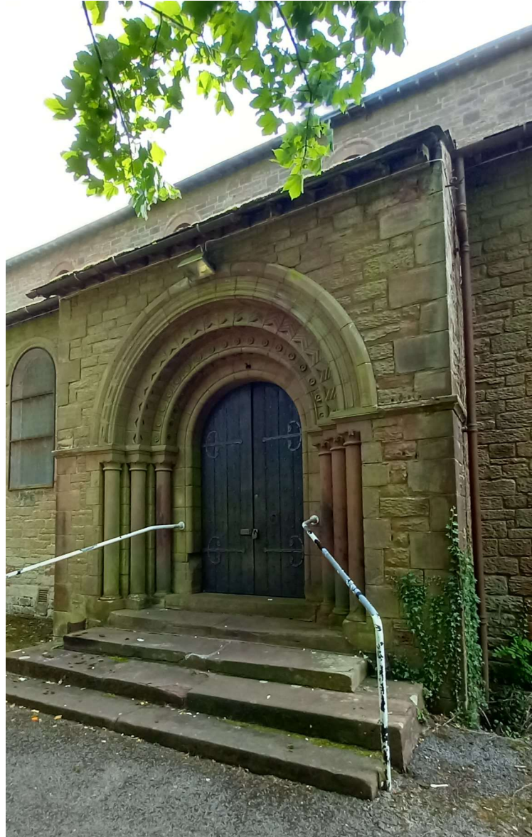
Fig. 7 - Existing stepped entrance. Existing steps to be removed. New access ramp to be constructed. Material removed from existing steps to be re-cycled in the construction of the new ramp and steps. To the right of the above image an existing rainwater downpipe can be seen. The addition of the ramp will raise the ground level in the location of this rainwater downpipe and as a result the gully will need to be raised to the new level.
