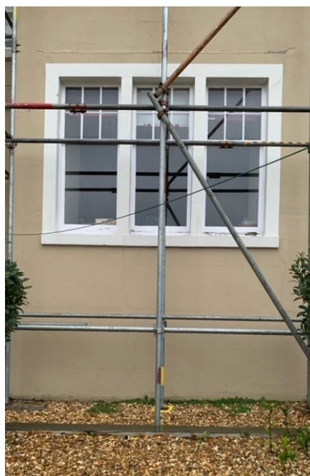
Photo1: View of the section of the southwestern side wall of the rear annexe below the ground floor kitchen window
