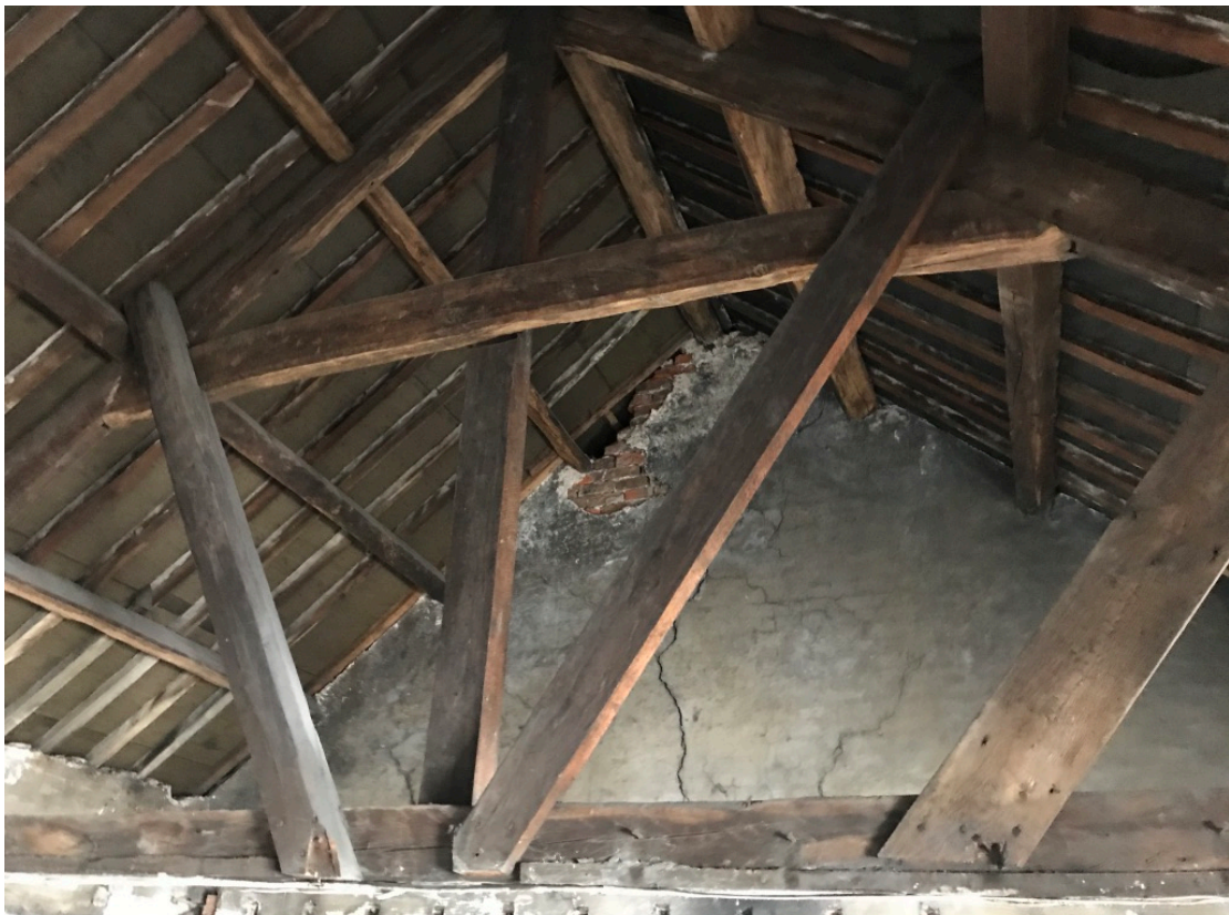
Original roof trusses within the second floor indicating additional strengthening and repairs
