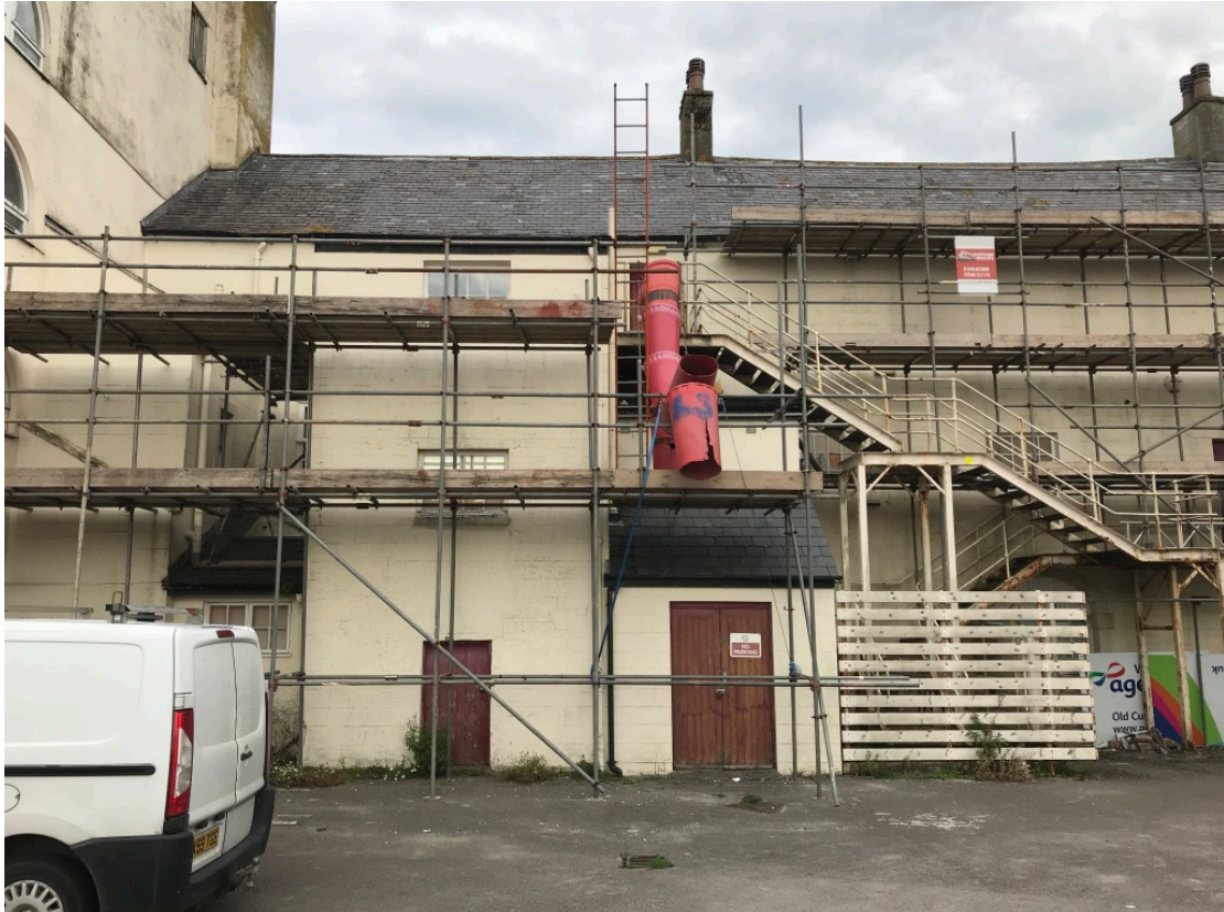
Rear elevation showing decayed steel staircase
