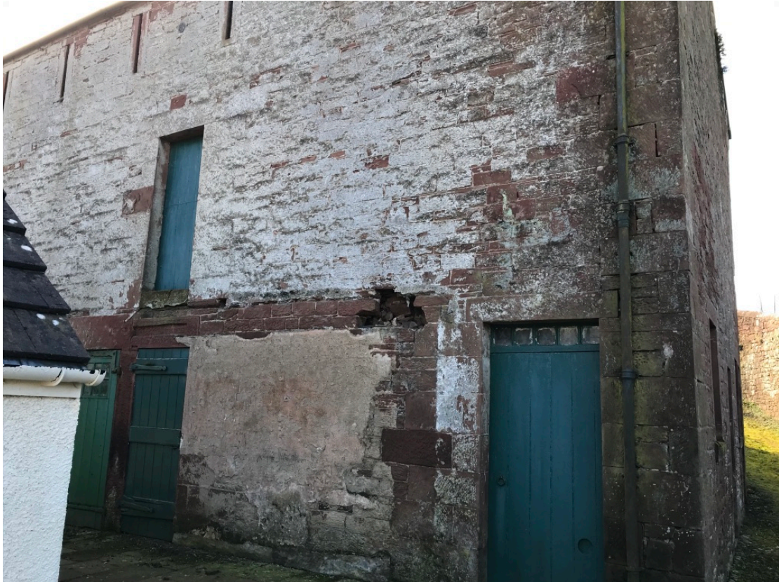
Part front elevation obscured by garage with evidence of modern lean to buildings
