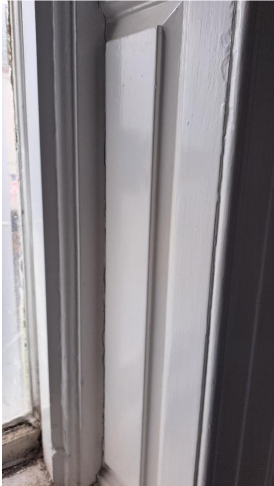
Figure 7 Panelling to upper floor window. Has the panelling been cut or is the secondary glazing surround scribed to it?
