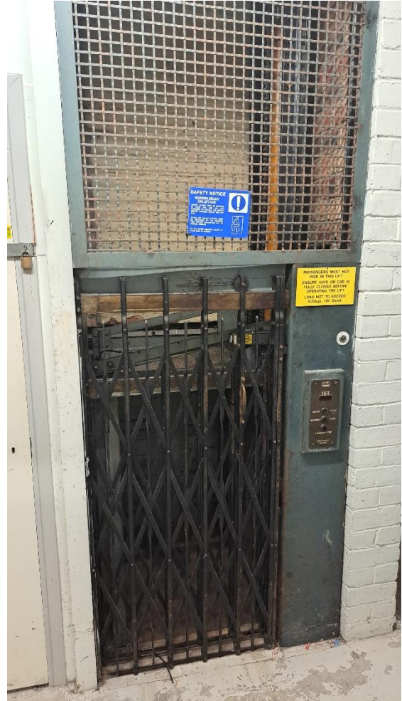
Figure 4 Cargo lift, basement level
