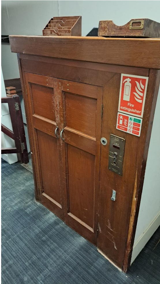
Figure 5 Cargo lift, ground floor level
