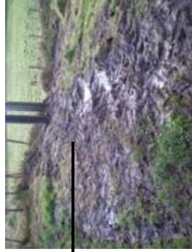
Outward face and Flood crest (heavy poaching)
