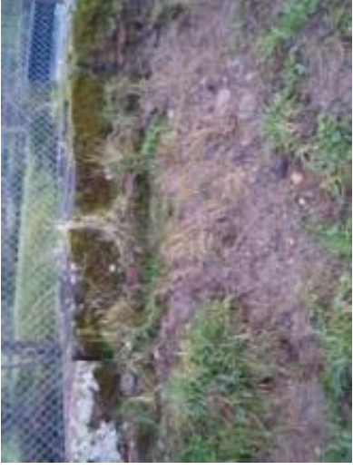
Heavily eroded outward face
