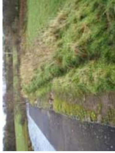
Heavily overgrown flood crest
