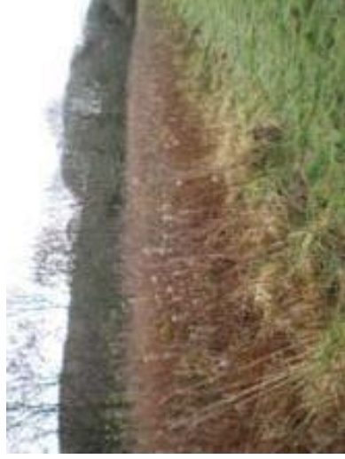
Invasive vegetation on outward face
