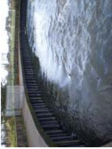
Sheet pile FI showing minor distortion But flood wall well protected by concrete berm
