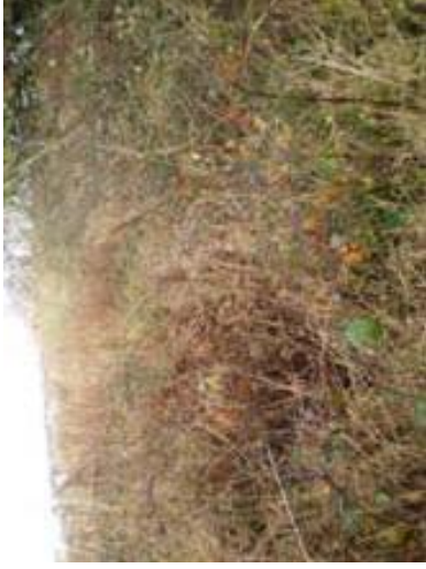
Invasive vegetation on whole embankment
