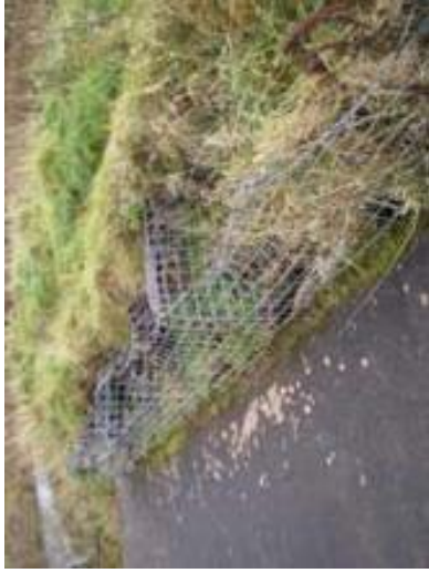
D/S gabion baskets in failed condition
