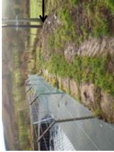
Flood crest Upstream (rutting)
