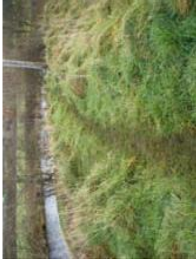
Crest heavily vegetated with rutting
