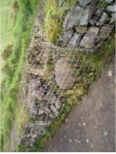
Gabions in Very Poor condition (Grade 5)
