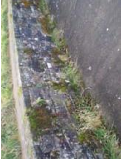
Minor grass growth in masonry wall joints
