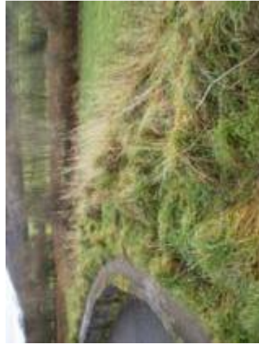
Heavily overgrown Flood crest
