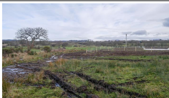
8. View of SUDS feature which serves Phase 1
