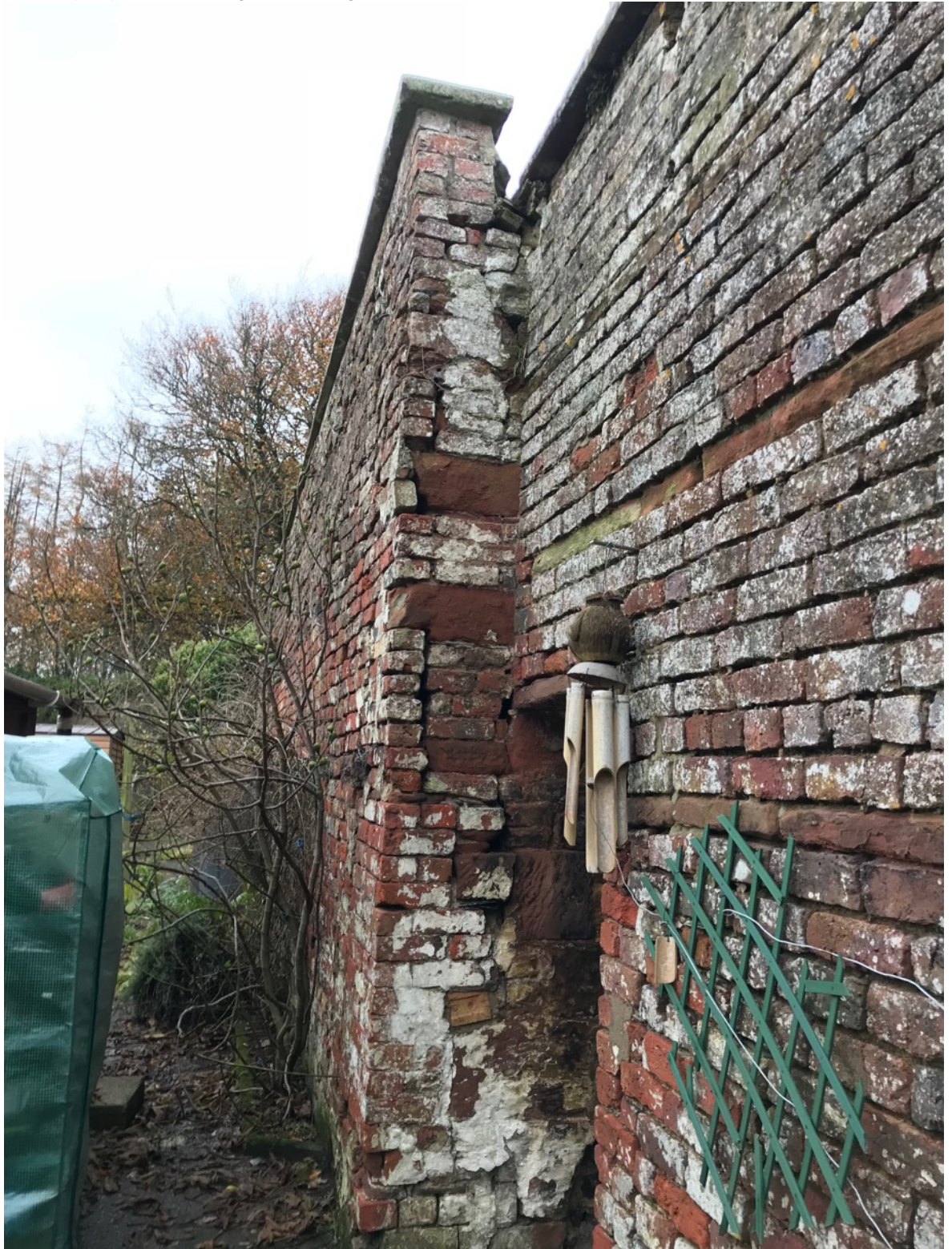
Photograph 10. Gaps within perimeter wall
