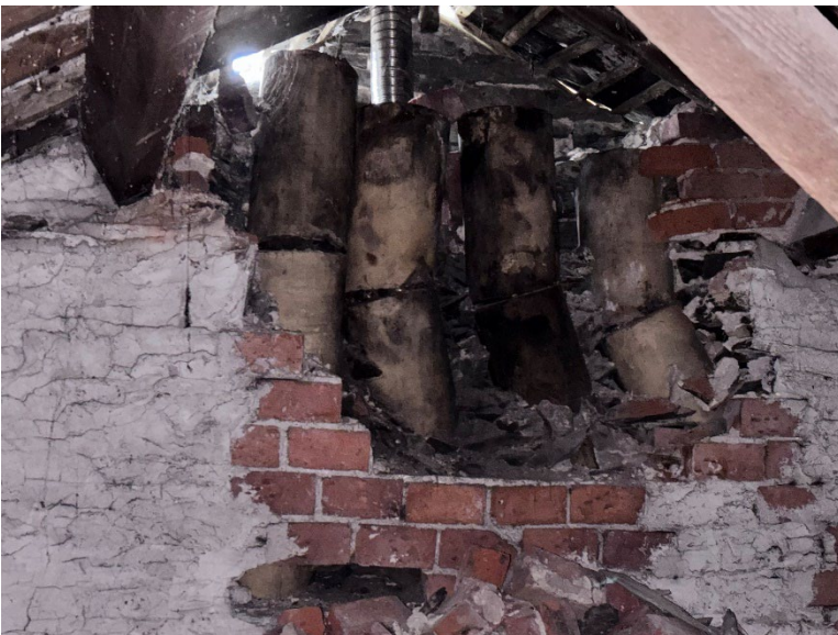
The gable walls has collapsed into the roof void and is unstable
