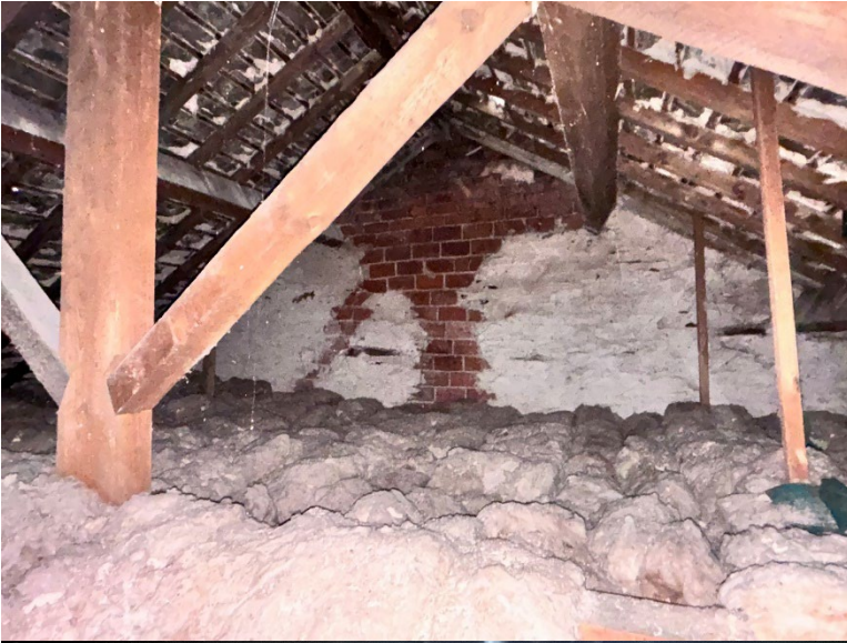
The roof void is open and light due to missing slates
