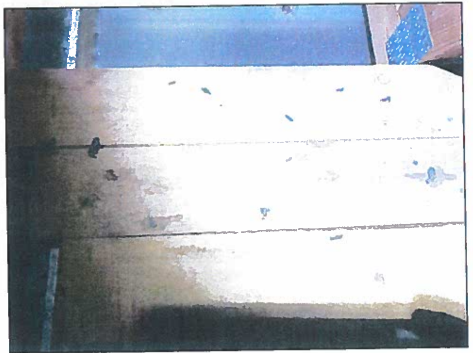
Figure 5: Showing rat droppings within the roof void.
