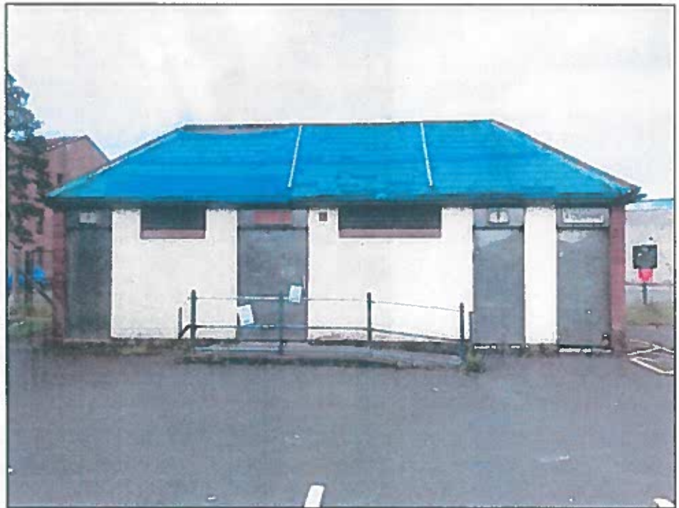
Figure 3: Showing the eastern elevation of Chapel Street Toilets with debris netting attached to the eastern pitch of the hipped roof to prevent broken tiles falling off.
