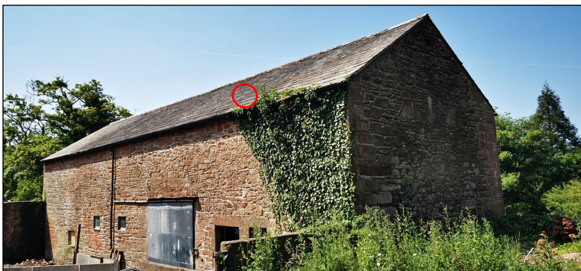
Plate 6 – showing Brandt's bat roost, used by three bats located under the roof slates within the eastern pitch of the roof.
