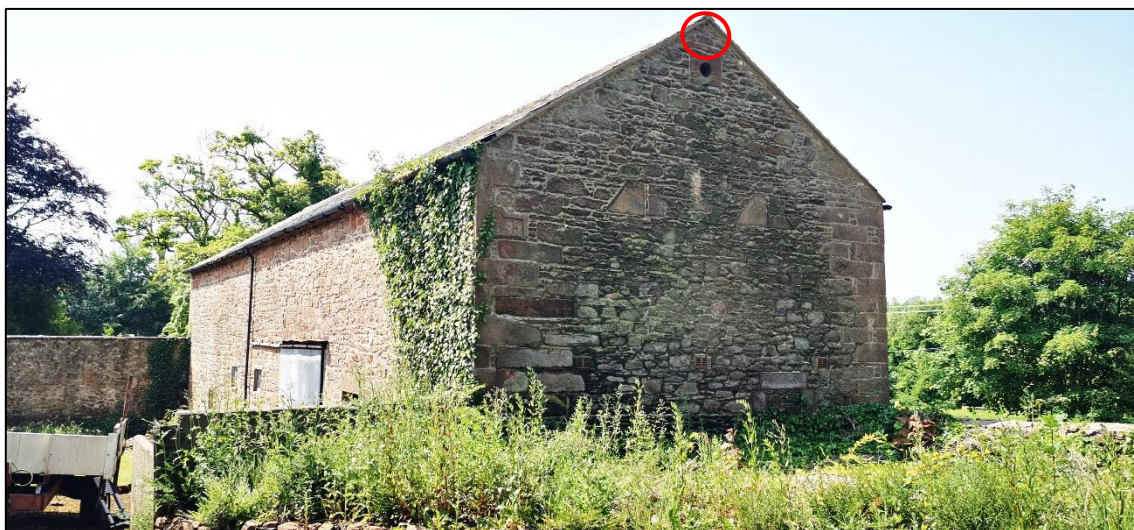
Plate 5 – showing soprano pipistrelle bat roost, used by a single bat located under the apex ridge tile of the northern barn gable.
