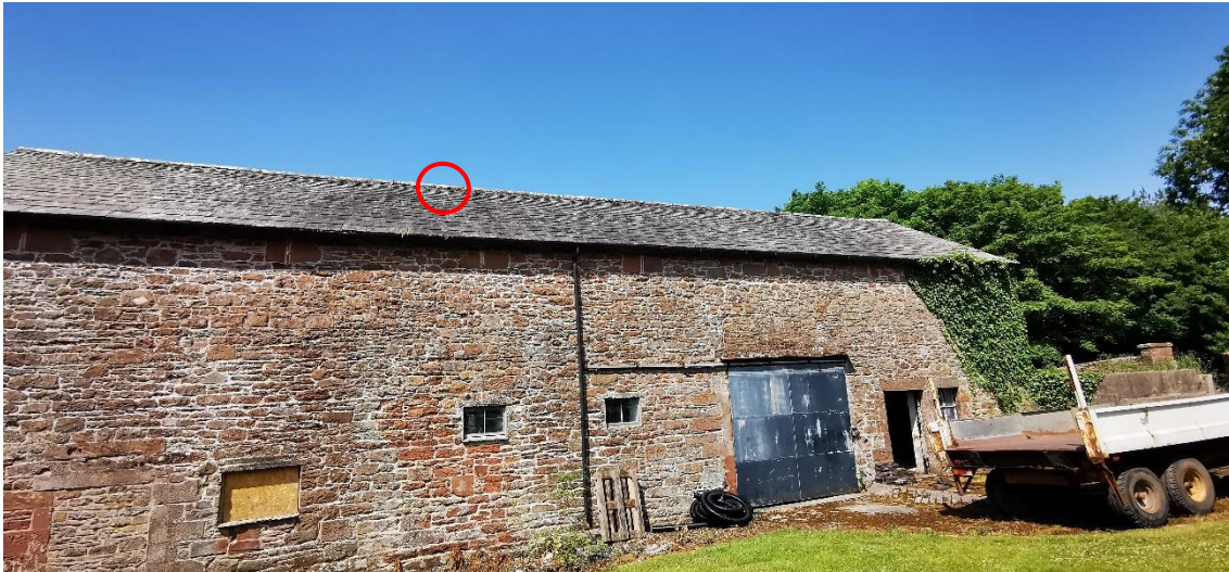
Plate 4 – showing Brandt’s bat roost, used by a single bat located under the roof slates within the eastern pitch of the roof.
