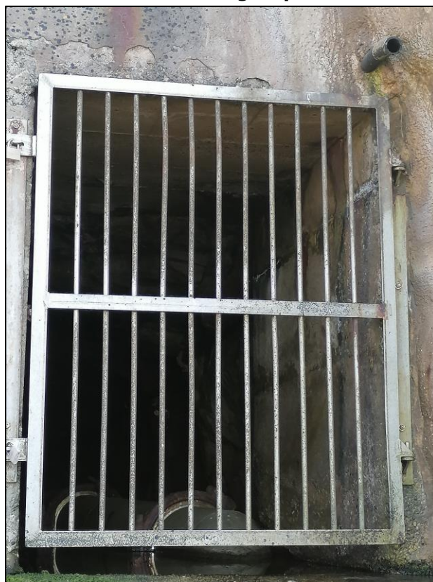
Photo 4 – Northern Discharge Pipe – Sea Outfall (II)
