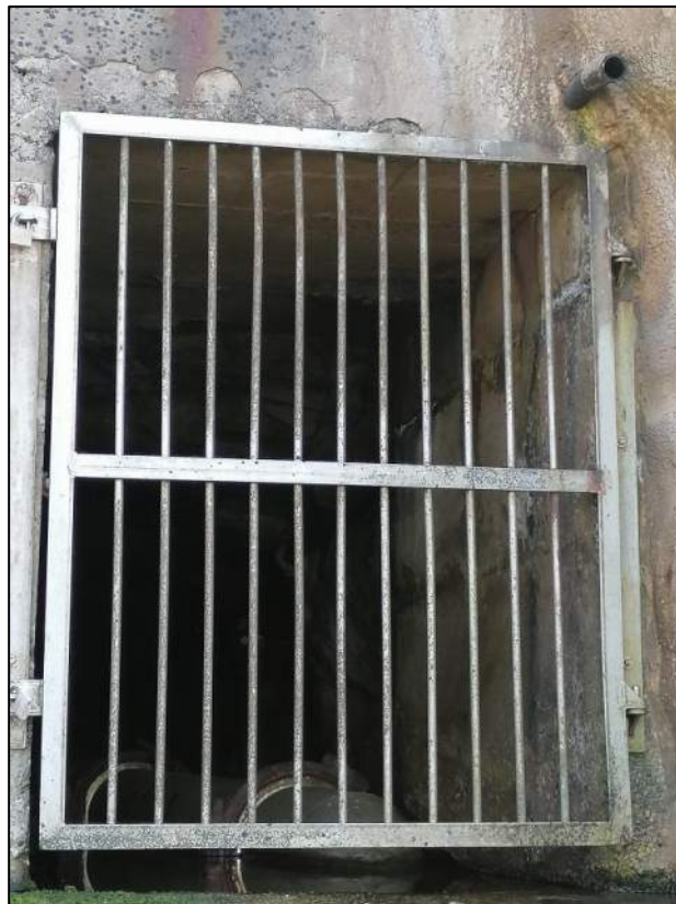
Photo 4 – Northern Discharge Pipe – Sea Outfall (II)
