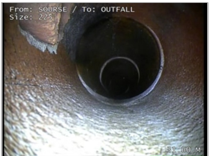
Connection other than junction at 9 o'clock, diameter 100mm
