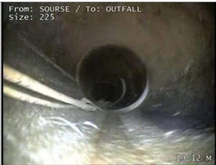
Roots tap at joint
