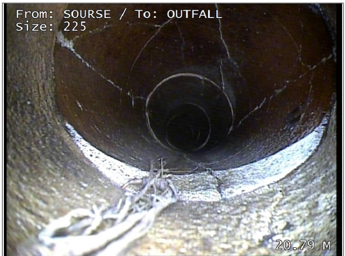
Fracture multiple from 9 to 3 o'clock
