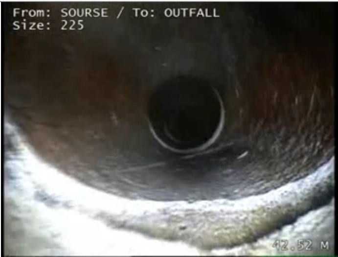
Joint displaced 10mm
