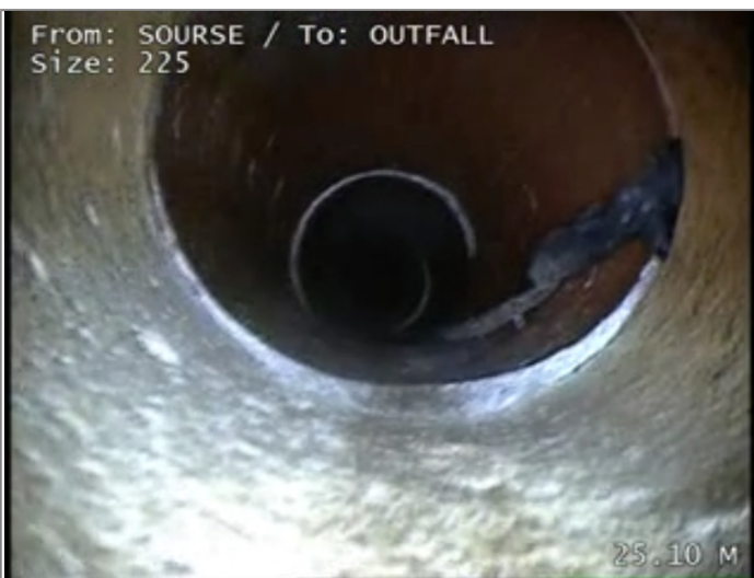
Roots tap at joint
