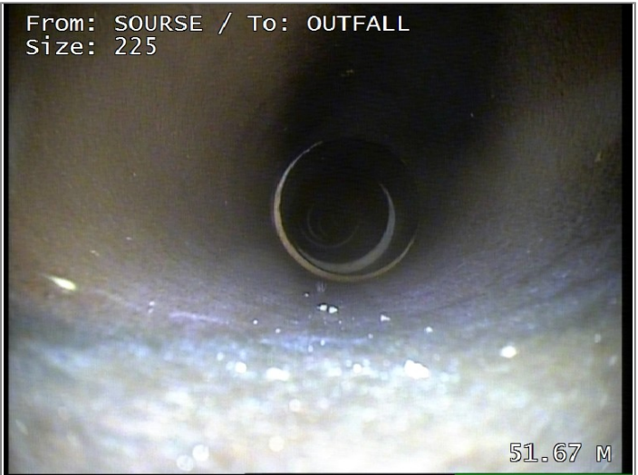
Finish node type, major connection without manhole, reference CCTV Has gone past site boundary
