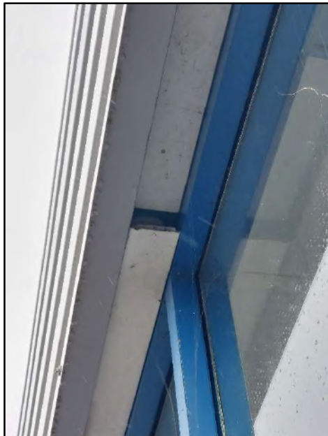
Photograph 7: Dropped section of material on south elevation of building reference A.
