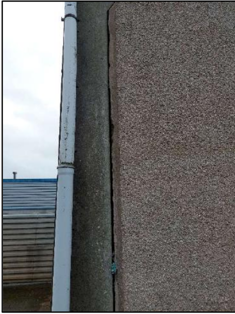
Photograph 11: Example of gap between supports and walls.
