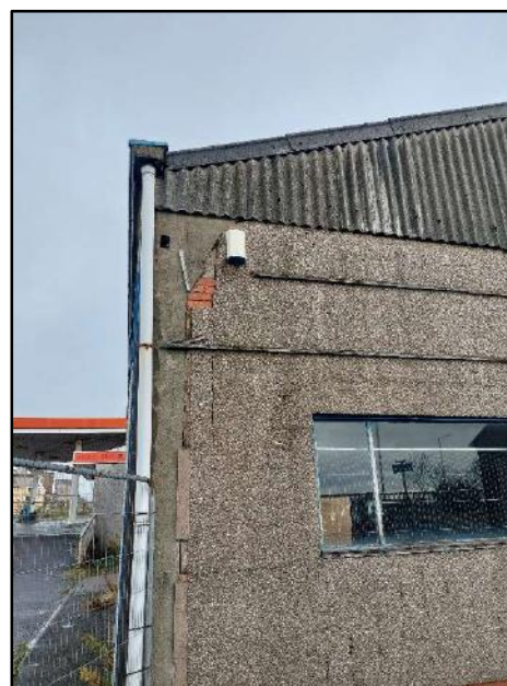
Photograph 10: Missing render, hole and cracks all providing potential for roosting bats.
